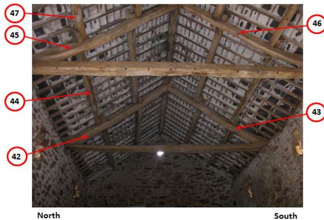
Figure 10e: Annotated photograph of the Garage barn to locate sampled timbers (photograph Robert Howard)
