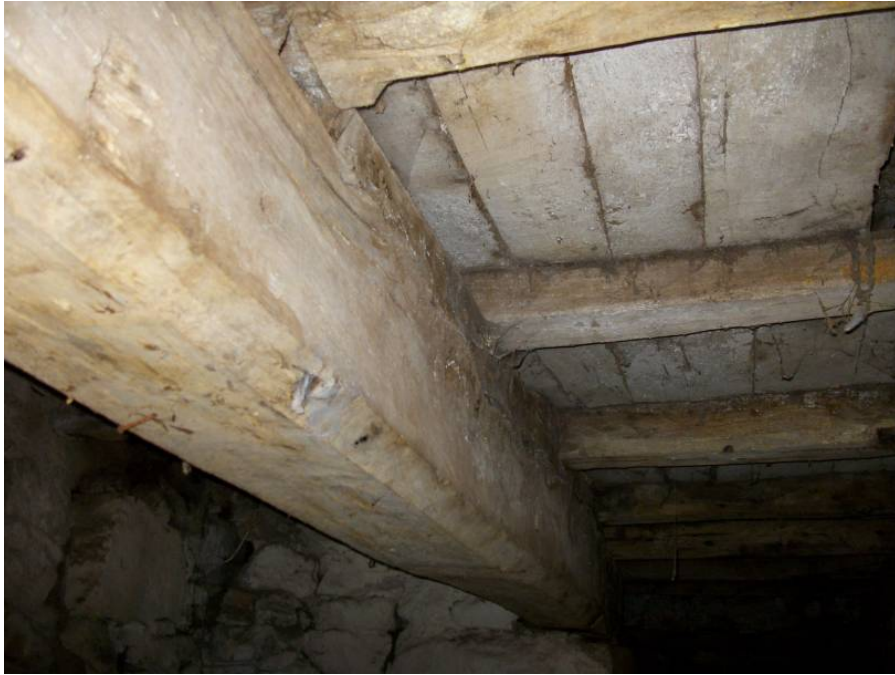
Figure 5d: View of bressummer and common joists to floor of room 2 (photograph Robert Howard)
