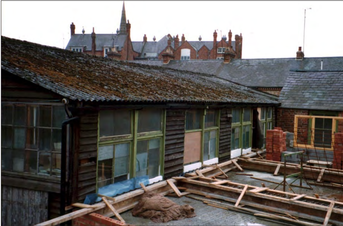
Fig. 5.1. NFF Banbury, former timber-framed factory building in use as coffin store, 1990 (R. Kinchin-Smith).
