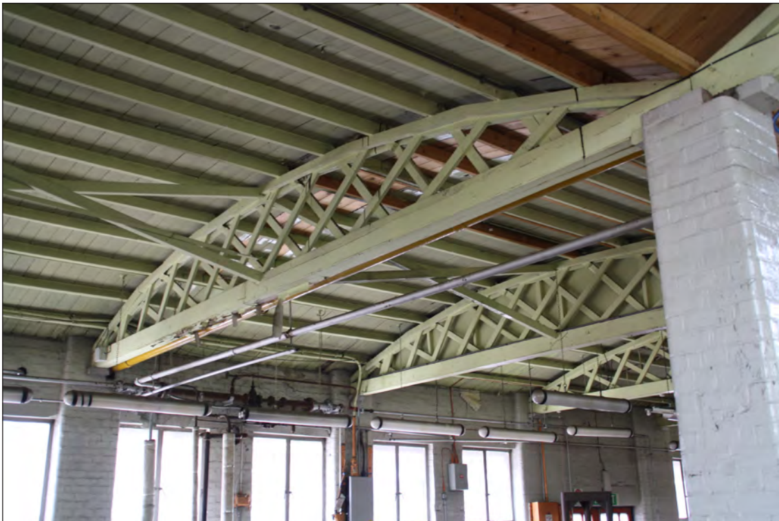
Fig. 3.3. NPF Birtley, surviving Belfast Truss roof in the former canteen building (W Cocroft).
