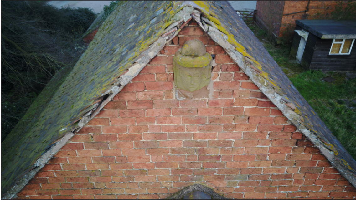
Figure 23: The ex situ carved corbel on the west gable of the building to the north of the gatehouse (© Mark Furniss, reproduced with permission)
