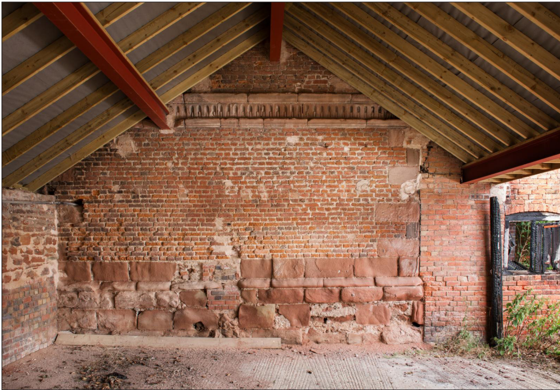
Figure 12: The south elevation with the best-preserved section of the fluted frieze (DP220869)
