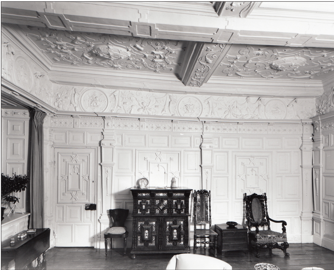
Figure 26: The plasterwork in the drawing room at Benthall Hall, Shropshire; photographed in 1995 (Historic England Archive, BF94928)
