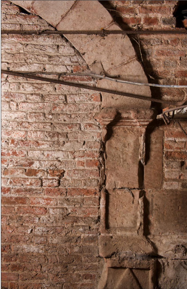
Figure 14: The north jamb of the arch in the east elevation with a moulded impost and a recessed panel above a raised lozenge (DP220872)
