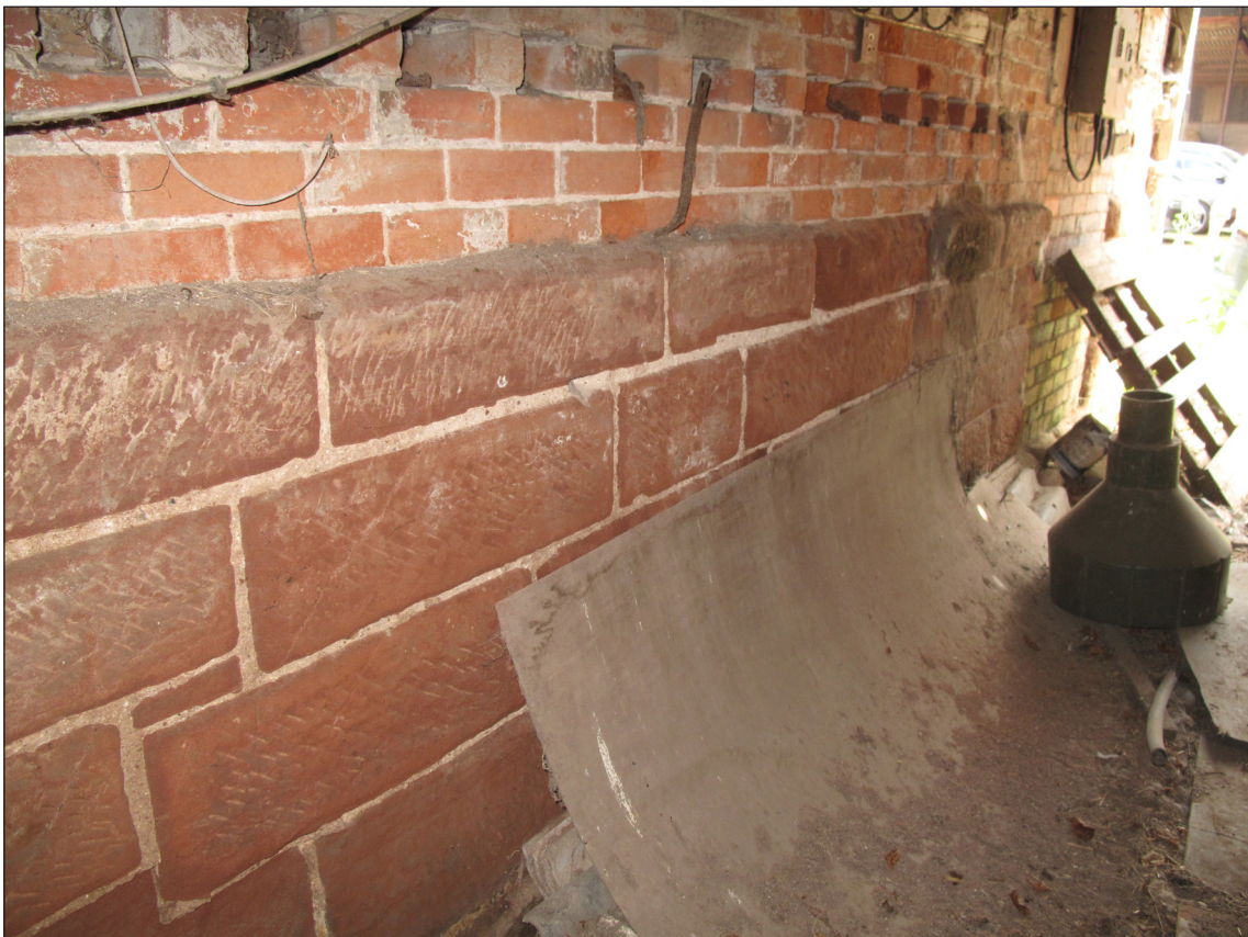
Figure 24: The sandstone base on the interior of the building attached to the east of the gatehouse (Rebecca Lane)
