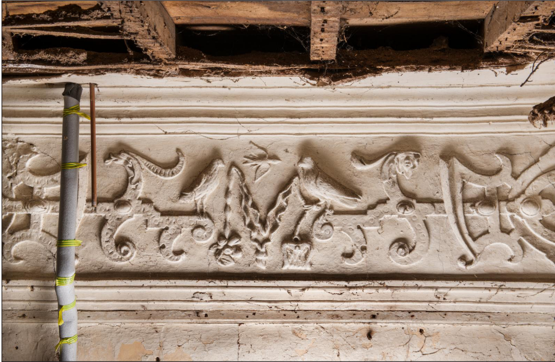
Figure 31: Detail of the frieze on the north wall of the gatehouse's first-floor south room (DP220820)
