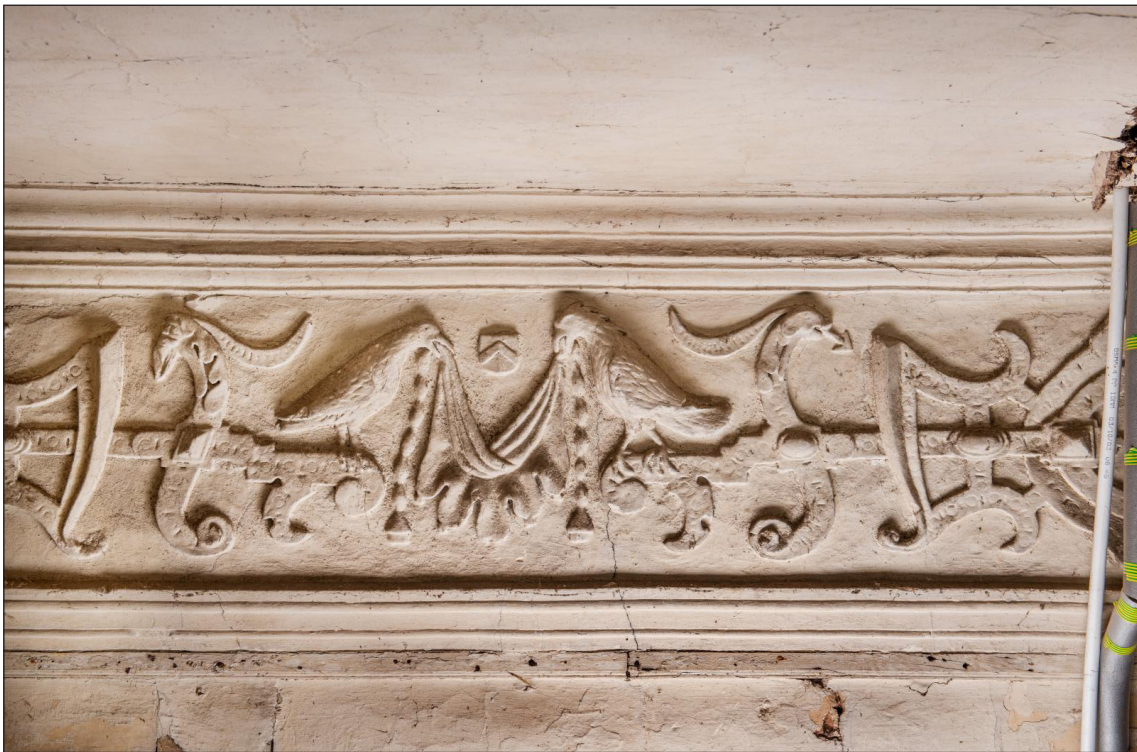
Figure 30: Detail of the frieze on the north wall of the gatehouse's first-floor south room (DP220818)
