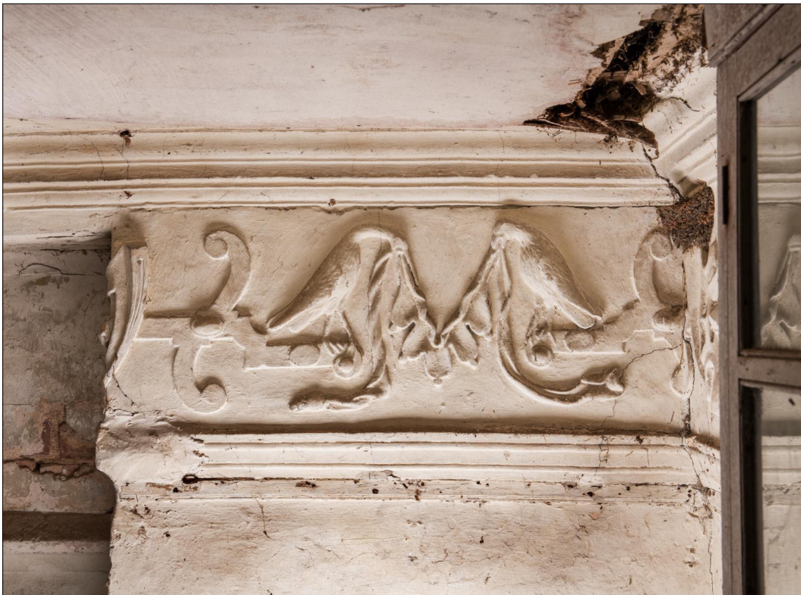
Figure 32: Detail of the frieze on the east wall of the gatehouse's first-floor south room (DP220825)
