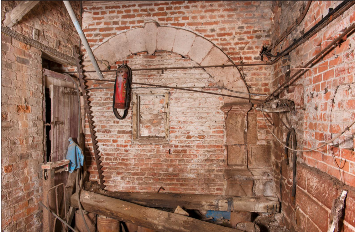
Figure 22: The blocked arch in the east elevation with the later timber window frame (DP220876)
