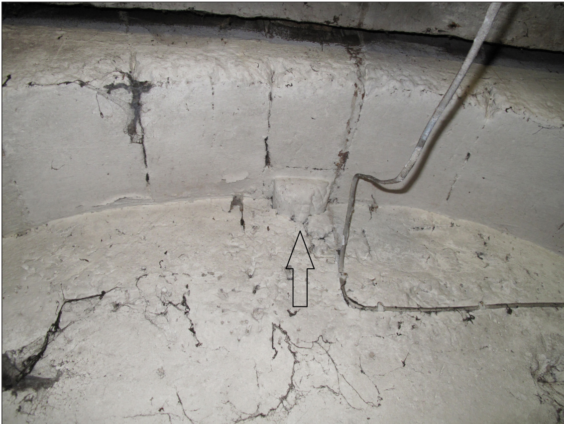
Figure 15: The blocked east arch seen from inside with the keystone pendant (indicated by an arrow) (Rebecca Lane)
