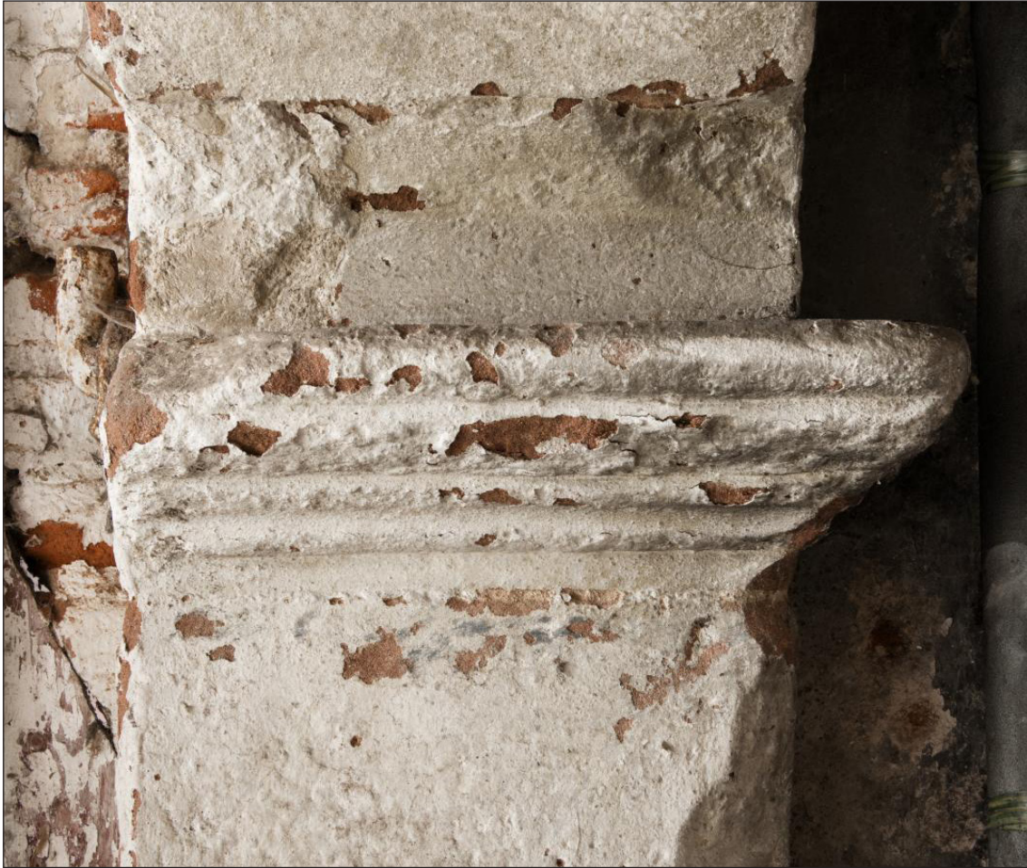
Figure 16: The northern jamb of the internal arch seen from the south, showing the historic pintle and the lack of an impost moulding, both on the west (left) face (DP220867)
