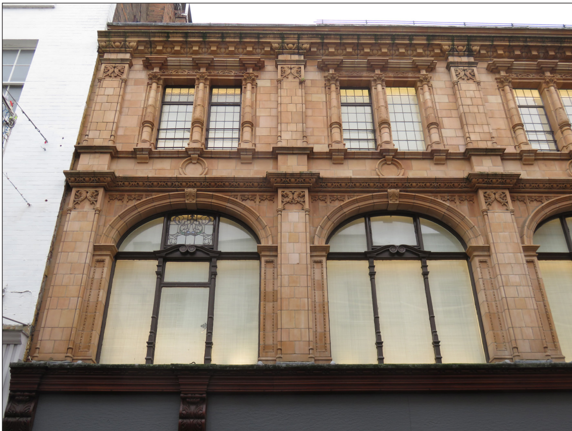
Fig 20. Detail of Pelham Street elevation, with decorative terracotta and glazing. (© Historic England, K. Morrison)
