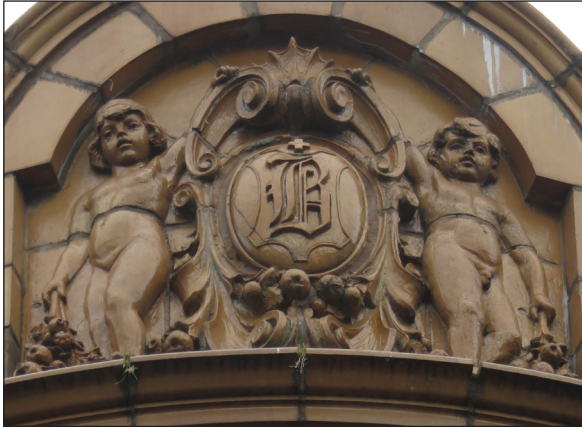
Fig 22. Detail of terracotta decoration with 'B' monogram on south-west corner of Boots' building. (© Historic England, K. Morrison)
