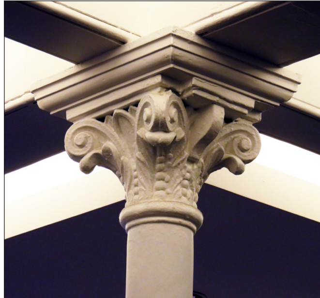
Fig 4. A cast-iron capital surviving from the first-floor gallery of Boots' 1892 shop. The ground-floor capitals (shown in figs 3 and 19) are of slightly different design. (© Historic England, K. Morrison)
