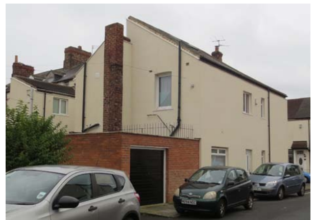
Figure 19 Note large thermal bridge
