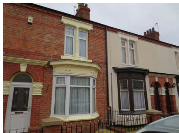
Figure 21 Large untreated areas to right-hand property
