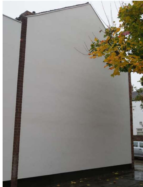
Figure 23 Exposed brickwork creating thermal bridge risk
