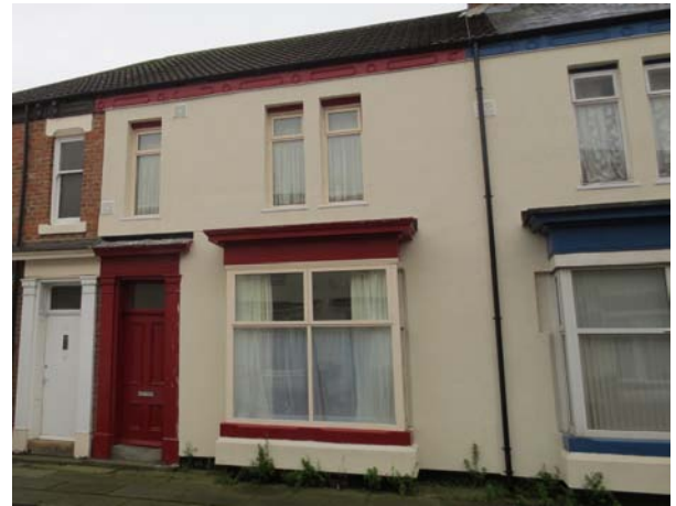
Figure 13 Untreated large window and door
