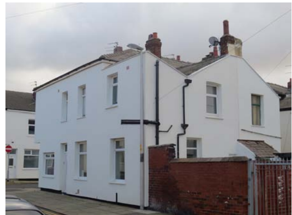
Figure 85 Lamppost obstructing pipework removal
