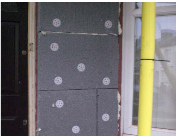
Figure 62 Poor insulation jointing 69
