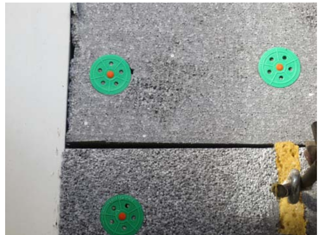
Figure 77 Poor insulation jointing
