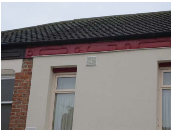
Figure 14 Thermal bridging at eaves
