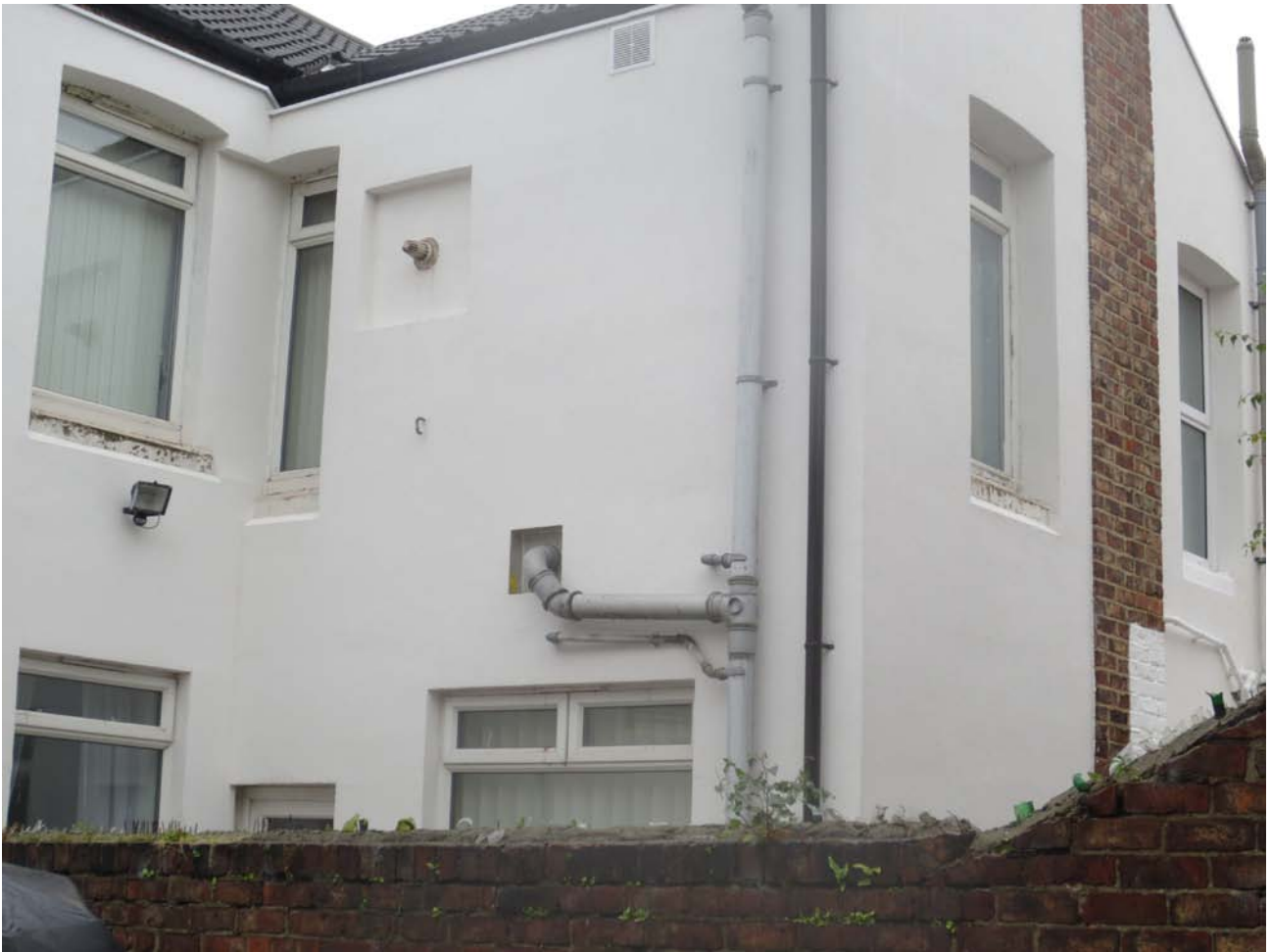
Figure 44 Note the many thermal bridges, in particular the corner bridge between the two upper windows
