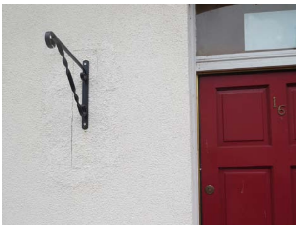
Figure 30 Note cracks in finish around plant holder
