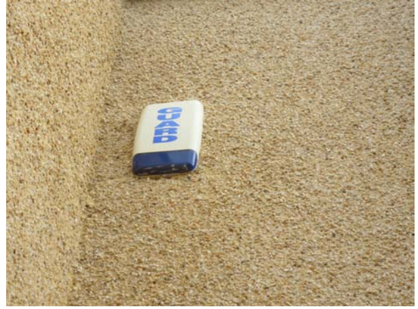
Figure 59 Alarm not removed prior to insulation
