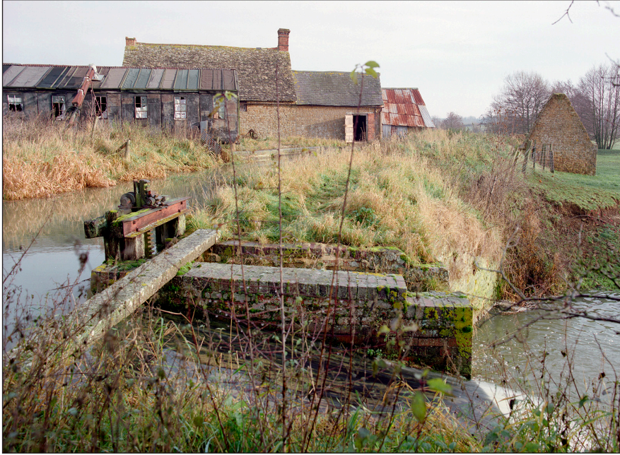
Figure 13 – A sluice gate and spillway at Little Barford Mill, Oxfordshire (Peter Williams © Historic England)
