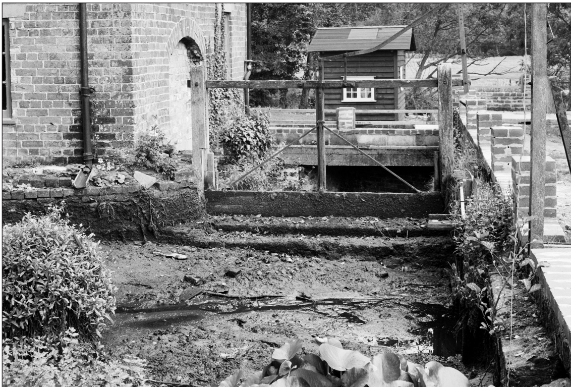
Figure 23 – The head race and sluice of a mill, silting up and filling with debris, probably Southover, Frampton, West Dorset but could also be Southover, Tolpuddle, West Dorset (1963 Joseph Addison © Historic England aa043572)
