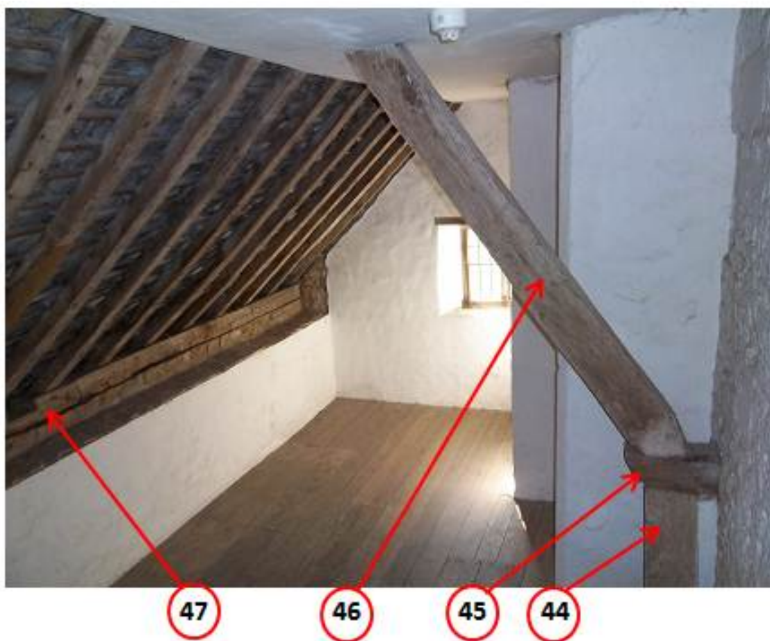
Figure 10: View of the west-end roof above the small chamber to locate sampled timbers (photograph Robert Howard)
