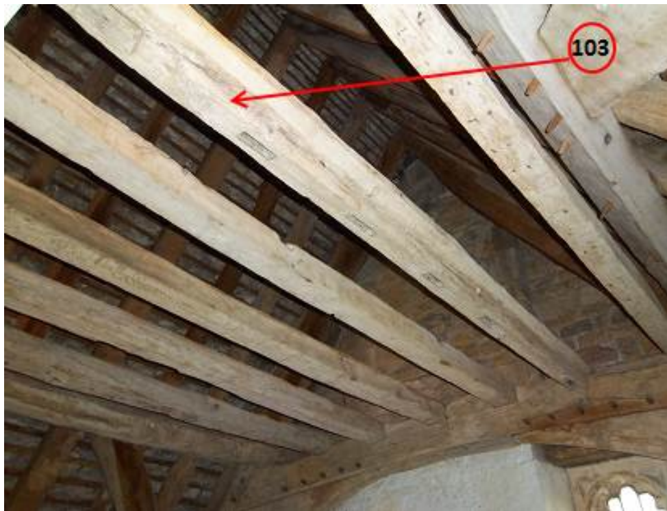
Figure 18a/b: Views of the partition wall and ceiling at the west end of the roof above the Great Chamber/Presence Chamber to help locate sampled timbers (photographs Robert Howard)
