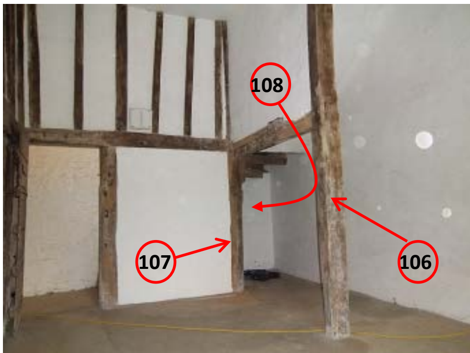
Figure 19a/b: Views of the Bedeswoman room 2 partition walls and stair framing to help locate sampled timbers (photographs Robert Howard)
