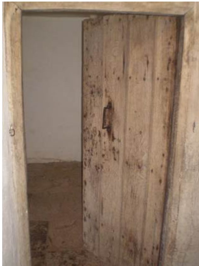
Figure 4a/b: Examples of the wooden doors to the Chapel/Bedeswoman rooms landing (L) and Great Chamber (R) (top) and to Bedesman room 5 (bottom) (photographs Robert Howard)
