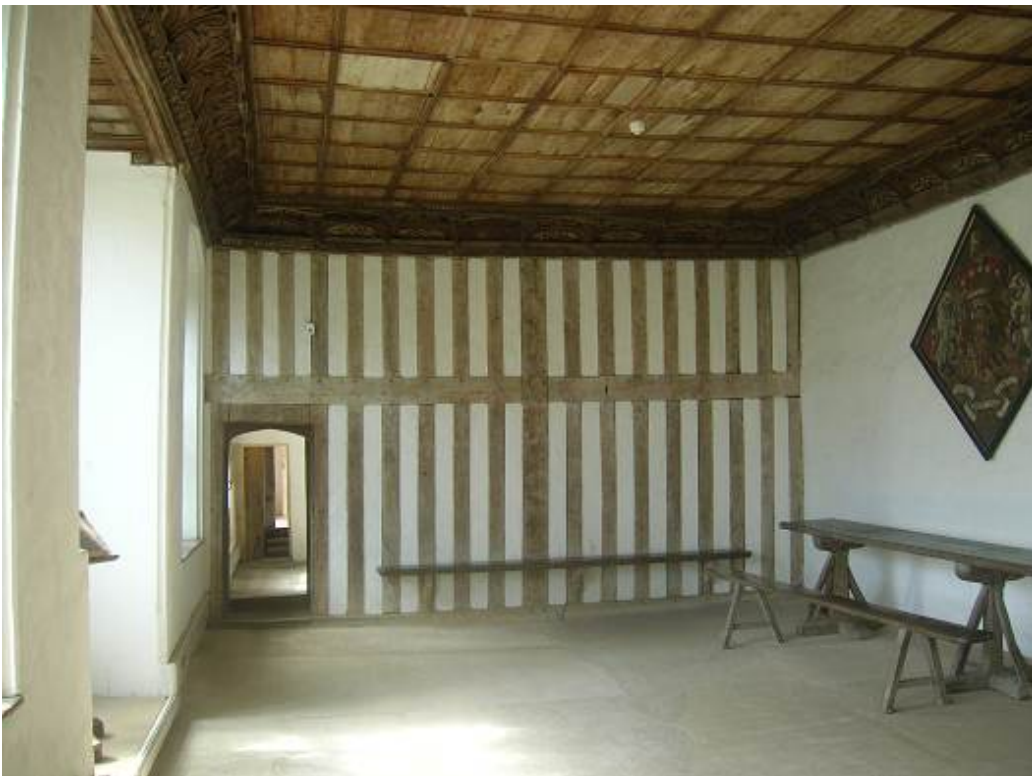
Figure 2a/b: The Pentice to the north wall of the Bede House (top) and the Great Chamber, with Presence Chamber and small chamber beyond (bottom) (photographs Robert Howard)
