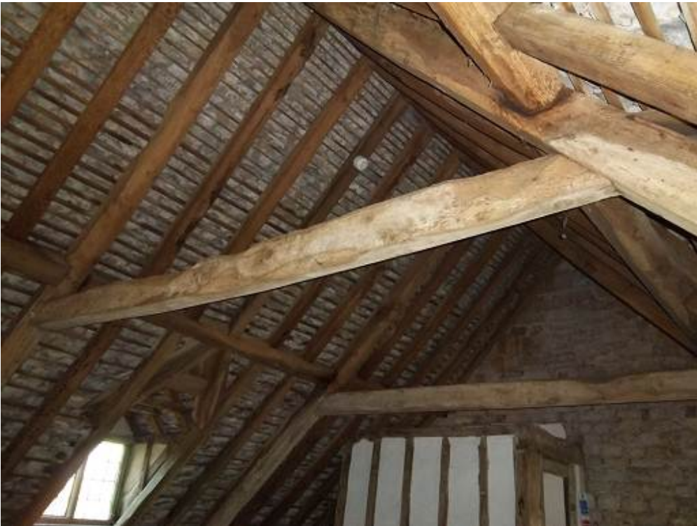
Figure 3a/b: The roof above the Great Chamber looking east (top) and the roof at the east end of the Bede House (bottom) (photographs Robert Howard)
