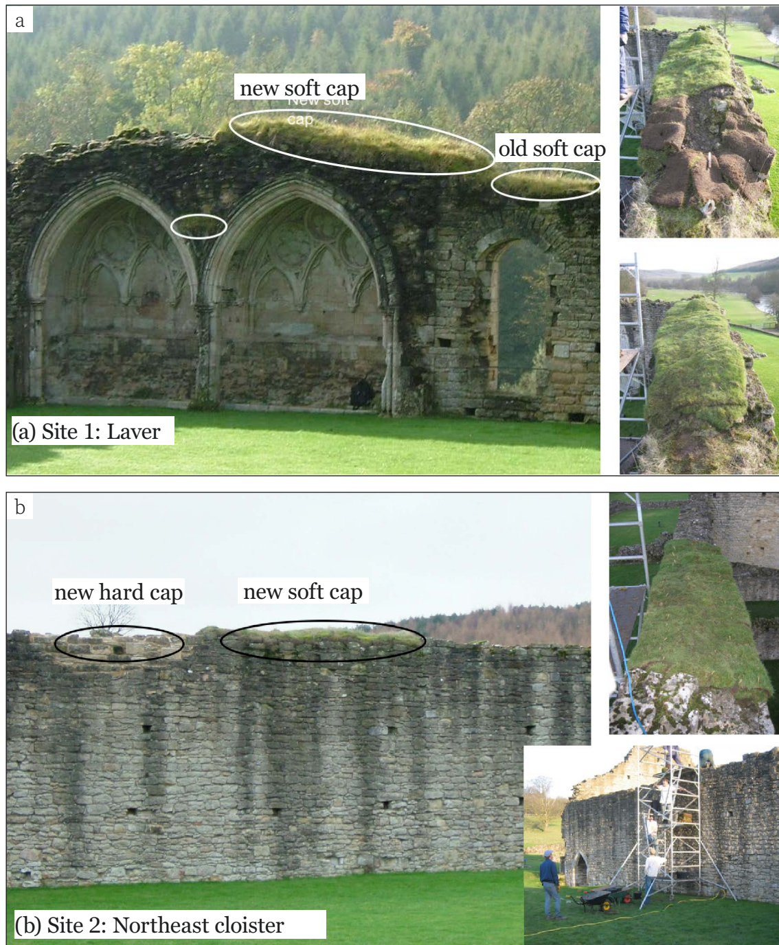
Figure 2.5 Location of newly installed soft capping at Kirkham Priory. (a) Site 1, the laver alcove, where a 5 m long (1.3 m wide) section of 10 cm thick soft capping (using local turf and soil containing regolith) was installed on the top of the wall (see insets of installation). A 30-cm (15-cm wide) section was also installed, at the top of the column between the arches (lower white circle). (b) Soft capping (3.9 m long, 50 cm wide 10 cm thick soft capping using local turf and soil with regolith) and hard capping (3.9 m, 50 cm wide using lime mortar and stone) on the north east cloister wall, at site 2. (all ©Heather Viles, University of Oxford)
