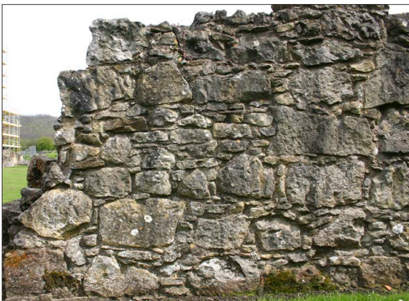
Figure 6.13 Cracking in the wall due to consolidation using cement mortars. © Chris Wood, Historic England
