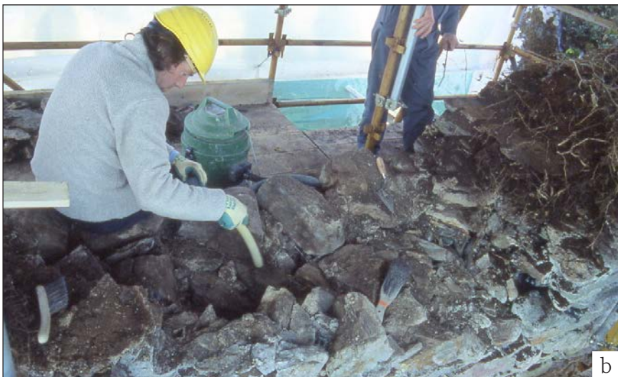
Figure 6.15 (a) Numbering and labelling the face work stones as they are removed from the wall, and (b) removal and cleaning of the core work. ©Colin Burns
