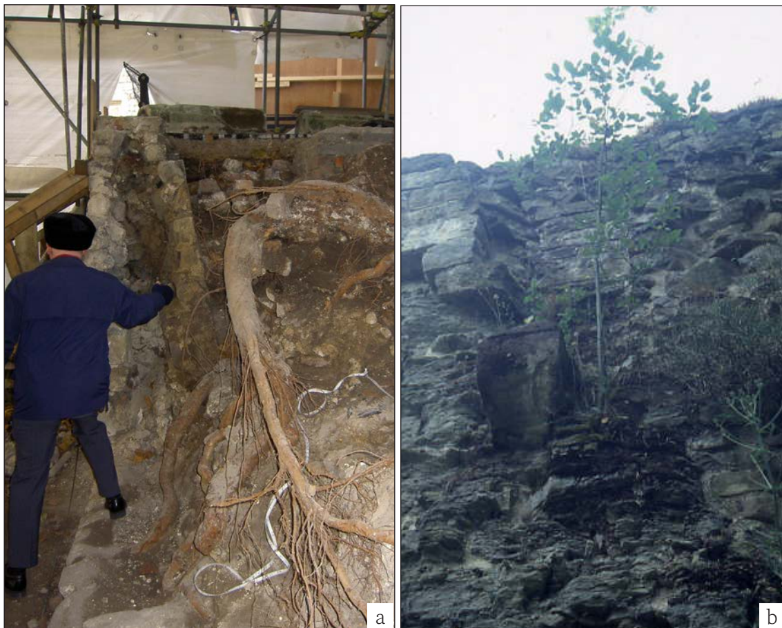
Figure 6.11 Damage to the moat wall at the Tower of London (a) caused by the secondary thickening of tree roots; and a tree growing on an uncapped ledge on a wall at Wigmore Castle (b). (both ©Alan Cathersides)
