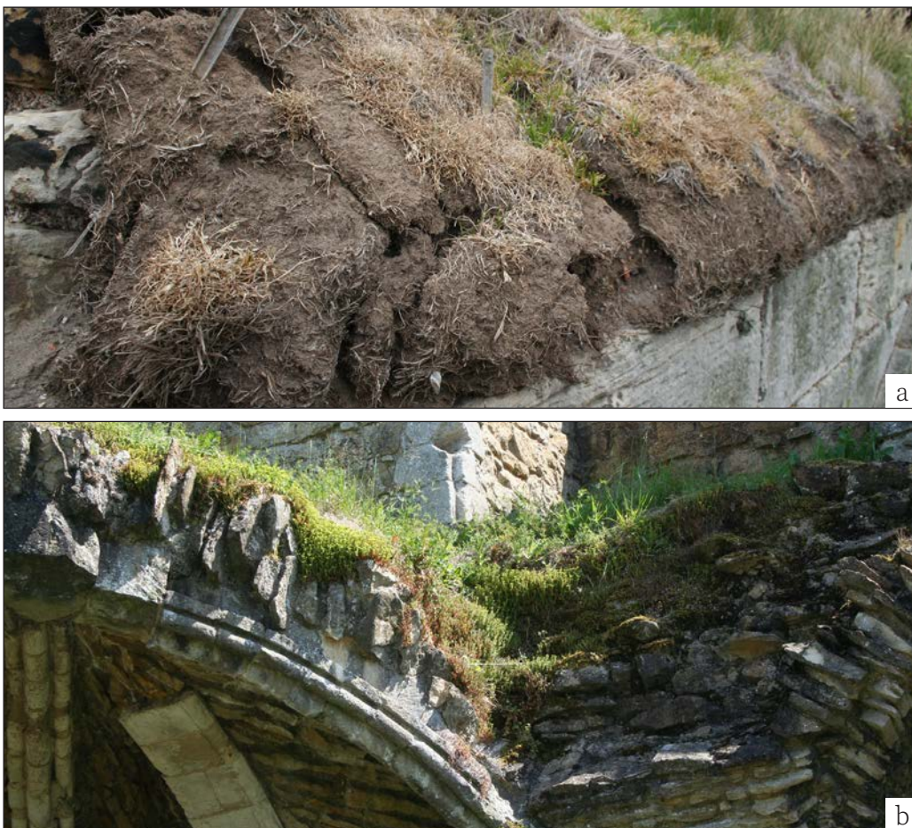
Figure 7.8 Soft capping in a highly exposed position at Whitby Abbey showing decay at the edges (a); and older soft capping at Kirkham Priory showing exuberant growth of sedum along the edges (b). (both ©Chris Wood, Historic England)
