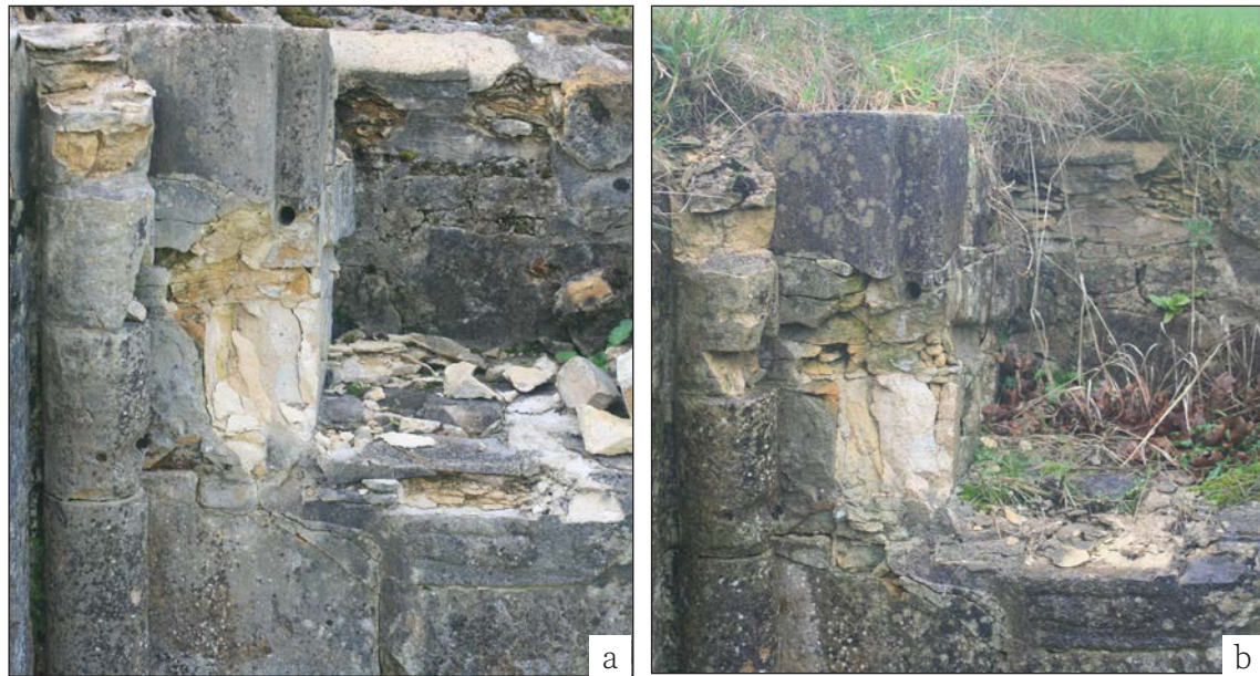
Figure 8.1 Deterioration in small sections of stonework which were not suitable for soft capping. (both ©Alan Cathersides)
