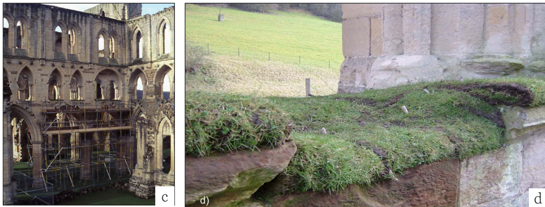
Figure 2.8 c, d The soft capping installed high at triforium level in the wall of the main abbey church nave at Rievaulx. (both ©Heather Viles, University of Oxford)
