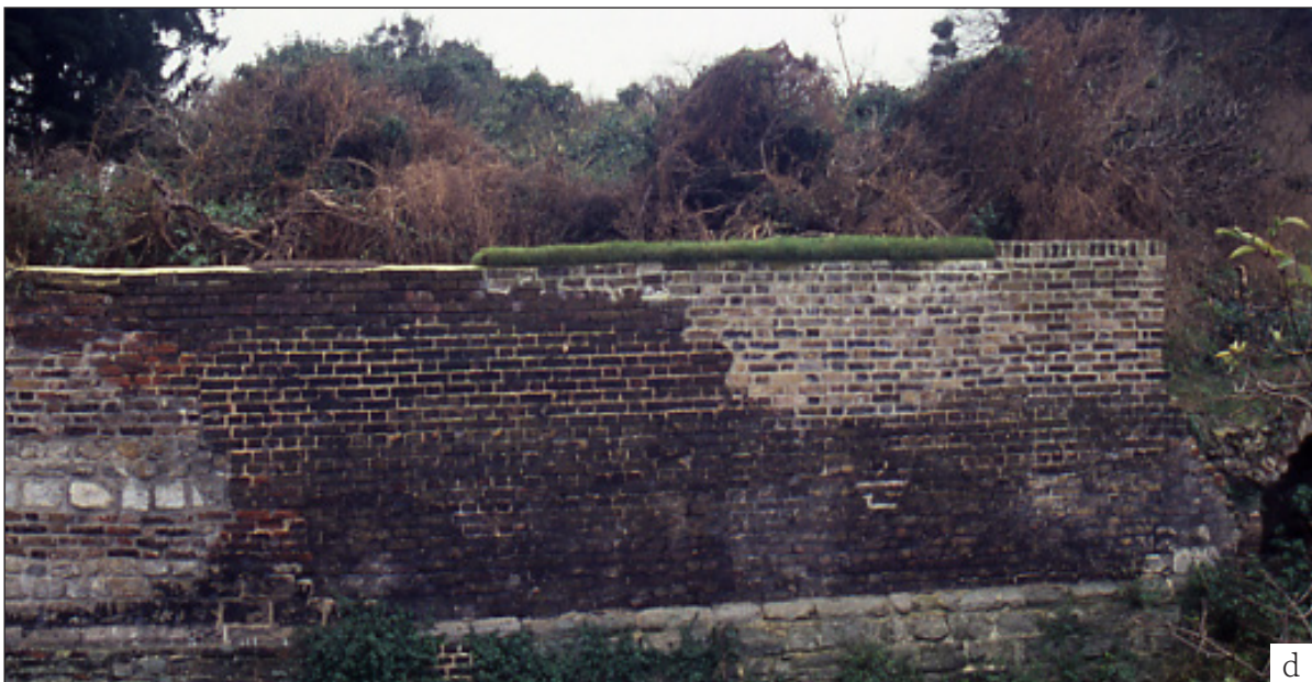
Figure 2.13 Soft capping work at Howbury Moated Site, (c) Site 1 and (d) site 2. (both ©Heather Viles, University of Oxford)
