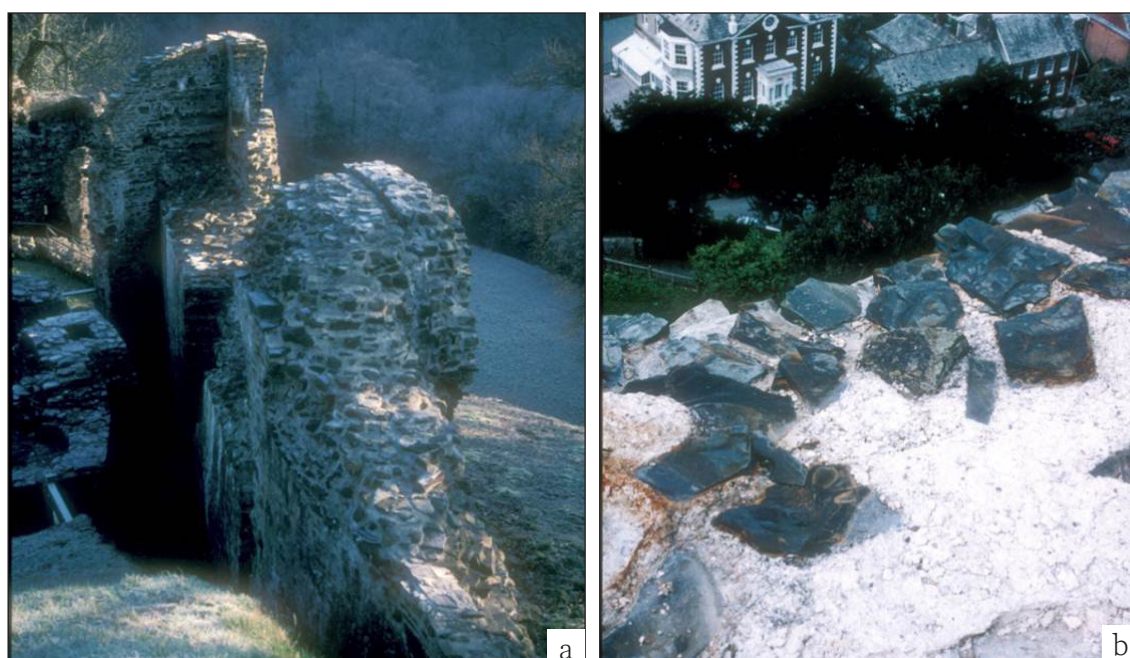
Figure 1.2 Frost damage at (a) Okehampton castle and (b) Launceston Castle. (both Chris Wood ©Historic England)
