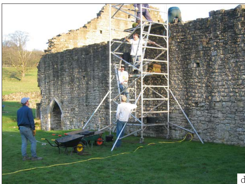
Figure 2.4 c, d Installation of soft capping on top of the laver alcove on the southwest side of the cloister (test location 1) and on the top of the northeast cloister wall (test location 2) at Kirkham Priory in February 2004. (both ©Heather Viles, University of Oxford)
