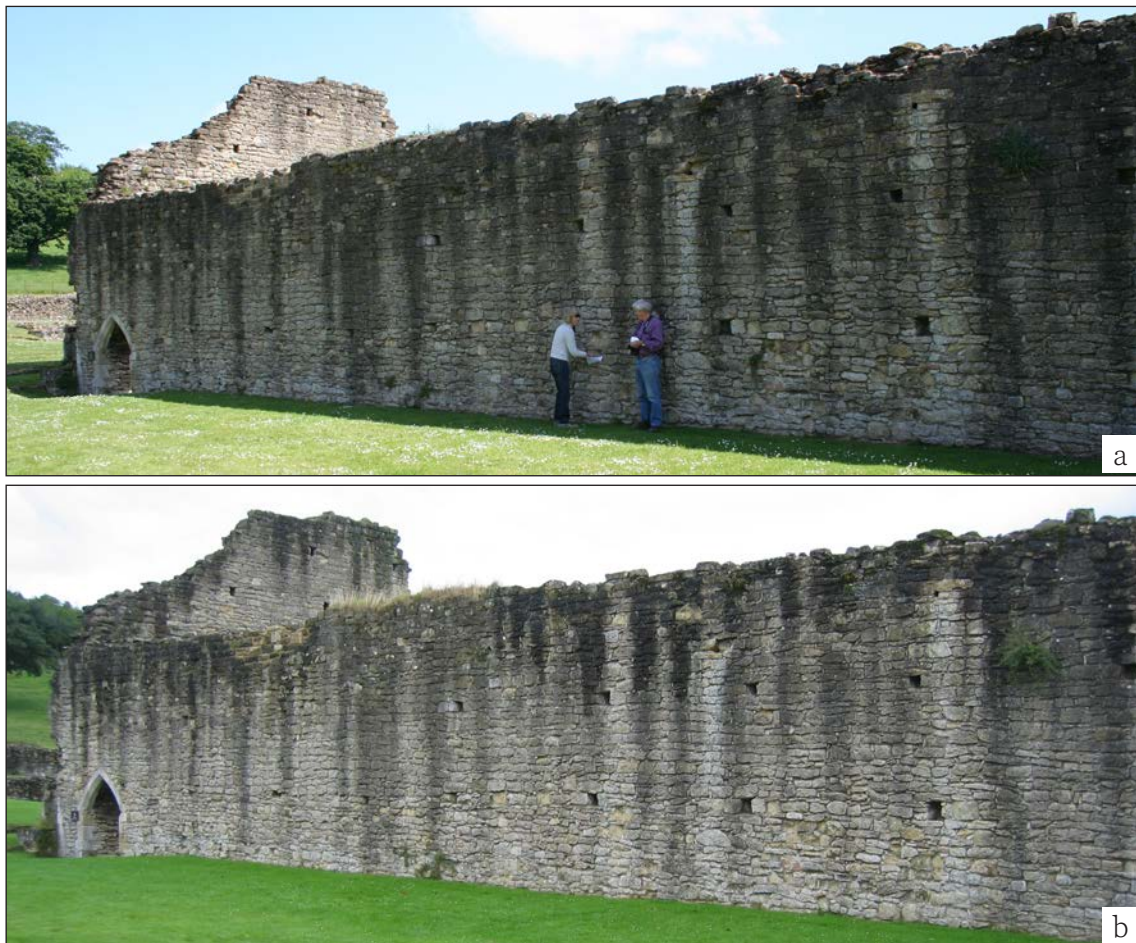
Figure 7.5 Streaking on the wall of the frater (refectory wall) (a) before and (b) 18 months after soft capping was installed. Streaking appears less noticeable after 18 months underneath the soft capped section (black line, image b, just after heavy rain), whilst there is no difference between the hard-capped section and the uncapped areas. (both ©Chris Wood, Historic England)
