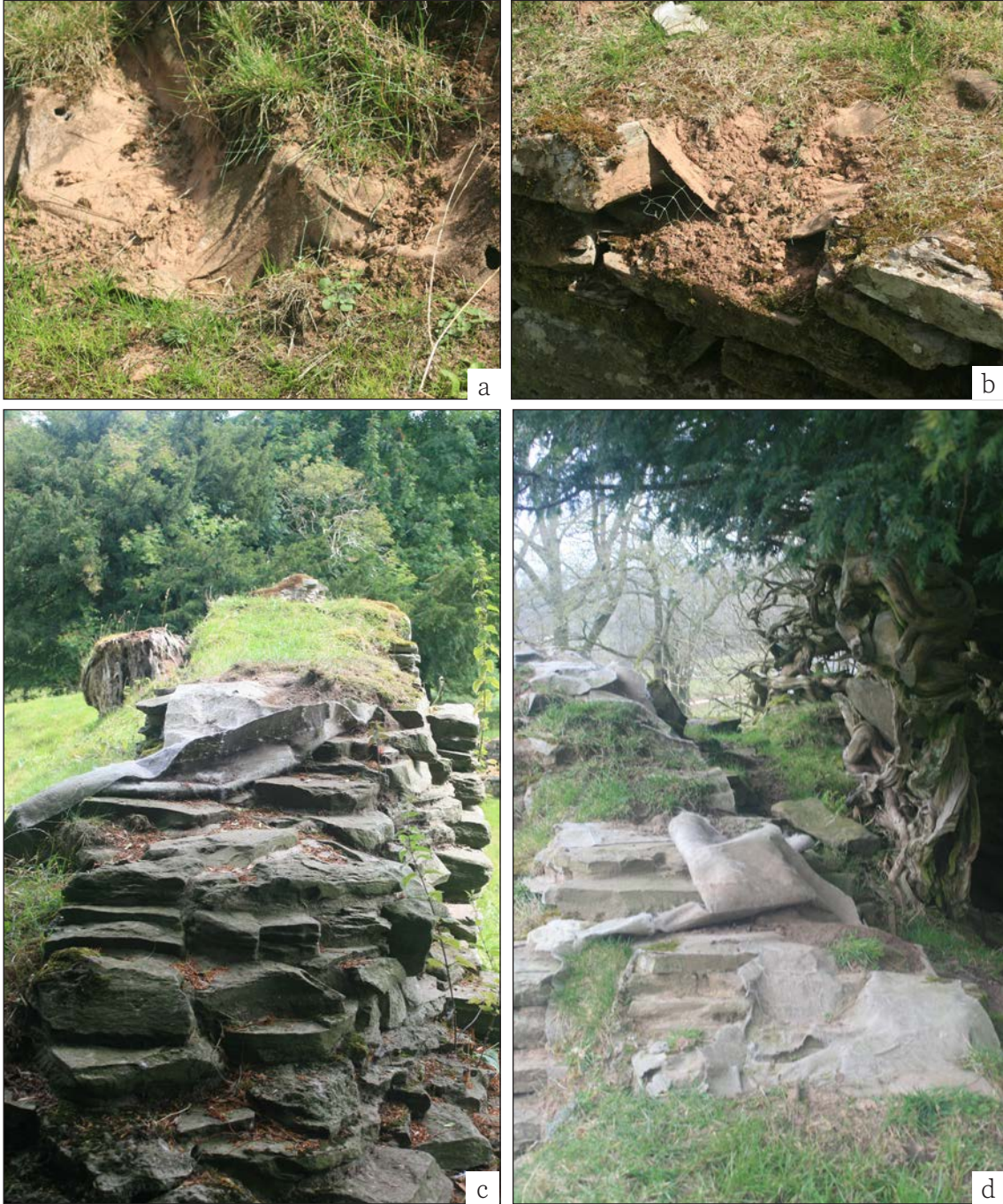
Figures 6.1 (a-d) showing the problems with using membranes on both even and uneven wall-heads. (all ©Alan Cathersides)
