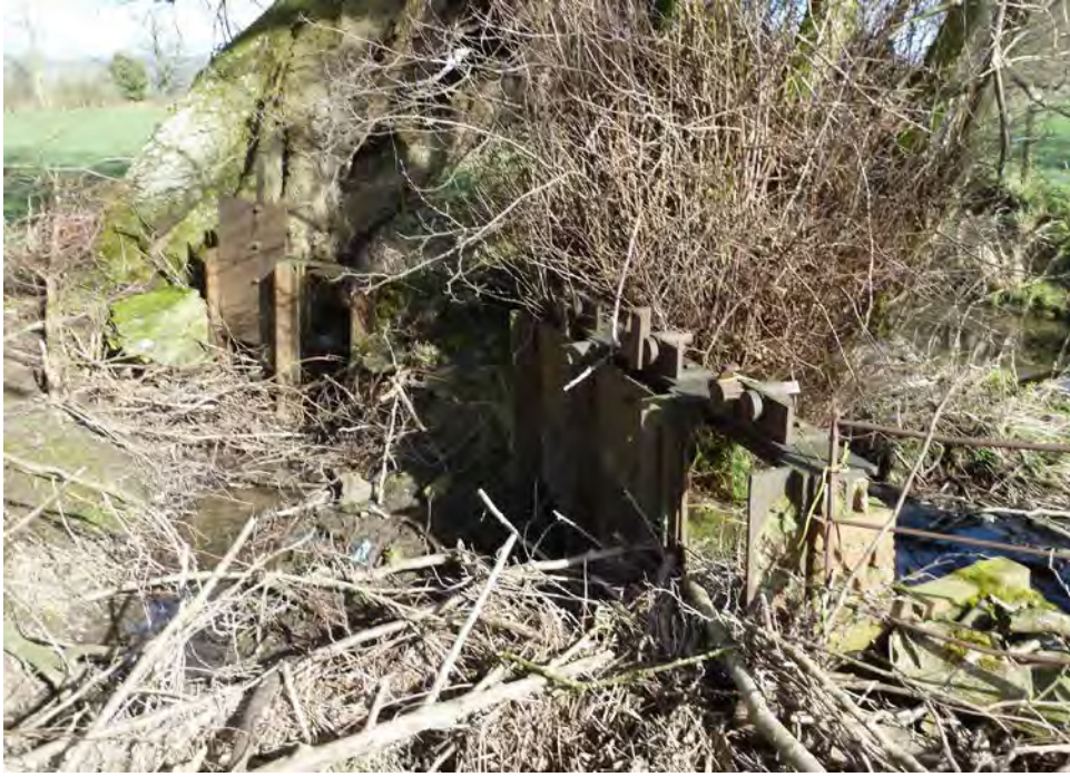
Fig. 10. New Mill, Pembridge: sluices controlling water for the mill, with a minor one for water meadow irrigation.
