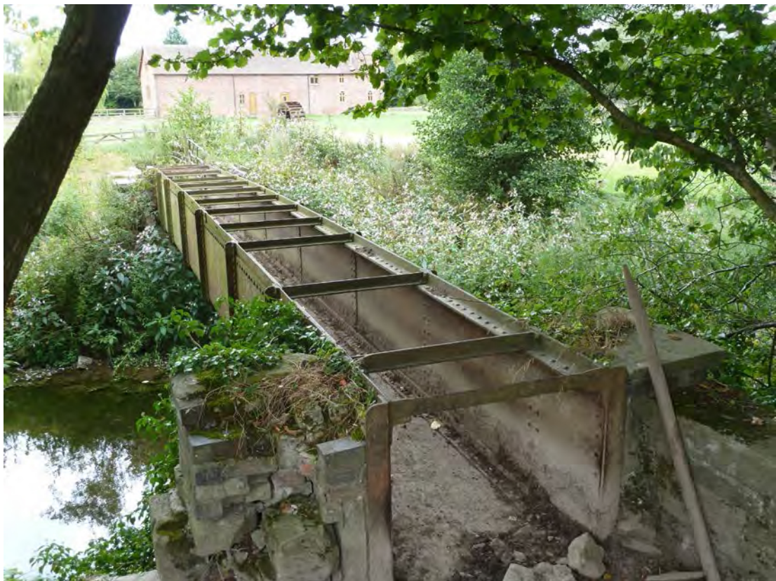
Fig. 29. Day House, Kingsland: the aqueduct across the River Lugg, with the farm mill and the waterwheel in the background.
