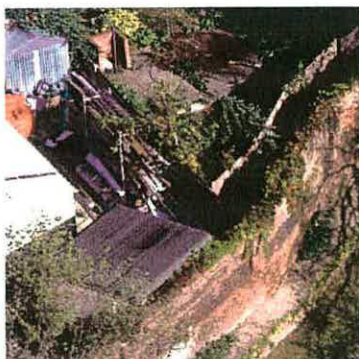
Fig. 12 - A section of the Mill Hill Park Estate boundary wall, viewed from Jerome Tower (English Heritage, 2004).
