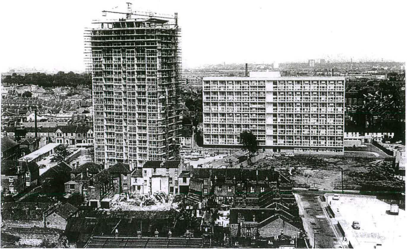
Fig. 60 - Barrie House, 100 flats in 21 storeys, under construction in 1967, with Barwick House, 99 flats and maisonettes in 13 storeys, built 1965-6, to the right, view from the roof of Jerome Tower with central London in the distance. Barrie House was demolished in 2001 (Ealing Local History Centre).
