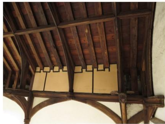
Temporary boards forming the south nave boxed-in area, viewed from the west end of the nave.
