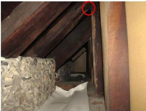
View inside the south nave boxed-in area. A mortise joint roost is circled in red.
