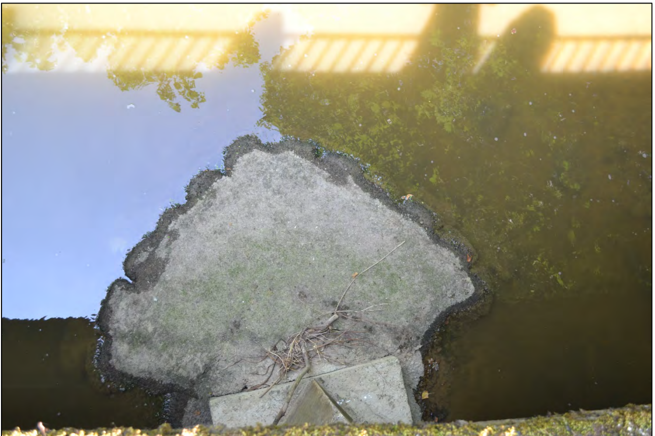
Plate 2: Modern bridge support apparently on much earlier pier, now covered in concrete and concrete bags, Dauntsey, River Avon (© Antony Firth/Fjodr)
