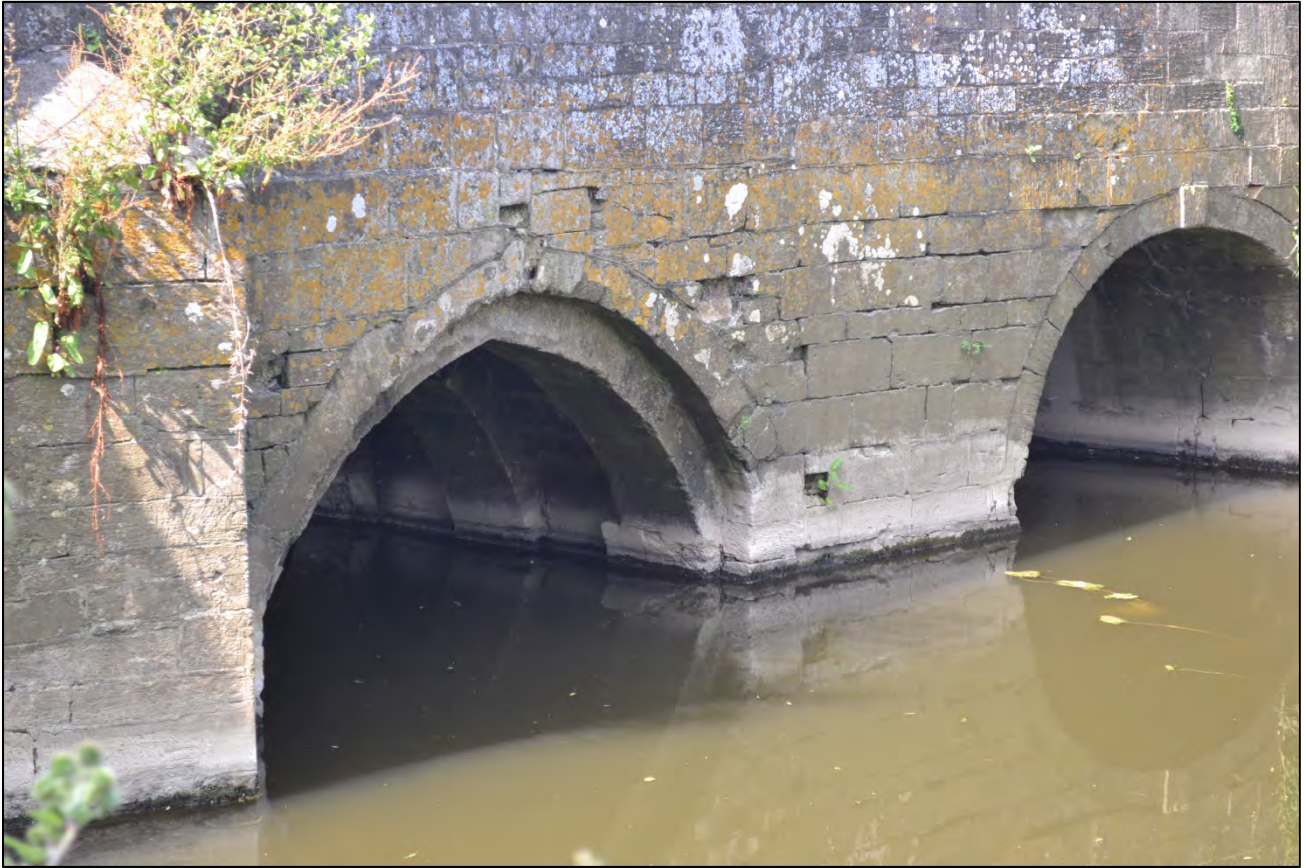
Plate 1: Ribbed arches beneath one side of Staverton Bridge, River Avon (© Antony Firth/Fjodr)
