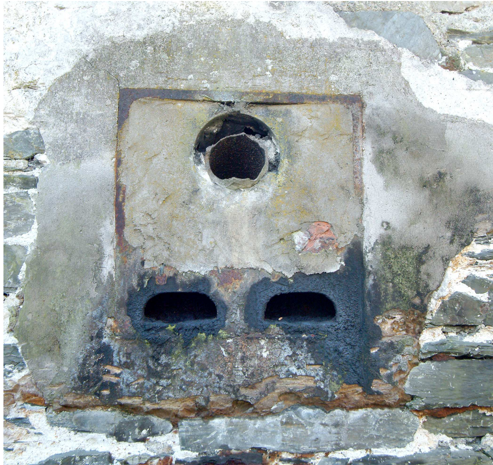
Figure 43. Wall box in outer face of north wall of building range immediately south of former incorporating mills. Broken pipe from later reuse is visible in upper hole. (NMR: DP003397)
