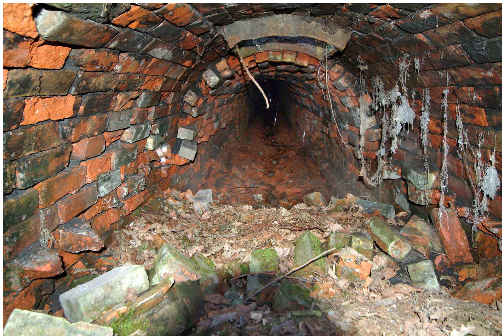
Figure 12. Internal view of east end of boiler house flue, looking west. (NMR: DP003402)
