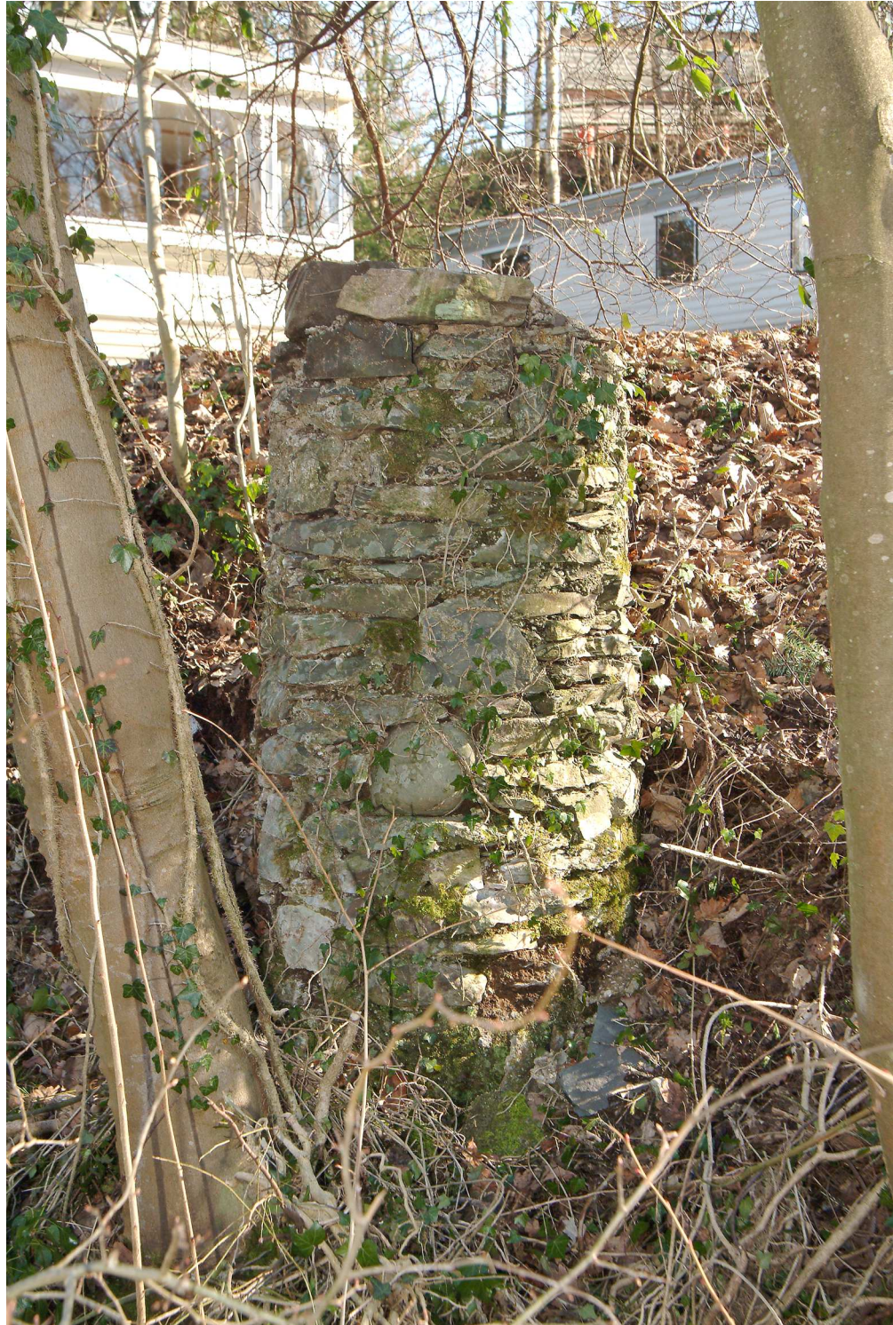
Figure 13. Northernmost surviving pillar which supported the steam pipes to the little engine house, looking south. (NMR: DP003406)
