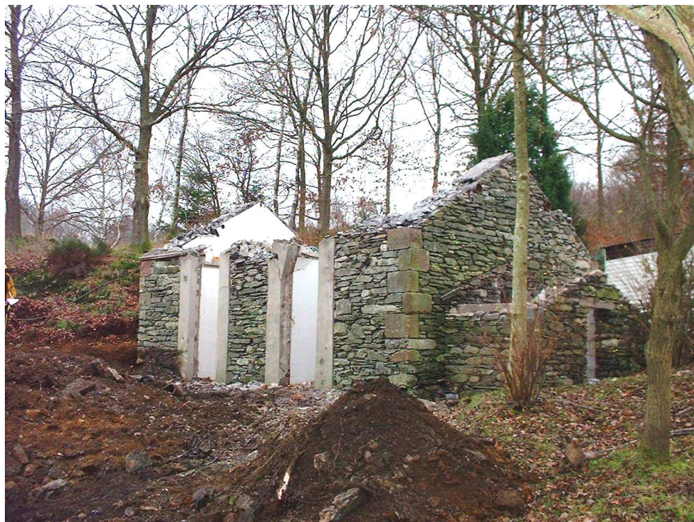
Figure 14. The oil engine house near the corning house in process of demolition, looking north west. (Abby Hunt, November 2003)
