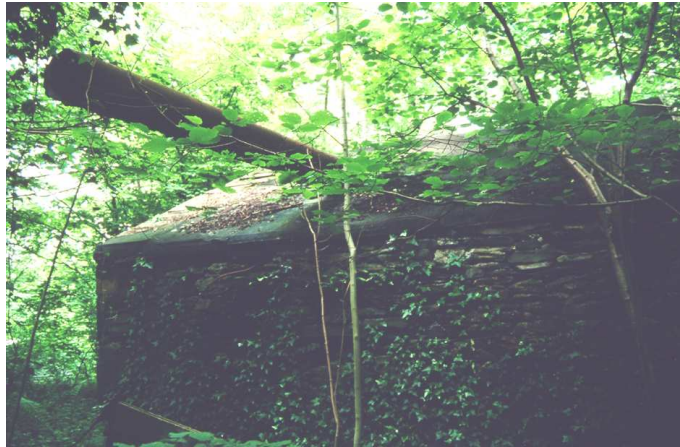
Fig 85. The rear of the heater house (building 47a) in 1991. (Davies-Shiel Collection, copyright reserved)
