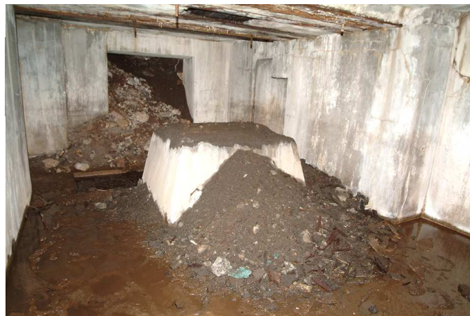
Fig 54. The basement beneath incorporating mill 34 mark II, looking south towards the wheel-pit. Note the iron beams in the ceiling which helped support the weight of the edge-runner mill immediately above. (NMR DP003439)
