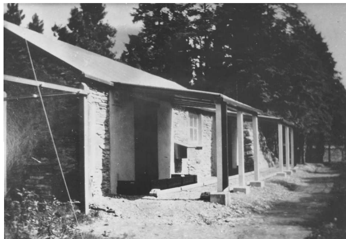
Fig 79. The front of the higher stove house during reconstruction in 1929. (Patterson Collection, ©English Heritage.NMR)
