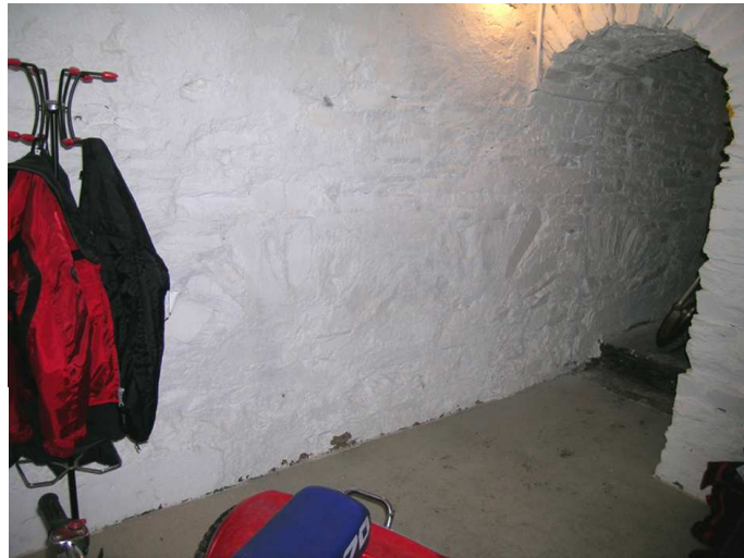
Fig 38. The three blocked, arched openings in the south-west ground-floor wall of the Clock tower. (Tony Berry, June 2005)
