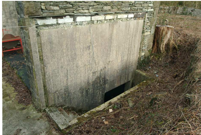
Fig 53. The staircase to the basement beneath incorporating mill 35 mark II. (NMR DP003443)
