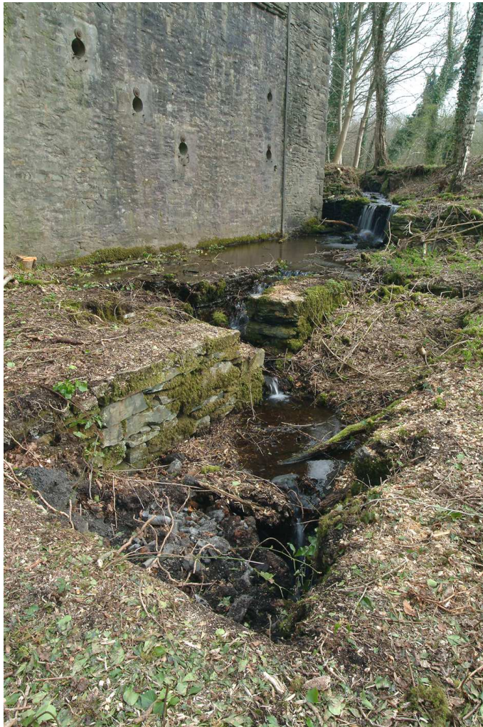
Fig 23. The infilled waterwheel-pit at the lower corning house mark IV. (NMR DP003476)
