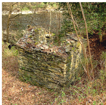
Fig 109. The privy (building 73) to the reel and glaze house, from the south-west. (NMR DP003487)
