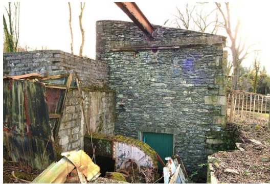
Fig 55. The header box and Armfield turbine at the exposed part- basement of incorporating mill 36 mark II. (NMR DP003444)
