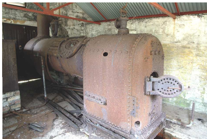
Fig 78. Robey boiler no. 19420 inside the 1929 boiler house at the lower stove. The water tank is just visible at left of frame. (NMRDP003493)
