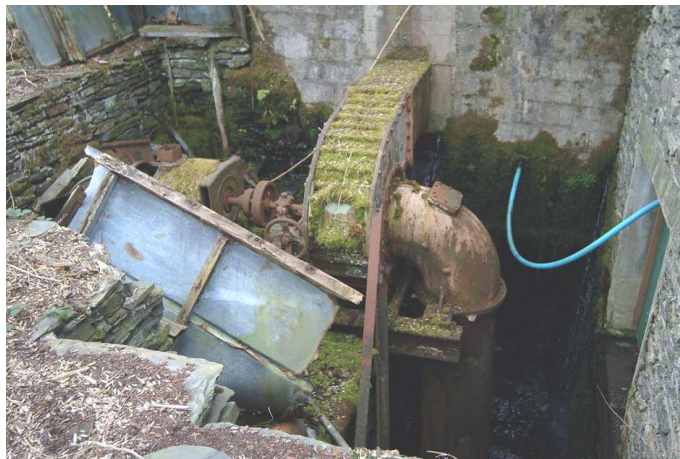
Fig 45. The exposed part-basement of incorporating mill 36 mark I, containing the later Armfield turbine. Note the patching in the rear wall showing that the supply pipe has been inserted into an existing structure. (NMR DP003472)
