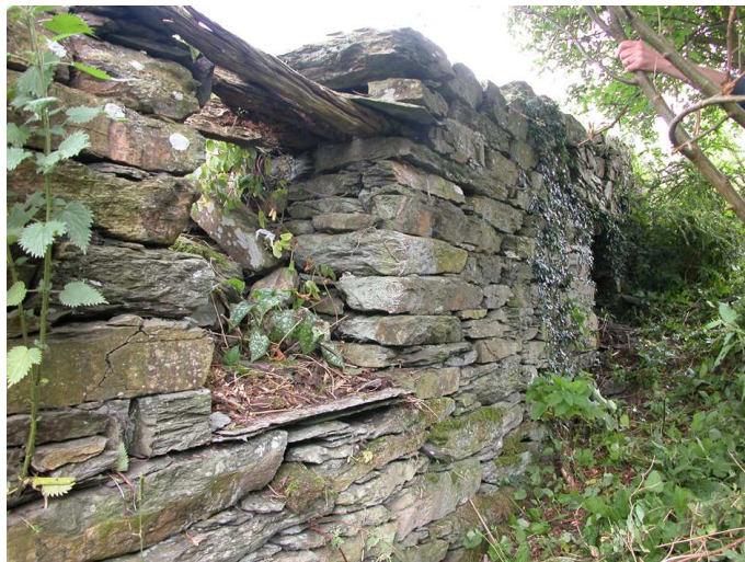
Fig 15. Exterior face of the surviving side wall of the ironworks bridge house viewed from the west. (Christopher Dunn, July 2005)
