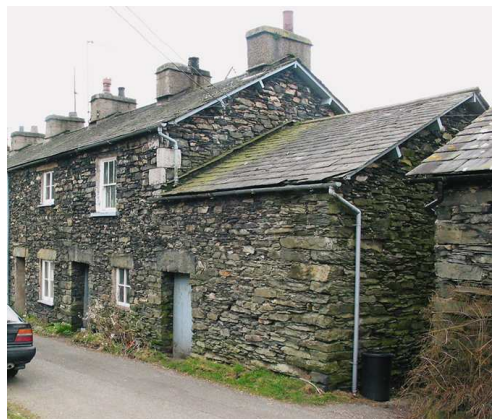
Fig 124. The front elevation of the unnumbered house and peat house at the north end of nos. 12-16 Low Wood (Simon Taylor, March 2004)
