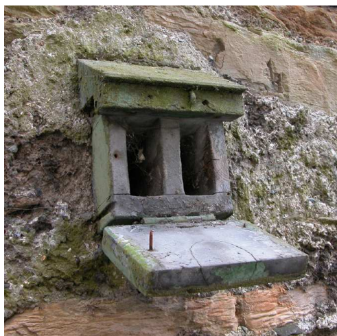
Fig 108. The key-box in the gable wall of the north-east office block. (Christopher Dunn, July 2005)
