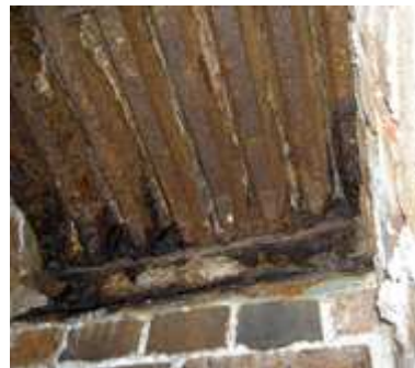
Fig 32. The iron straps supporting the flat-topped voids above the furnace vaults. (Christopher Dunn, March 2005)
