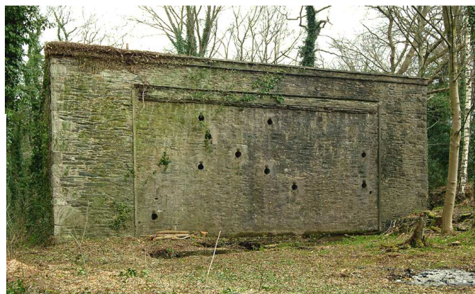
Fig 63. The outside of the rear wall of the lower corning house mark IV, showing the scar of the now vanished belt-drive house and the circular openings for the line shafts. (NMR DP003473)
