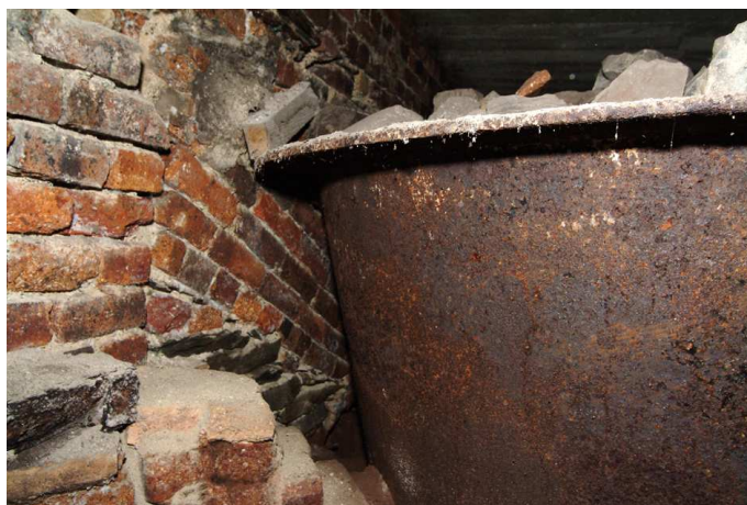
Fig 33. One of the boiling vats sealed beneath the modern inserted floor of the saltpetre refinery. (NMR DP003514)
