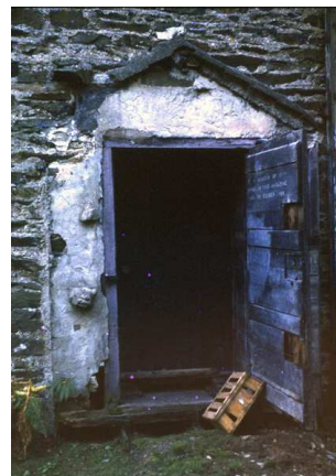
Fig 89. The entrance to the '1798' Roudsea magazine in 1969 prior to conversion to a summerhouse. (Palmer Collection, copyright reserved)
