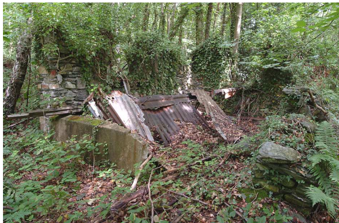
Fig 98. The remains of the women's dressing-room, viewed from the south. The concrete wall in the foreground presumably marks the division between it and the boiler house which has now disappeared. (NMR DP006419)
