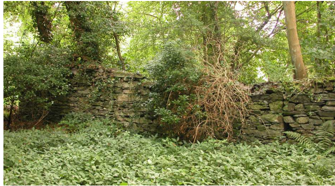
Fig 18. The rear wall of the ironworks stable and/ or cart house viewed from the north-east. (Christopher Dunn, July 2005)
