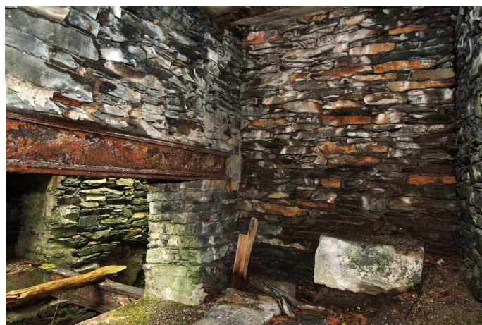
Fig 70. Inside the reduced basement beneath the south-western compartment of the glazing house, showing the stone block incorporated within the rear wall and the inspection opening for the turbine occupying the waterwheel-pit. (NMR DP003531)
