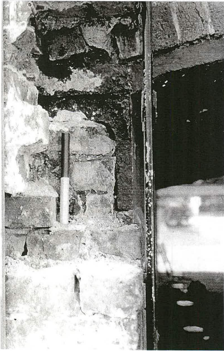
Main span, SW seating plate end opened up, from SE
