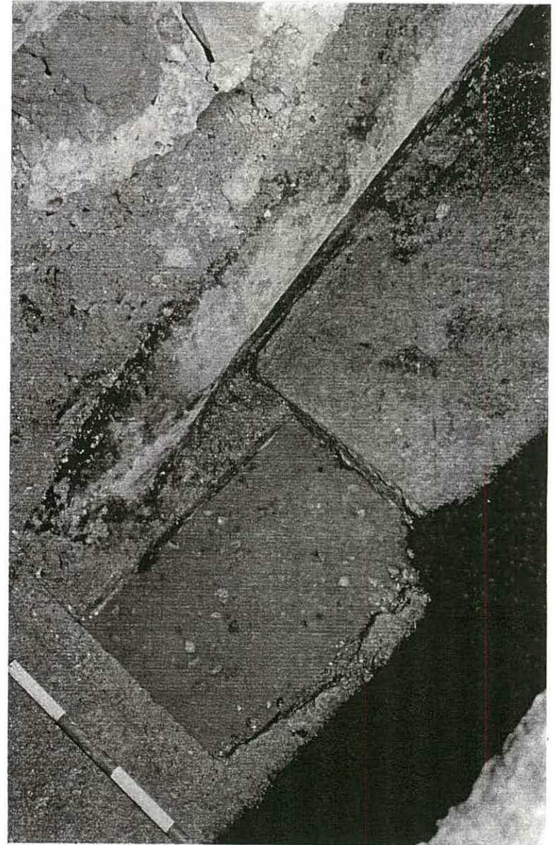
Side span, end of girder and corner of soffit plate from S
