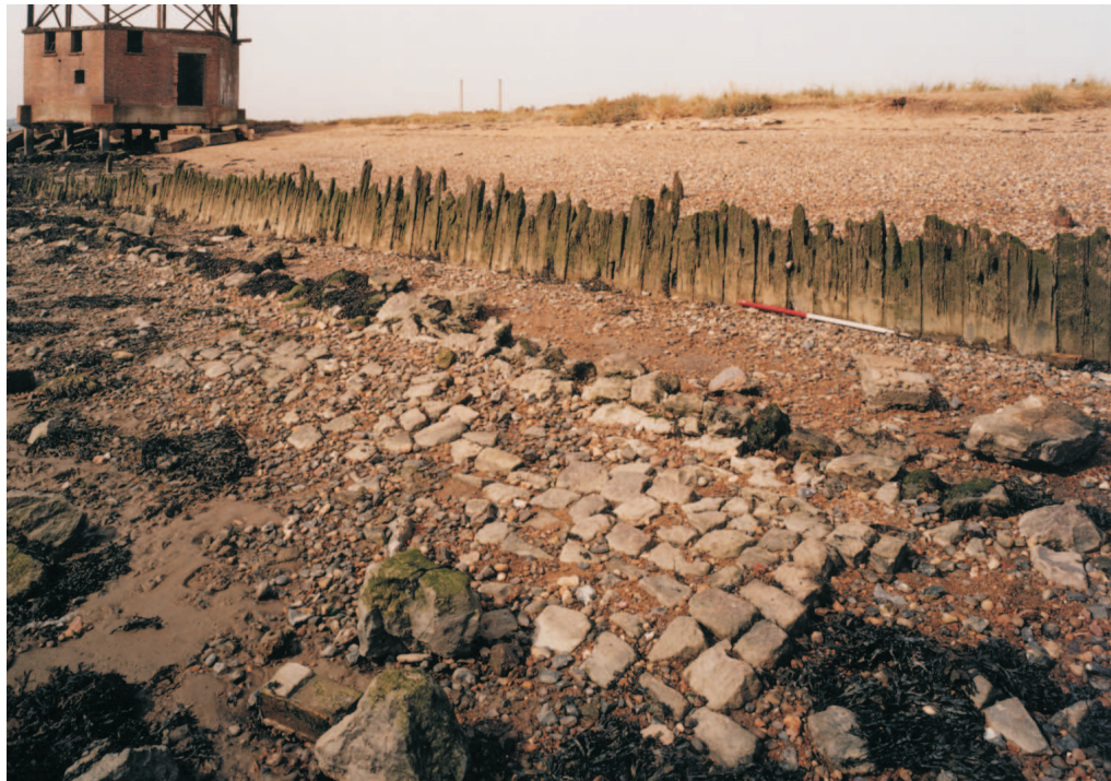
Figure 15 Revetment 2, showing collapsed wall in front (©Crown copyright NMR: AA/046704)
