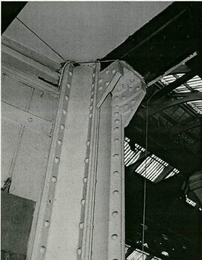
Figs. 19 and 20 – Shelf brackets riveted directly to the flanges of the Phoenix column— a technique similar to those being used in contemporary American skyscrapers (DP001755-6, Copyright © English Heritage)
