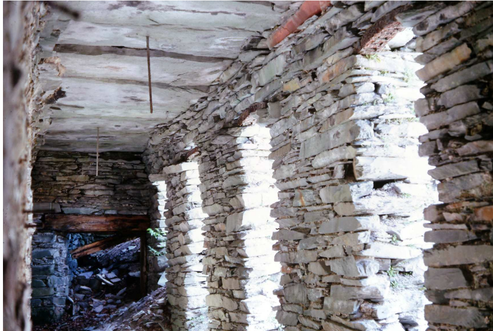
Figure 15. The boilerman's walk and openings into the vat room in the salpetre/sulphur refinery (building 24), photographed from the south in June 1967 (Davies-Shiel collection, copyright reserved)
