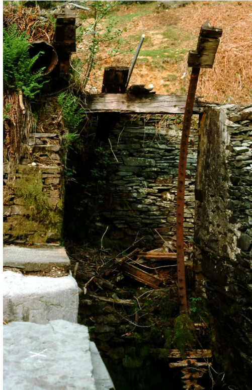
Figure 51. The wheel-pit to glazing house no. 3 (building 9) in 1982. According to the MMB the wheel was under-shot, but Mike Davies-Shiel suggests it was close-breasted (Davies-Shiel collection, copyright reserved)
