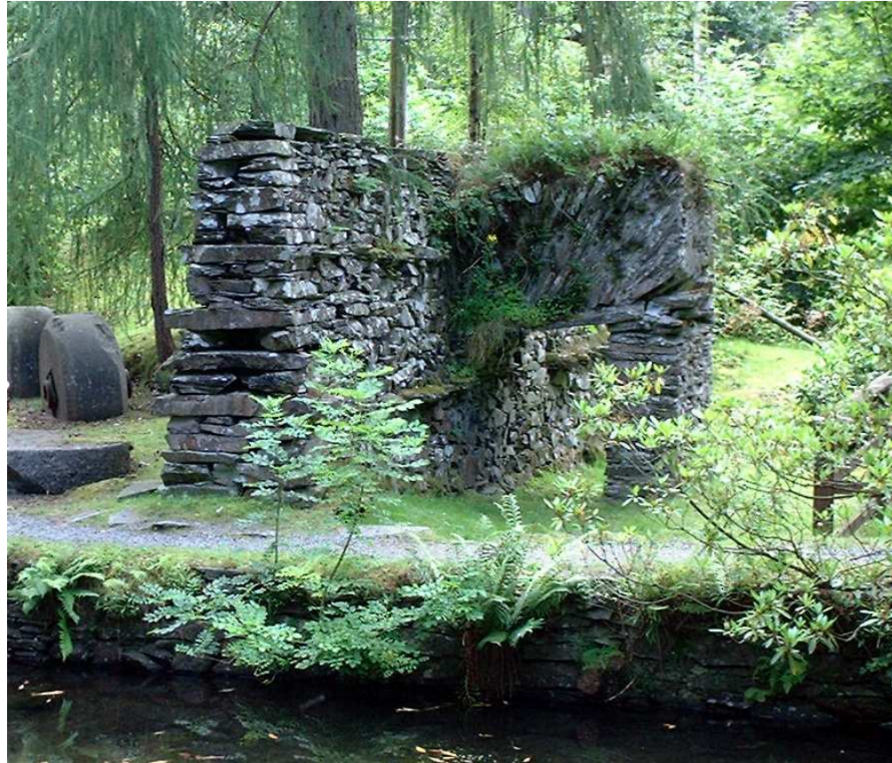
Figure 35. The buttress against the west side of blast wall BW1 at the lower mill site
