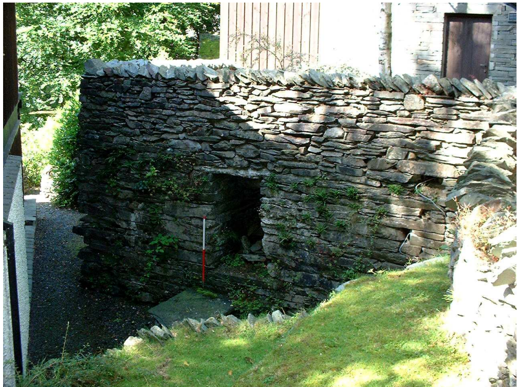
Figure 38. Surviving fabric at the east end of mill 6. Masonry below the lintel covering the passage is original, erected everything above is modern
