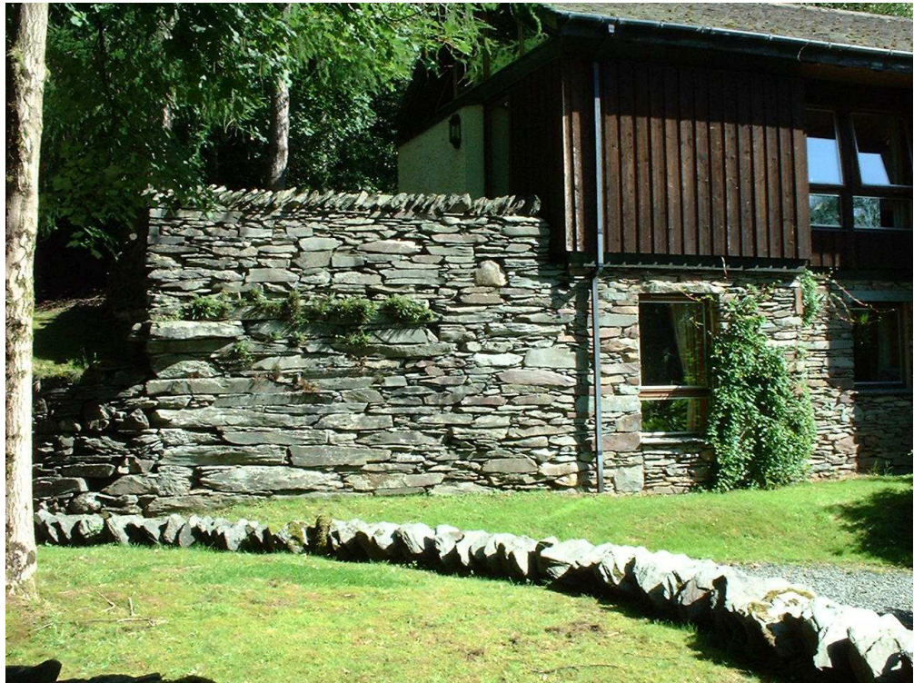
Figure 37. Surviving fabric at the west end of mill 5. The larger stones beneath the plant line are in-situ original masonry; the rest has been rebuilt when Lodge 16 was
