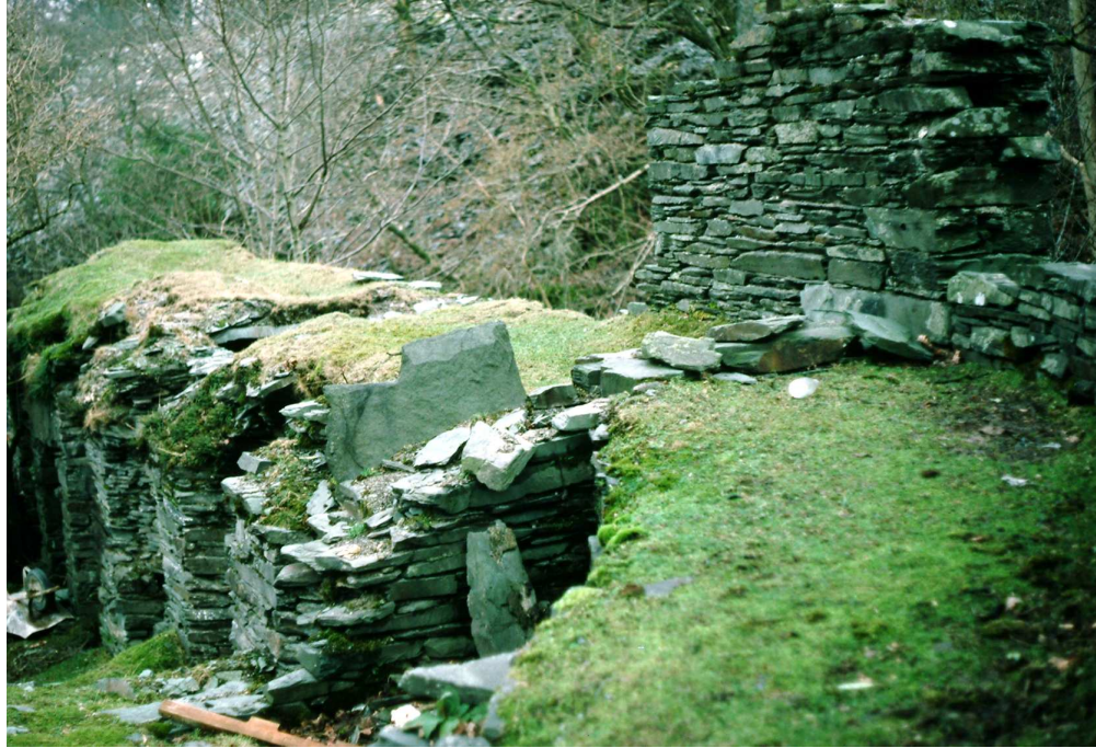
Figure 17. The boilerman's walk and openings into the vat room, photographed from the north-west in February 1983 (Davies-Shiel collection, copyright reserved)
