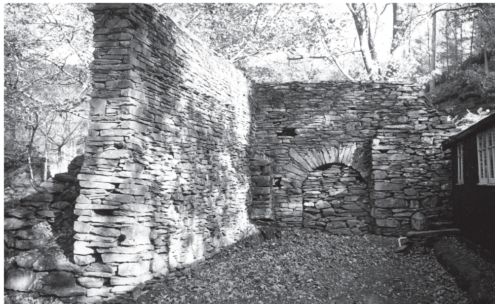
Figure 50. Blast wall BW8 shielding the northern corner of corning houses nos. 3 and 4, photographed in the 1960s. Note the arch for the tramway (Barter collection, copyright reserved)
