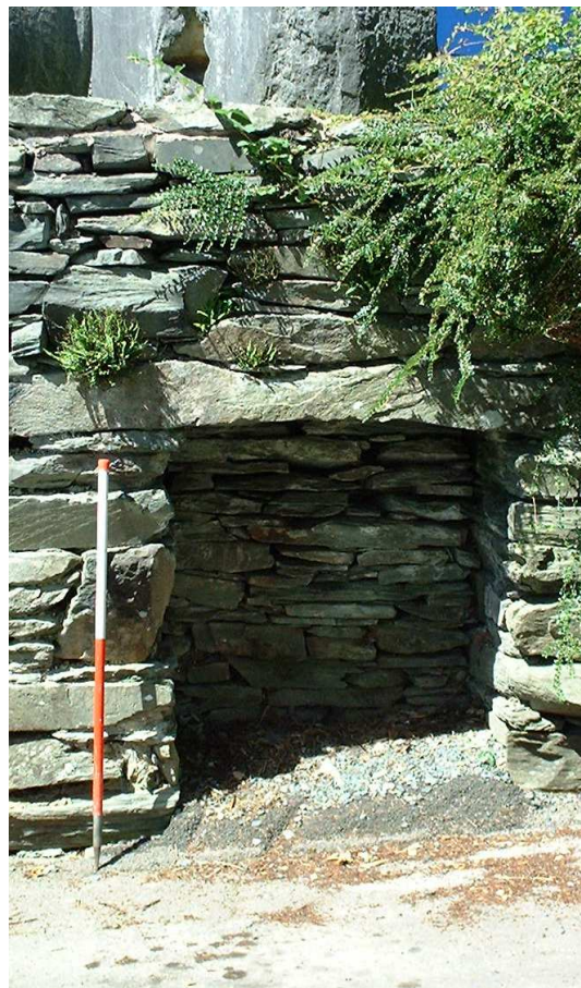
Figure 46. The blocked door opening in the facade of mill 12. Note that the modern ground surface has been raised, and obscures the base of the opening
