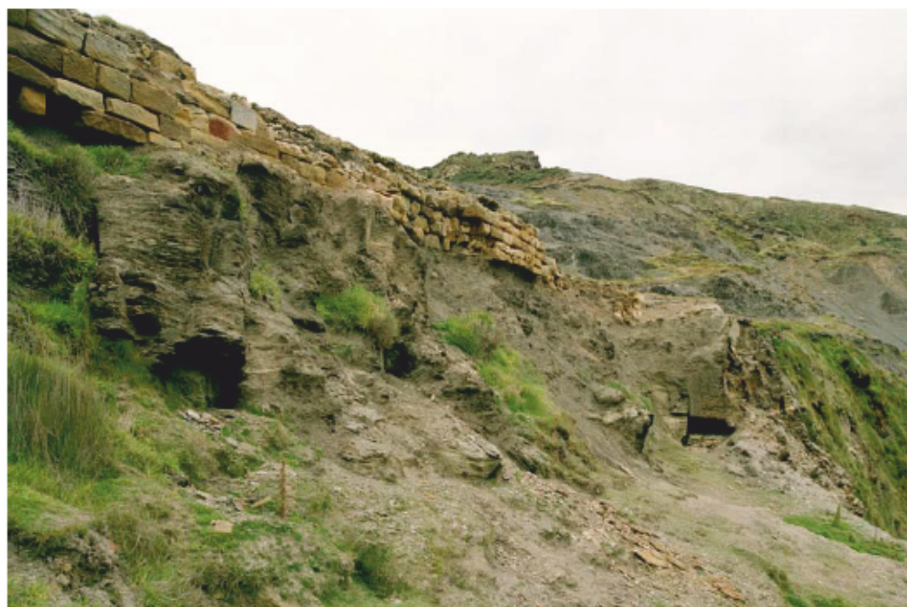
Figure 48. The collapsed ledge at the edge of the alum-house shelf. Note the entrance to mine 5 at right of frame, and wall 3 (part of the alum house) along the top of the rear edge of the ledge. (NMR AA040229)
