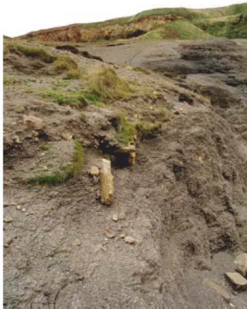
Figure 35. Detail of conduit 1 above the north-east corner of the alum- house shelf. Displaced stones overlie the scree below. (NMR AA040230)
