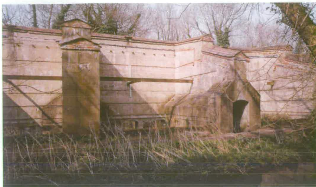
Figure 25 1880s gunpowder incorporating mills [52], note the remains of the drenching mechanism on top of the rear wall (AA044443). (c) English Heritage
