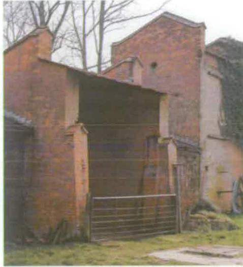
Figure 39 View of the Cordite kneading, pressing, motor and engine house No.30, showing the central passageway (AA044455). (c) English Heritage
