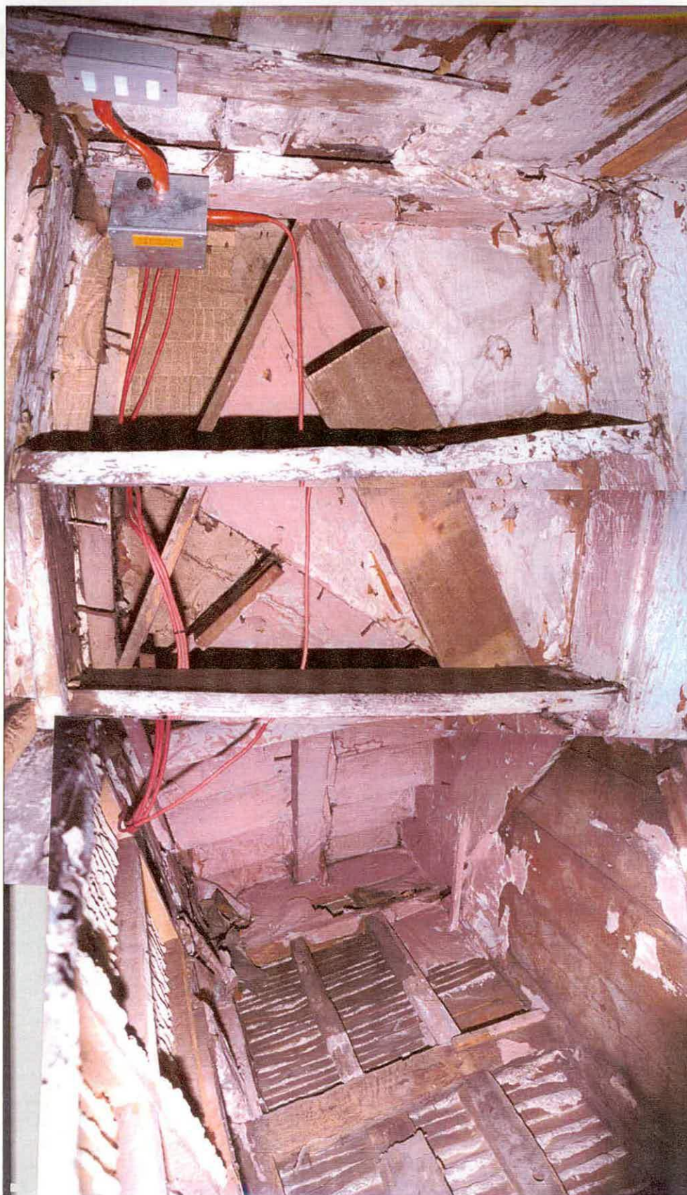
Figure 53, a panoramic photomontage of the underside of the winders and the upper flight of the stairs at the east end of the Blue Anchor Lane Wing, looking up. Note the newspapers glued to the soffit of the winders.
