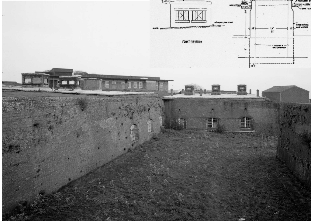
Figure 34 The South-West Face Casemates and the South-West Flank casemates, from the NW, showing the windows at ditch level (inserted into the former embrasures) and the lantern lights placed on the roof around 1913. The drawing shows the lanterns as proposed in 1913 (photo NMR: AA043990 © Crown copyright 1998, drawing 402652 © HMPS)
