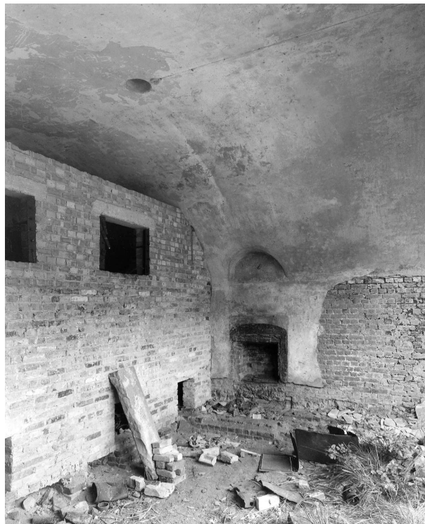
Figure 80 Interior of a Haxo casemate in the South Flank Casemates, showing the original vault with circular smoke vent, fireplace, and the inserted wall (at left) partitioning off the front of the casemate (NMR: AA043998 © Crown copyright 1998)
