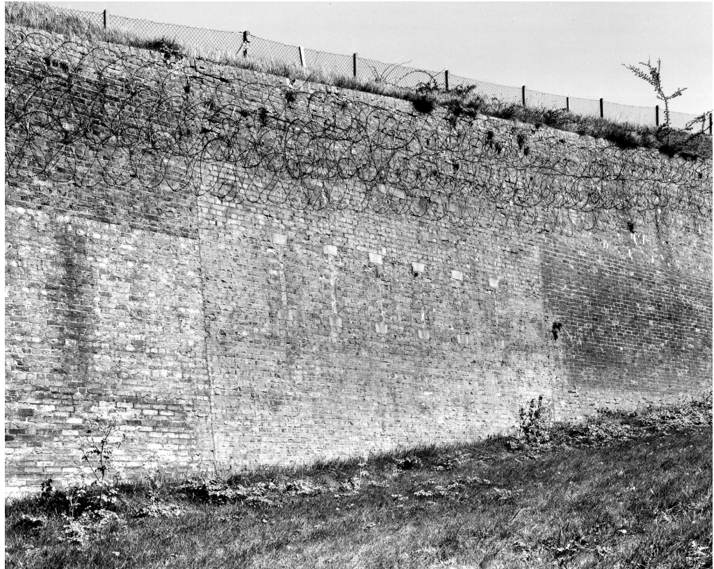
Figure 20 Inserted walling in the counterscarp revetment of the NW Bastion with, just visible, blocked loopholes (NMR: BB032730 © Crown copyright 1998)
