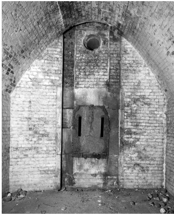
Figure 42 Inner NW Bastion; a gunroom in the Right Flanking Casemates. Detail of the ditch wall showing the scars from the original sliding shutter and its replacement, a small fixed steel shutter perforated with loops for small arms fire (NMR: AA043967 © Crown copyright 1998)
