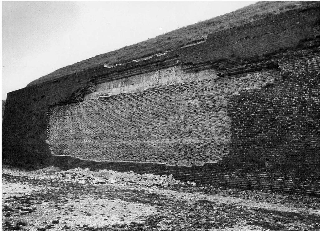
Figure 18 North end of the western scarp revetment of the NW Bastion, in 1959, showing defective brickwork cut out prior to repair. Note the heightening marked by a junction between brickwork and chalk ashlar, probably representing the Napoleonic and 1860s construction phases respectively (A6207/4 © Dover Museum)
