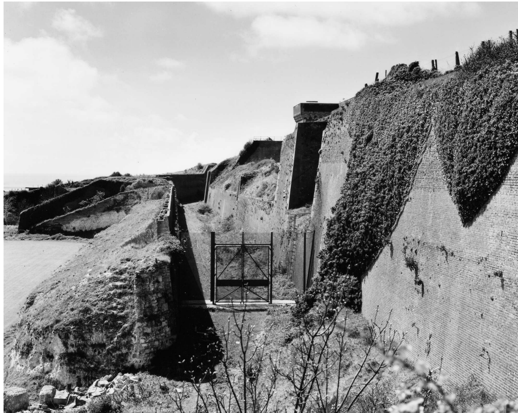
Figure 23 The south face of the Citadel, from the east. The inner ditch of the tenaille, now guarded by a modern gate, survives, while to the left, the tenaille itself has been cut away leaving a 45° slope; the outer ditch has gone (NMR: BB032737 © Crown copyright 1998)
