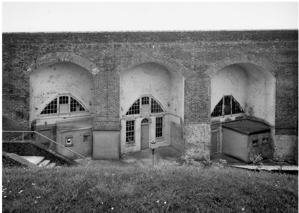
Figure 33 The rear elevation of the West Face Casemates. The central casemate retains much of its original appearance with central fan-lit entrance and flanking windows. Above the entrance another window rises to the crown of the parabolic vault (NMR: AA043936 © Crown copyright 1998)
