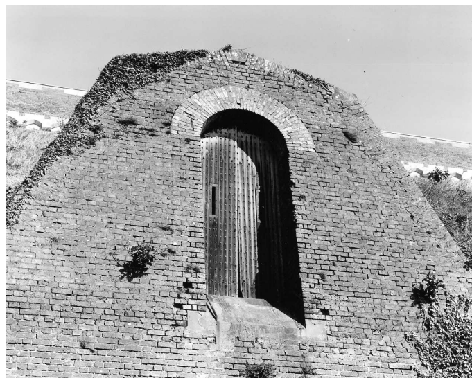
Figure 25 Reinforced doors in the scarp revetment of the inner South Ditch, formerly leading onto a bridge to the tenaille (NMR: BB032740 © Crown copyright 1998)
