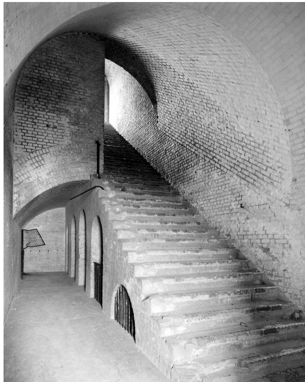
Figure 76 Stairway between levels in the South Flank Casemates, looking NW (NMR: AA043996 © Crown copyright 1998)
