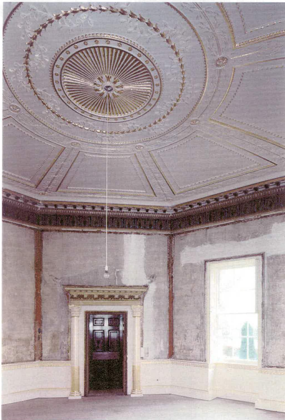
Figure 1, the saloon in its present condition, after partial restoration by English Heritage. Photograph: English Heritage.
