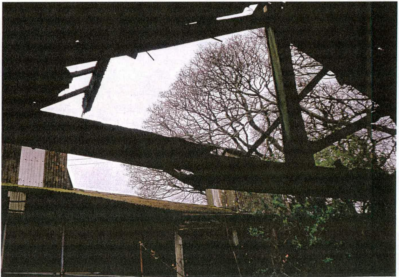
Fig. 22 Engineers' Shop: collapsing roof, 2002
