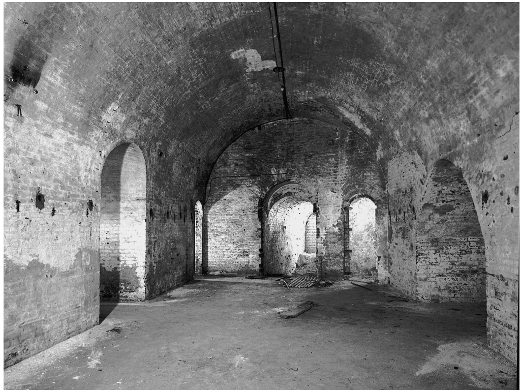
Figure 13 Clarence Tower, basement level of the east casemate, looking north. The entrance at centre rear of the photo leads to the Main Magazine, the one on its right leads into the NW turret (©NMR: AA031464)
