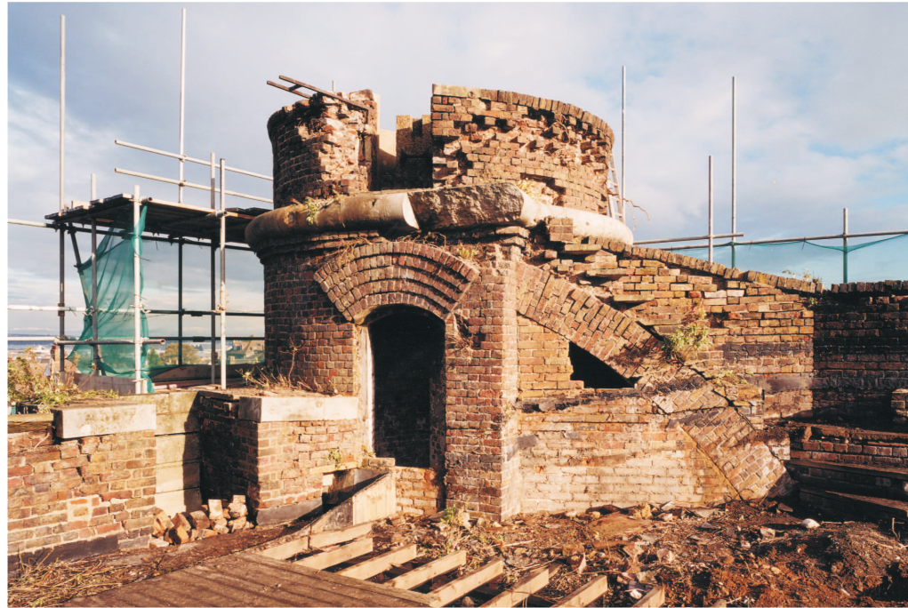
Figure 36 Clarence Tower; the NE turret. Note the steps over the flying buttress, ascending to the observation platform (© NMR: AA020048)
