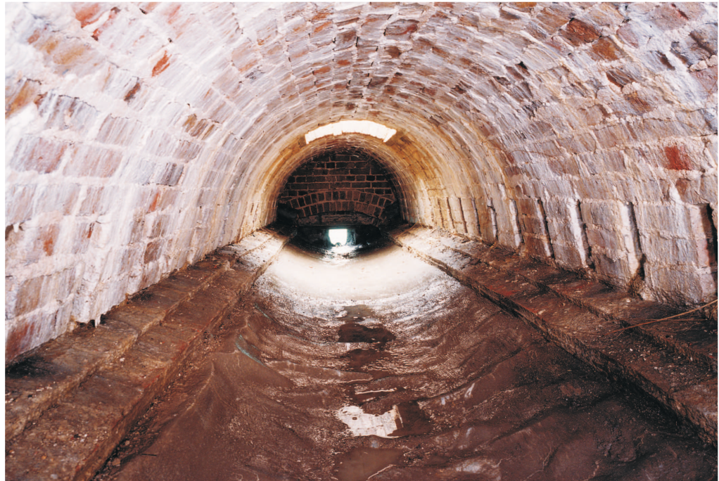
Figure 31 Clarence Tower; interior of the large central cistern, situated between the roof level and the first floor vaults, looking north to the drainage aperture (© NMR: AA021147)
