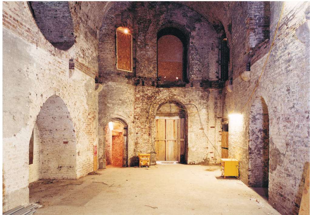
Figure 17 Clarence Tower, west casemate ground and first floor levels looking north. The timber floor structure has gone, leaving only the stone corbels from the tie beams. Note the different design of the artillery embrasures on the ground and first floors (at left) (© NMR:AA020022)
