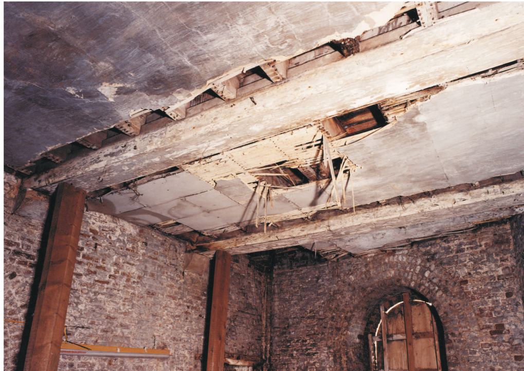
Figure 21 Clarence Tower, detail showing the structure of the ceiling in the ground floor east casemate. The wooden props at left are modern (© NMR: AA020015)
