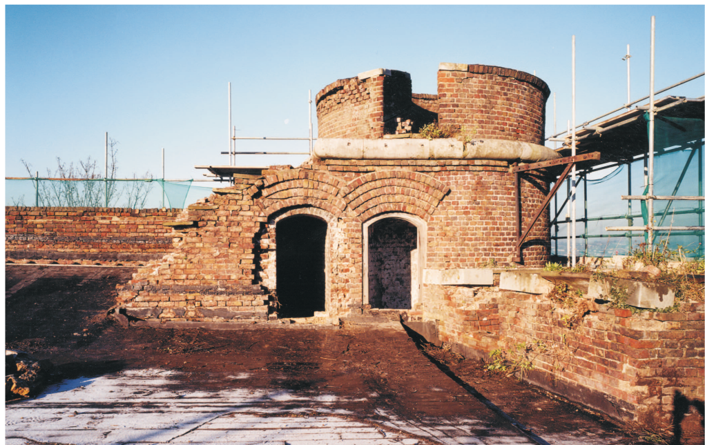
Figure 34 Clarence Tower; the NW turret. The right-hand entrance is to the newel stair, the left-hand to the store room (© NMR: AA021108)
