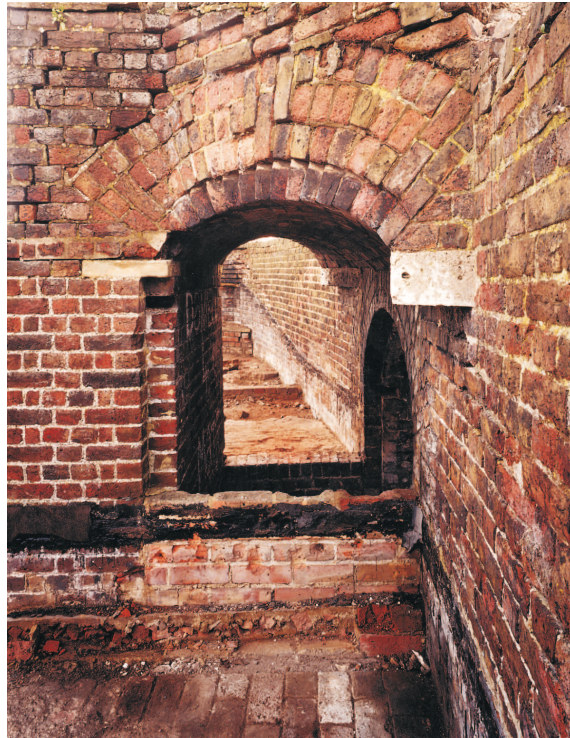
Figure 33 Clarence Tower; detail of the entrance to the porch to the ammunition shaft at roof level (© NMR: AA 021128)
