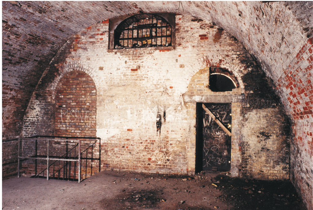
Figure 42 The West Casemates, interior at first floor level showing windows in the west wall (© NMR: AA020006)
