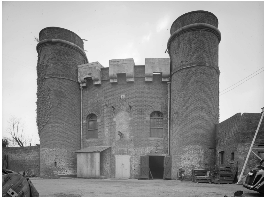
Figure 14 The north, entrance elevation of Clarence Tower in 1961. Note the RSJ projecting centrally at first floor level, with lifting gear linked to a winch in the shed below. This was for lifting heavy loads up and down from basement level via a vertical shaft, for which the trapdoors can just be seen at ground level (© Crown copyright NMR: AA61/2554)
