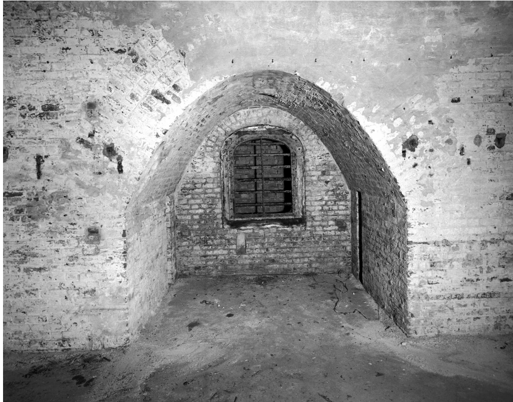
Figure 15 Clarence Tower; artillery recess in the basement west casemate, with its secondary barred frame of asylum or prison vintage (© NMR: AA021155)
