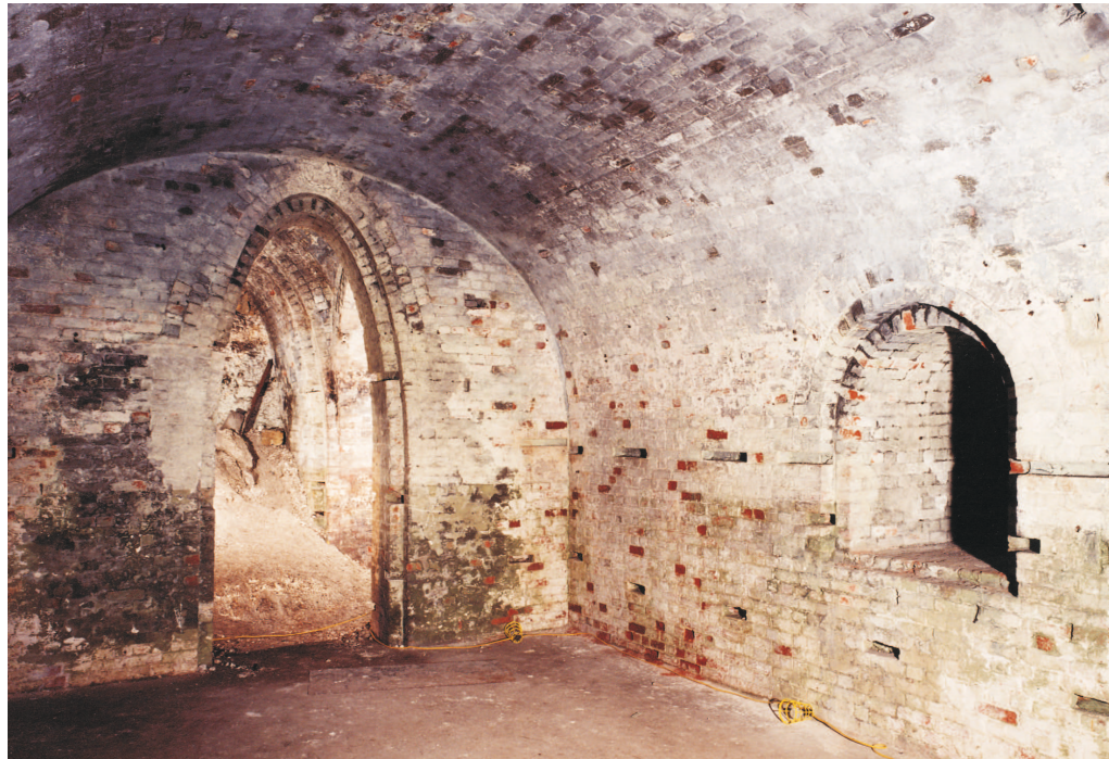
Figure 37 Clarence Tower; the main magazine, looking north-west. Note the parabolic entrance and the lighting recess (at right) (© NMR: AA020011)
