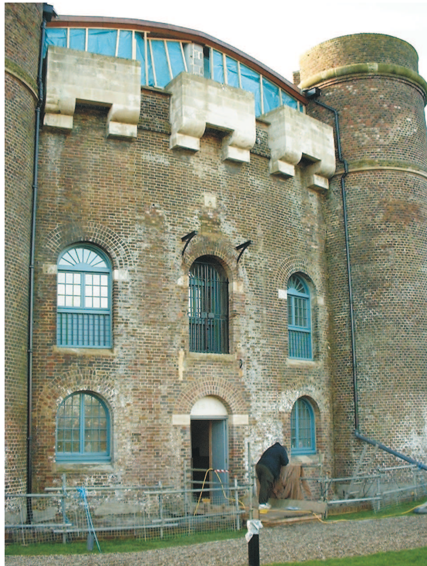
Figure 9 The north elevation of Clarence Tower, with refurbishment nearing completion, in December 2002. Note the Portland machicolations, original entrance at first floor centre and new entrance at ground floor centre. The structure above the machicolations is modern (author)
