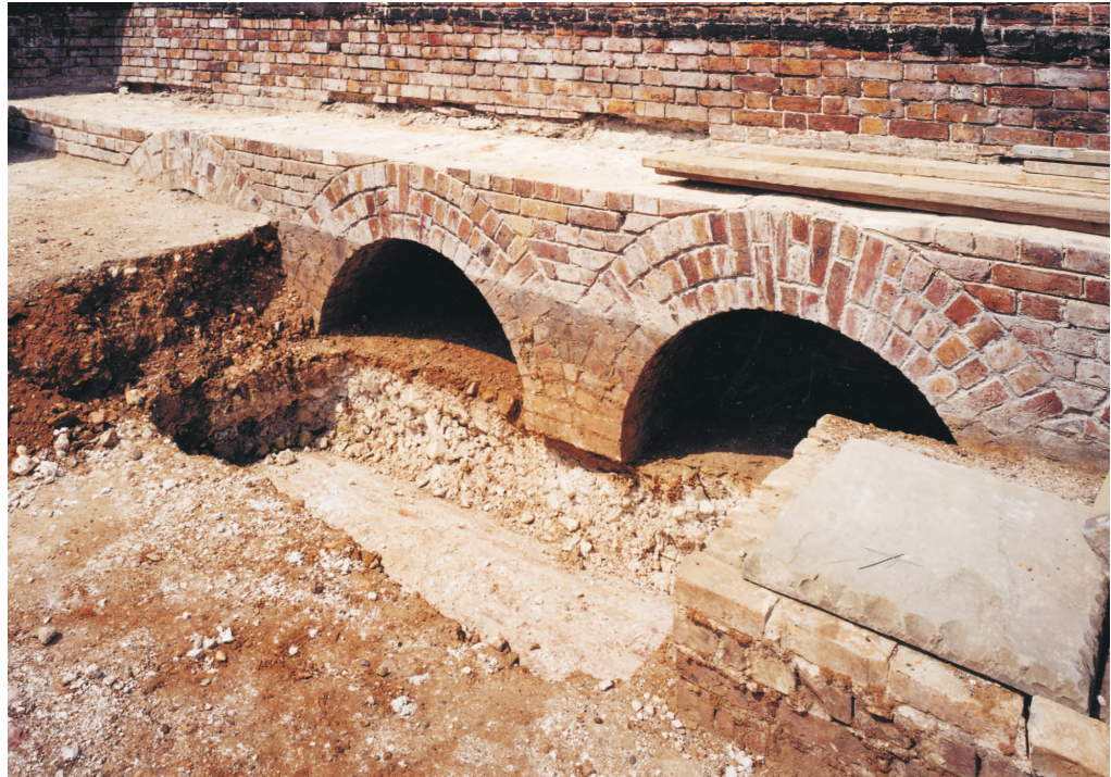
Figure 30 Clarence Tower; western infantry step . The stone flags above the relieving arches have been removed. The trench at centre is cut through original chalk infill which itself sits above the vault of one of the roof cisterns. The brown soil and rubble deposit over the chalk post dates the removal of the brick gun floor(© NMR: AA031471)
