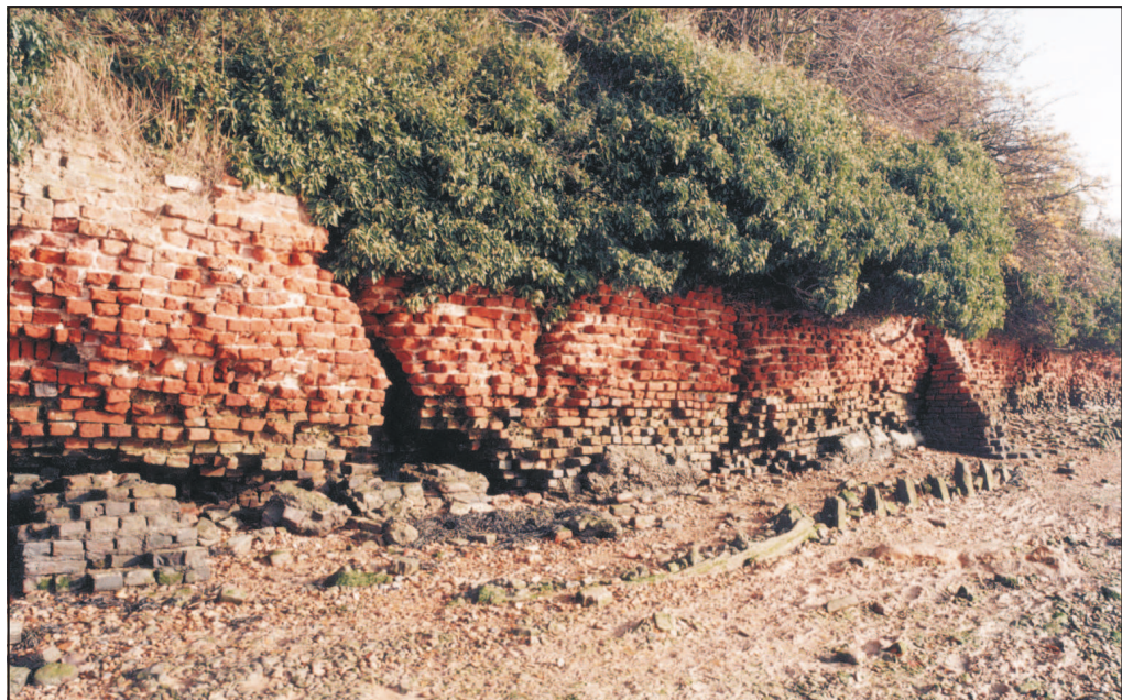
Figure 25 The revetment wall of the lower gun line with the timber remains of the tidal defences in front (NMR: AA031343)
