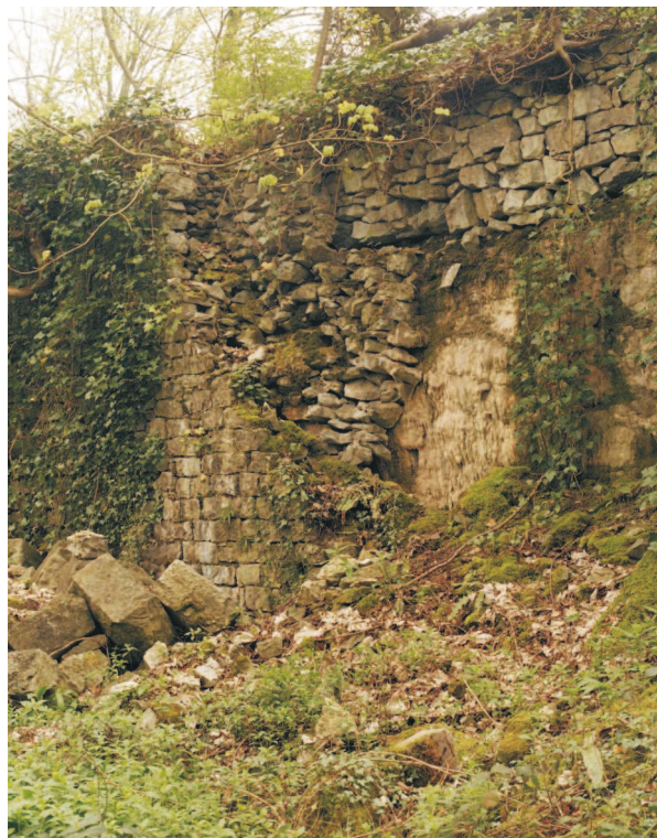
Figure 28. Wall collapse below the terraced walk (NMR: AA038825)
