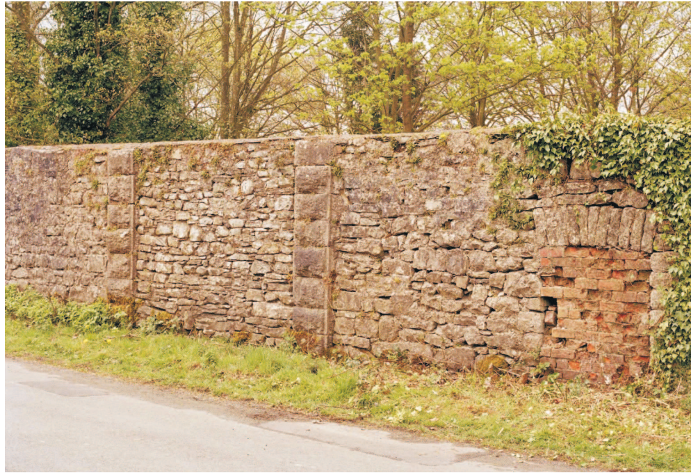
Figure 23. Blocked gateway and doorway in the perimeter wall (NMR: AA038836)
