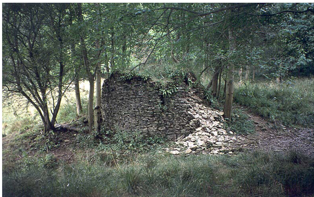
Figure 13: Collapsed stone structure adjacent to the Old Pond
