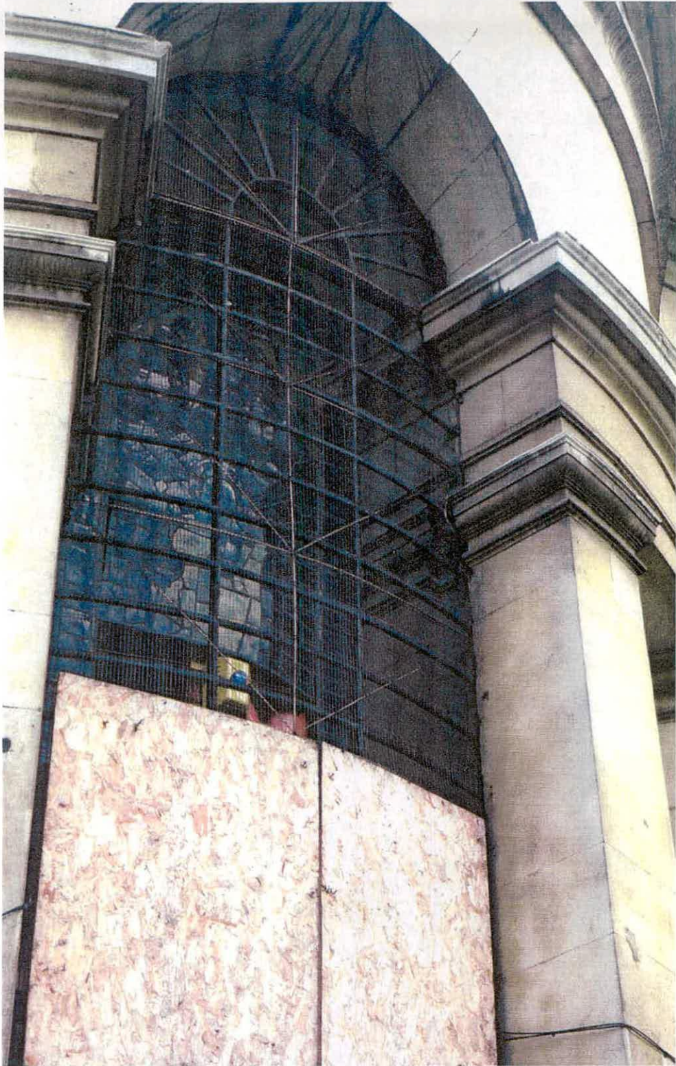
Fig. 14, a detail of the east window, showing the original ferramenta outside the plane of the later glazing and the rebate between the inner and outer columns, June 2002.
