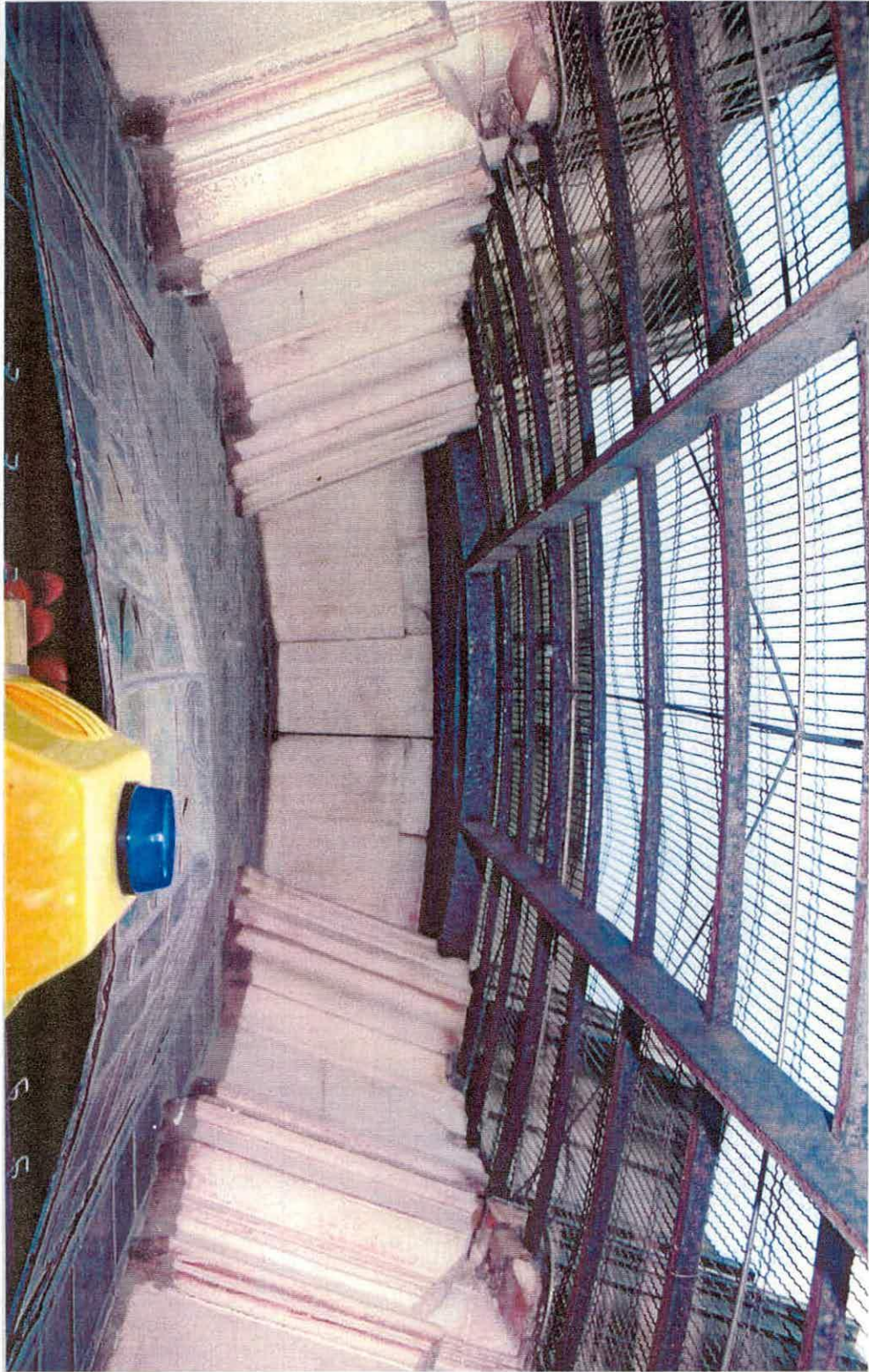
Fig. 34, the space between the original ferramenta and the Powell glazing in the centre light in the east window, looking upwards, June 2002. The buckling of the lower part of the surviving Powell glass is apparent in the glazing detached from the wire ties visible at the left-hand edge of the photograph.
