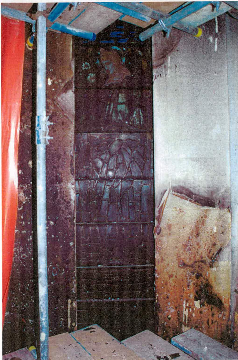
Fig. 31, the southern light in the east window, the figure of St Gabriel, after the fire of May 2000. The heat lifted the paint on the adjacent wall surface but left the glazing intact.
