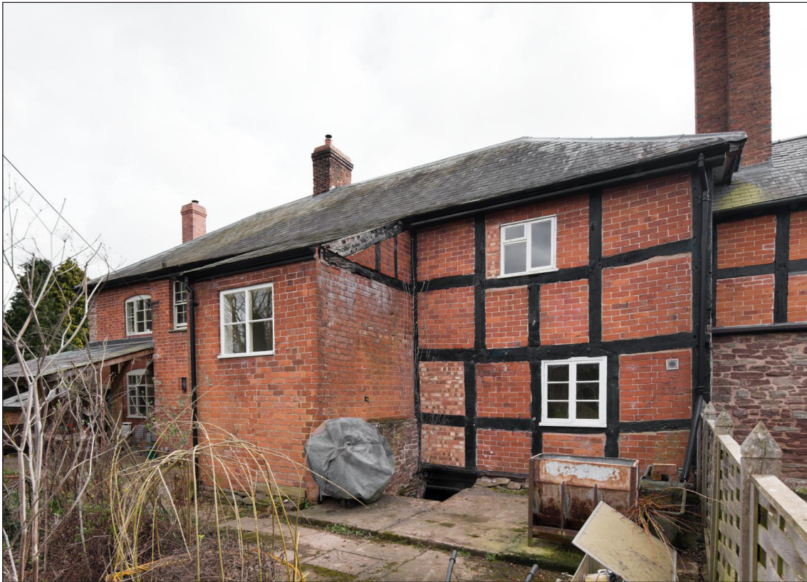
Figure 20 North elevation, showing stair turret, mostly reconstructed in the 19th or 20th century but with an early stone base (DP221701)
