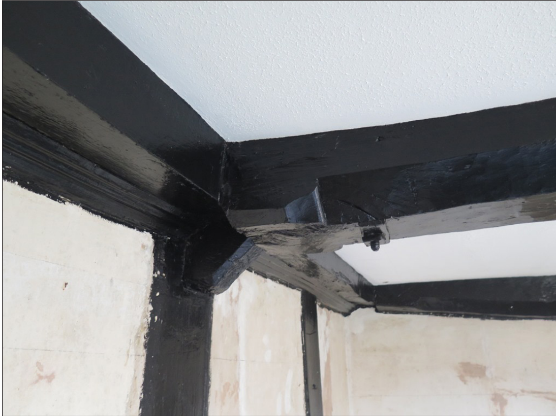
Figure 22 Detail of reused 17th century beam in the southwest room of the hall range. Photo Stuart Mee.
