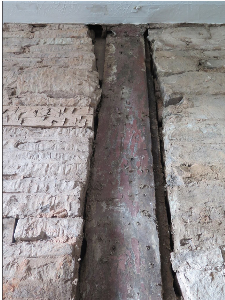
Figure 5 Central post in west elevation of cross wing showing rebate on its northern side. Photo Stuart Mee
