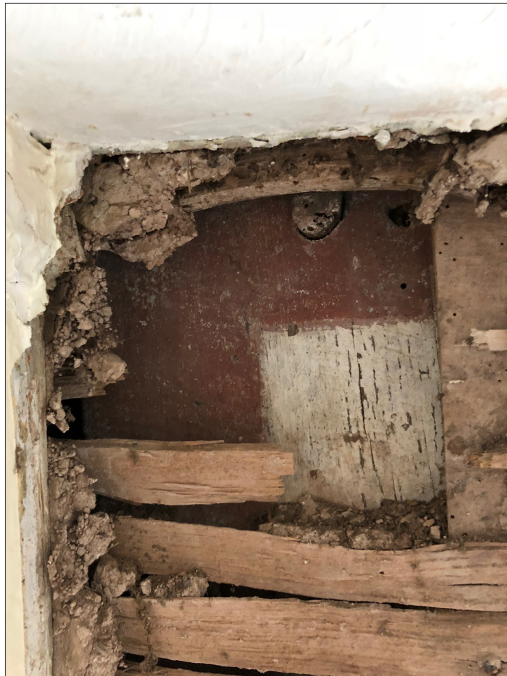
Figure 17 Detail of paintwork exposed during restoration of the south wall. Photo John Stevenson.
