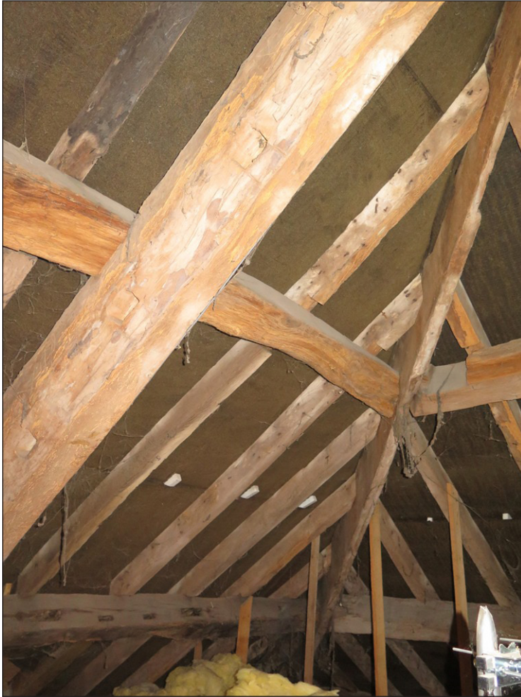
Figure 21 Detail of roof structure, showing reused timber elements, some with charring. Photo Stuart Mee.
