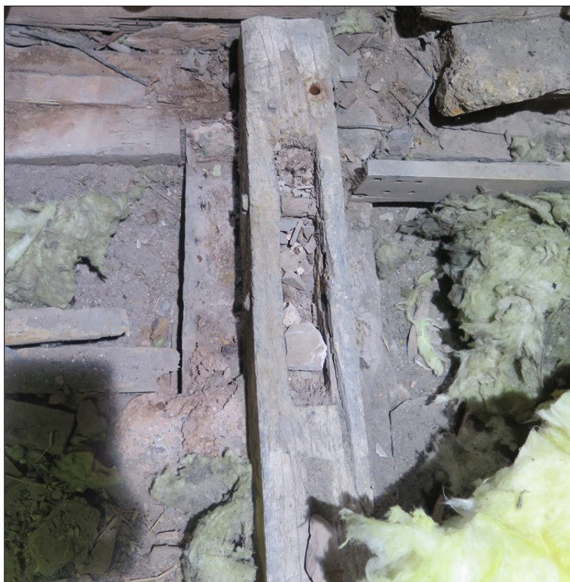
Figure 7 Tie beam of the original roof over the cross wing still in situ. Photo Stuart Mee
