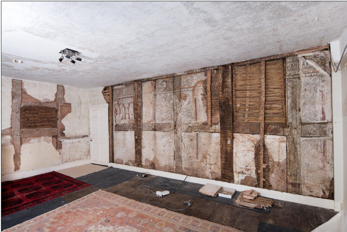
Figure 10 Main room in the first floor of the cross wing, showing exposed parts of decorative scheme (DP221673)
