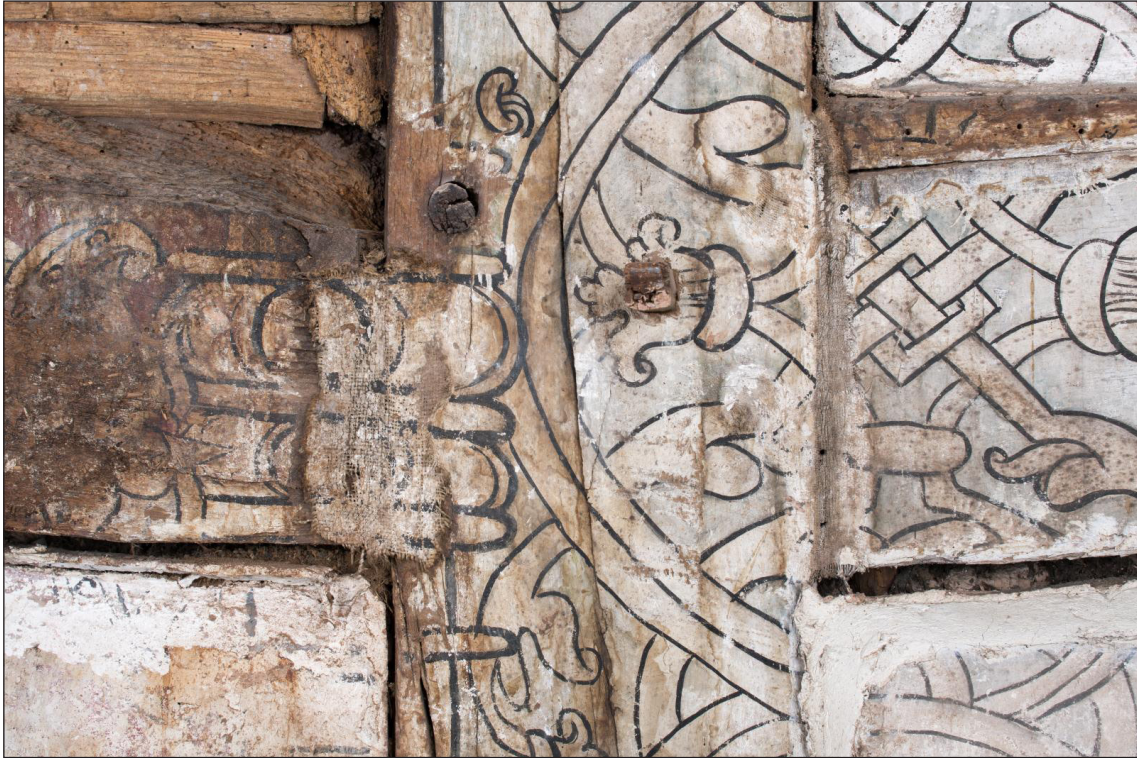
Figure 11 Detail of junction in timber frame, showing detail of small patch of cloth used to cover the joint on the left-hand side (DP221695)
