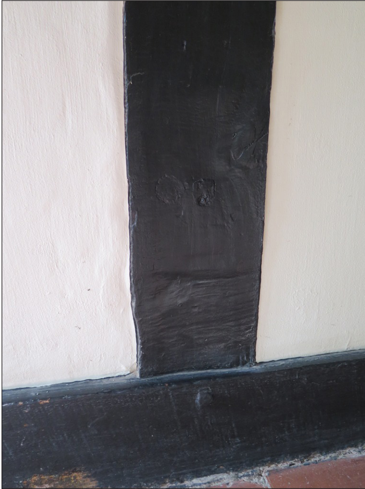
Figure 4 Detail of studs in east elevation of cross wing, showing the residual peg holes for a high-end bench arrangement. Photo Stuart Mee
