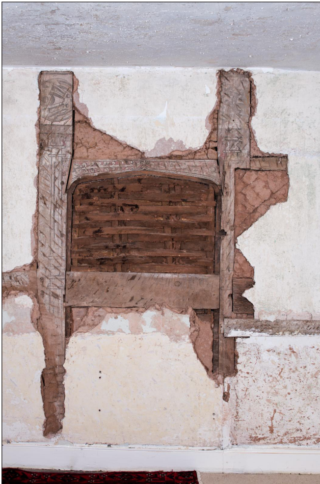
Figure 9 Doorway in the inserted cross wall between the northern and southern rooms at first-floor level (DP221674)
