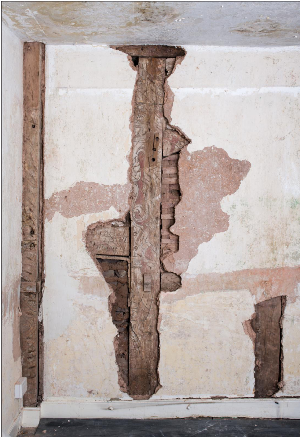
Figure 6 Exposed studwork of the west elevation of the cross wing at first-floor level with part of the doorhead for the garderobe visible on the northern side of the stud (DP221684)
