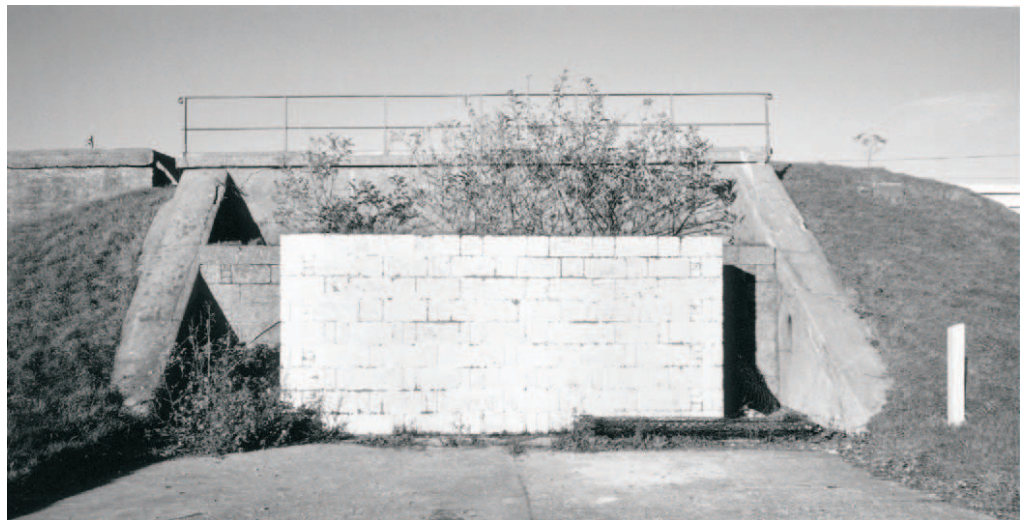
Figure 16 The entrance facade of magazine A, partially concealed by the Second World War blast walls
