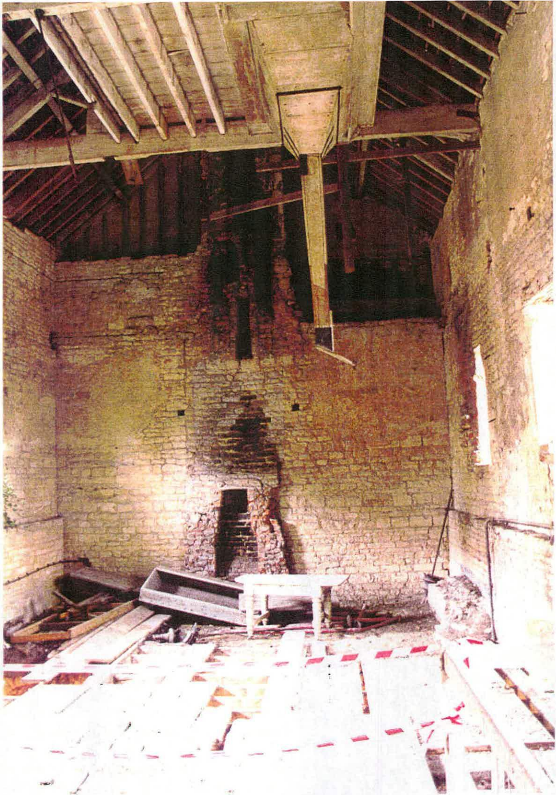
Fig. 24 A general view showing the interior of the upper levels in the three central bays of the brewhouse, looking south.
