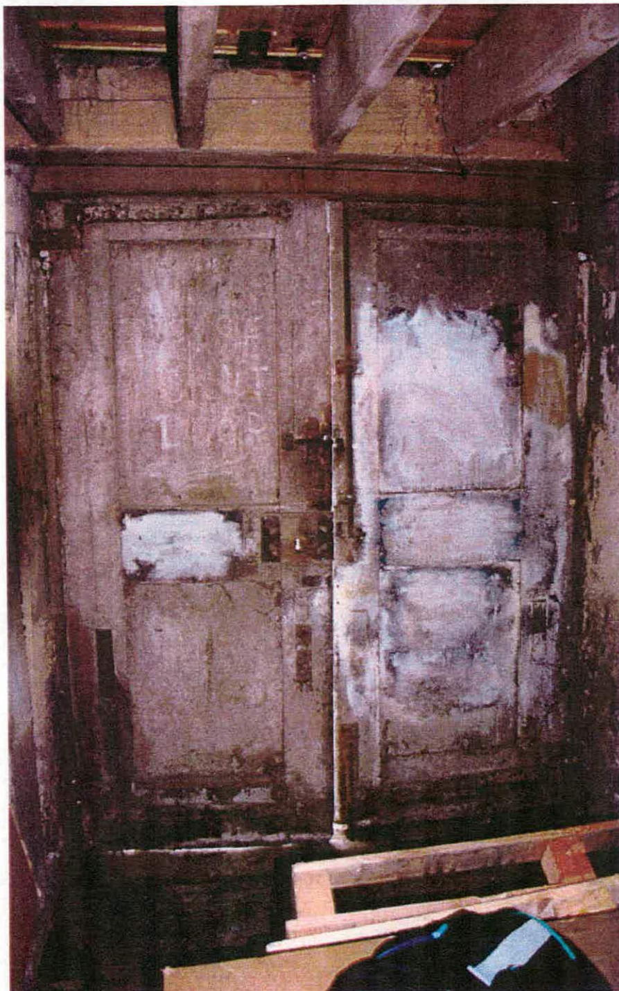
Fig. 43 The interior of the east doorway (fig. 19) into the central bays of the brewhouse. The early nineteenth-century inserted floor truncated the rounded head of the original doorway.
