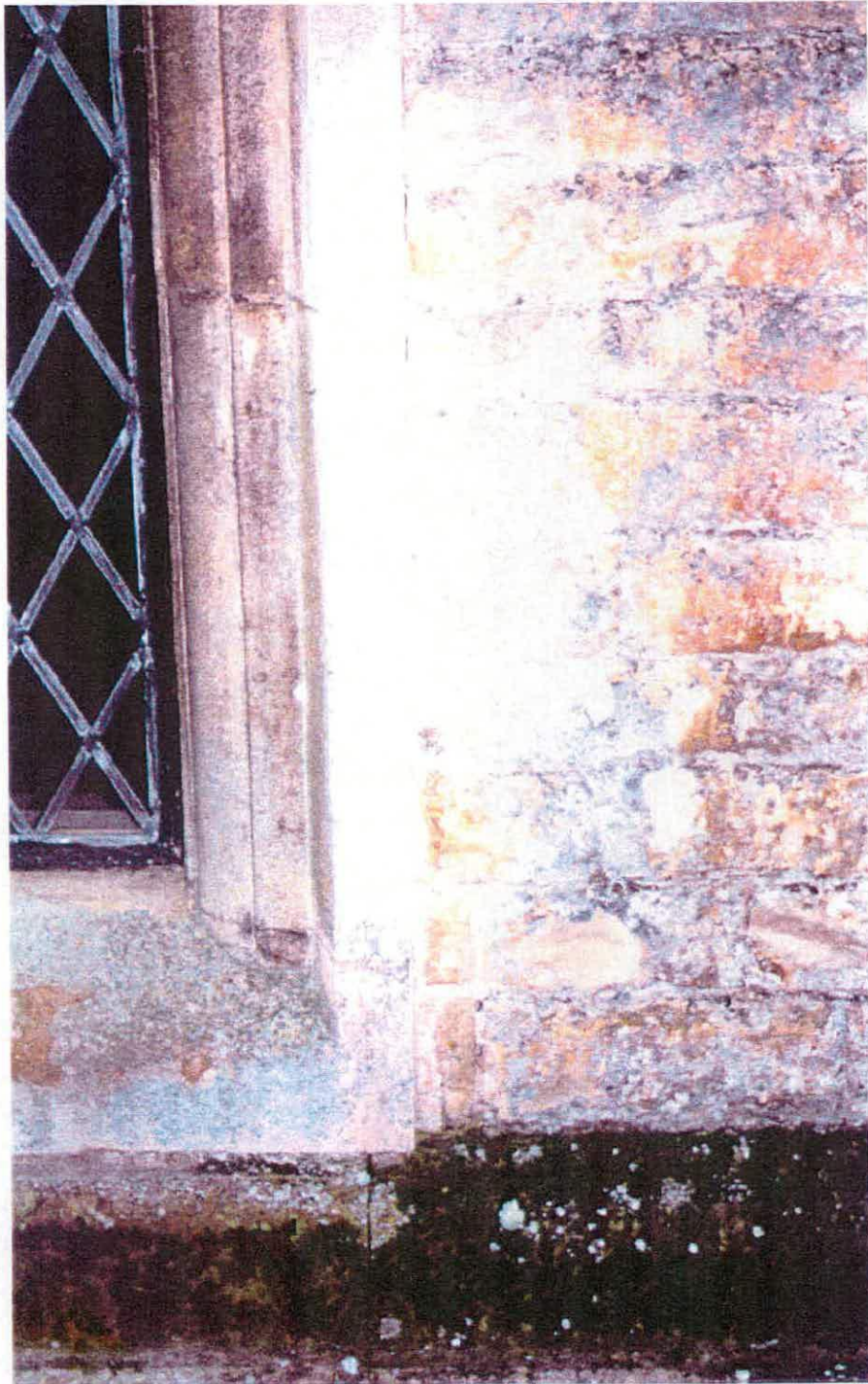
Fig. 38 Detail (of fig. 37) showing the lower right jamb of one of the windows at the northern end of the brewhouse east façade. Note the stones to the lower right of the jamb, cut to accommodate the extended window. Differences in mortar can also be observed.
