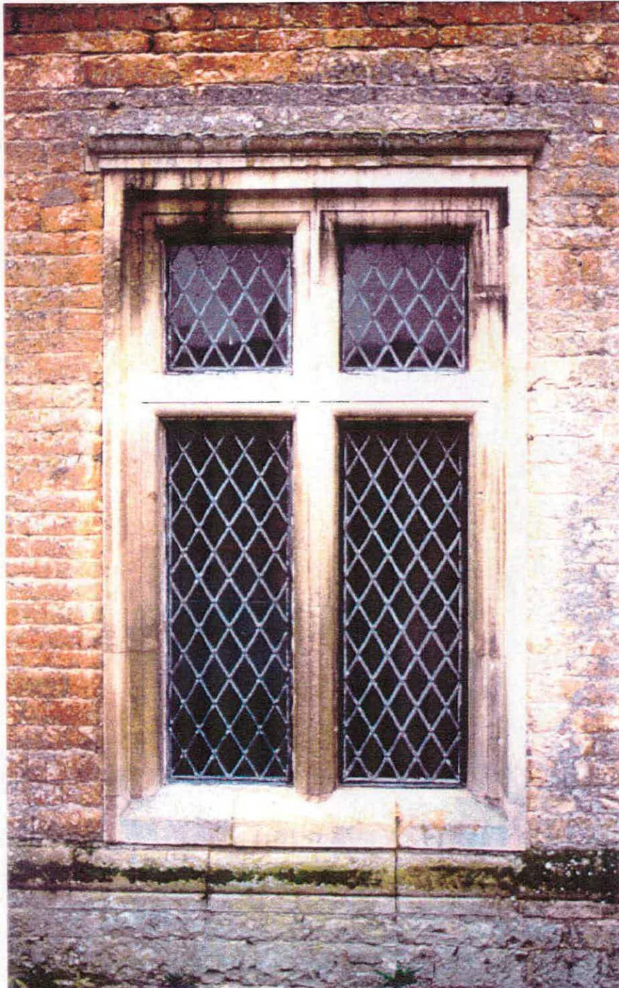
Fig. 37 One of the two extended windows at the northern end of the brewhouse east façade. The sill was lowered, and the transom introduced, as part of one of the secondary phases of work on the building.
