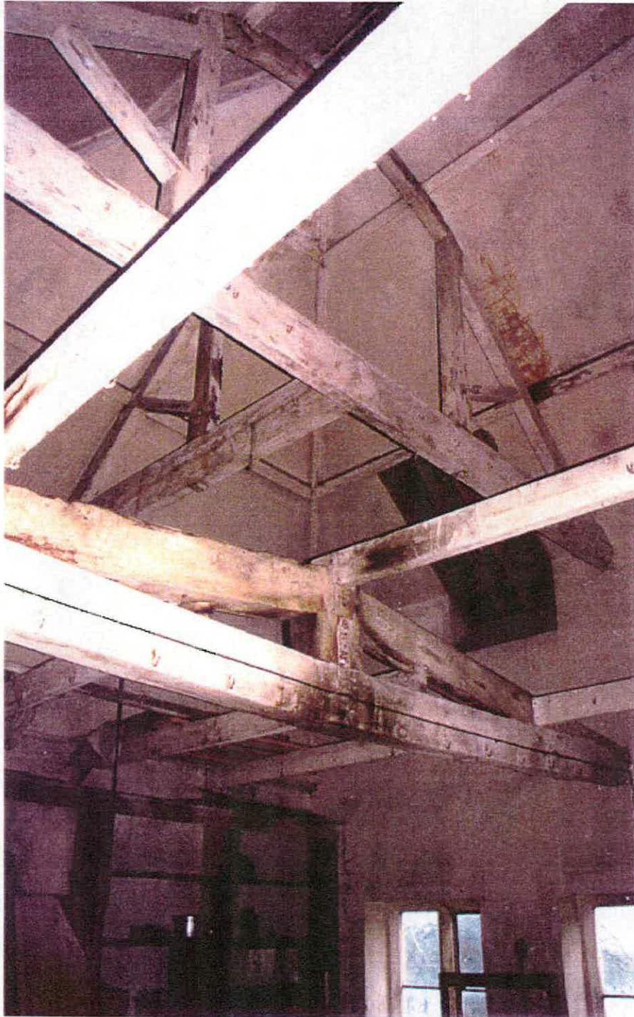
Fig. 33 Two of the trusses which supported the original roof over Brown's brewhouse range survive. They are of low pitch, with tie beams. This view shows the truss in the chamber over the 'Slaughter House'. The purlins are also original. Above is a truss of the later roof.
