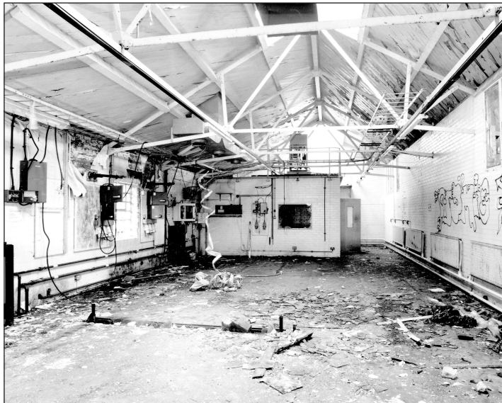
Figure 23 Interior of the radio station workshop incorporating the earlier 1903/1904 Shell and Cartridge stores (note the original steel roof structure) (AA00/1086)
