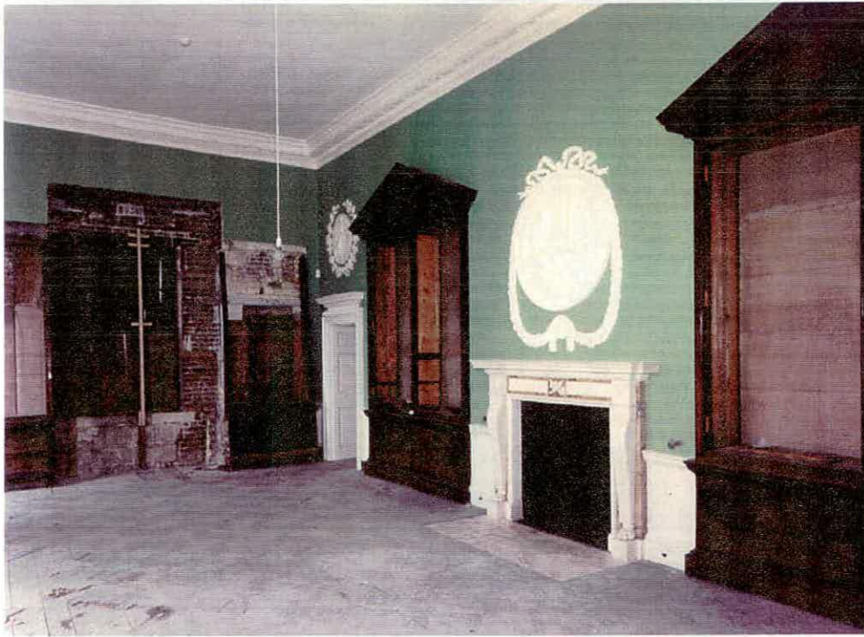
Figure 5, the Library in January 1998, after restoration of the plaster, with the two pedimented bookcases on the east wall in-situ and the two smaller bookcases against the north wall partially dismantled.
