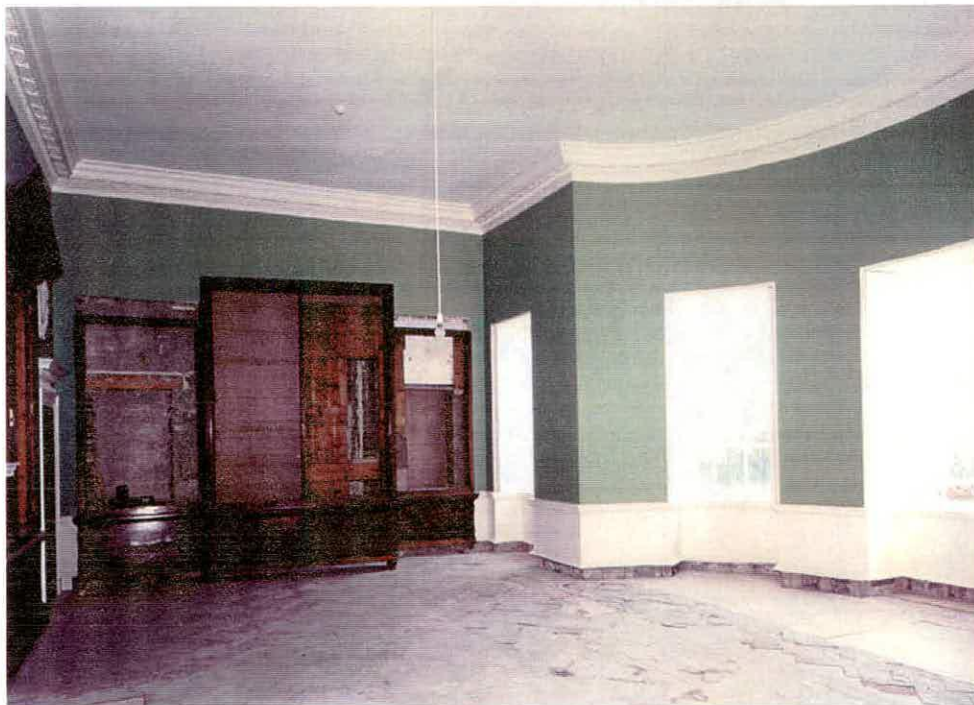
Figure 6, the Library, looking south in January 1998, after restoration of the plaster, with the three bookcases partially dismantled and only approximately placed in position.
