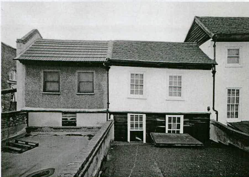
Fig. 6 - Nos 60 and 62 Peckham High Street, view from over shop extensions showing upper-storeys front in 1998 (RCHME, BB99/00124).
