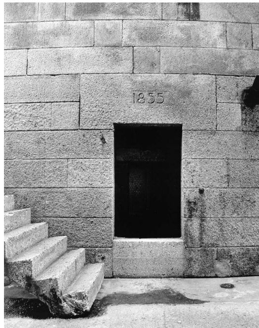
Figure 6 The original entrance into the Tower with the date of construction incised into the lintel (NMR: AA98/07903)
