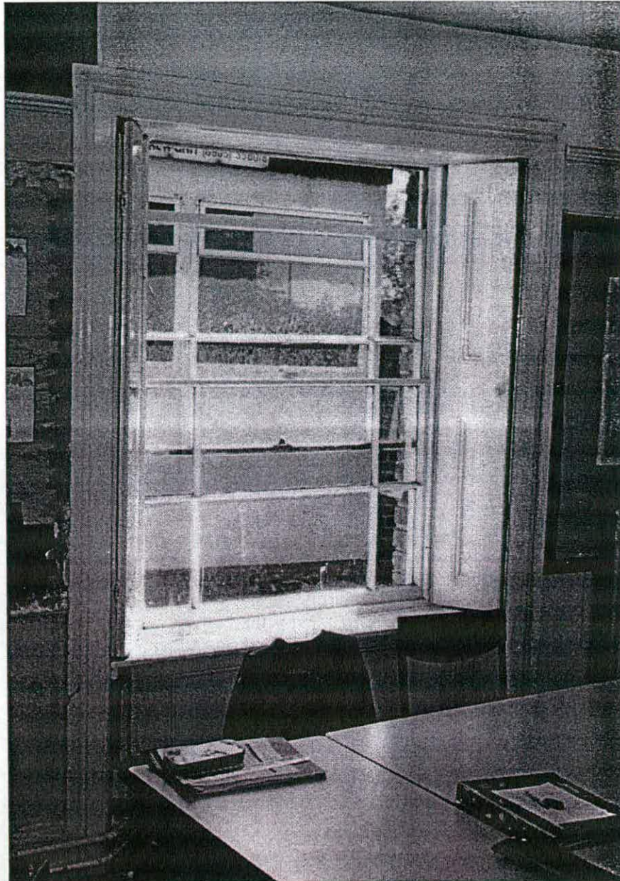
Internal elevation showing surviving shutters, sash boxes and margin-light, counterbalanced sashes to main ground floor, flank wall.
