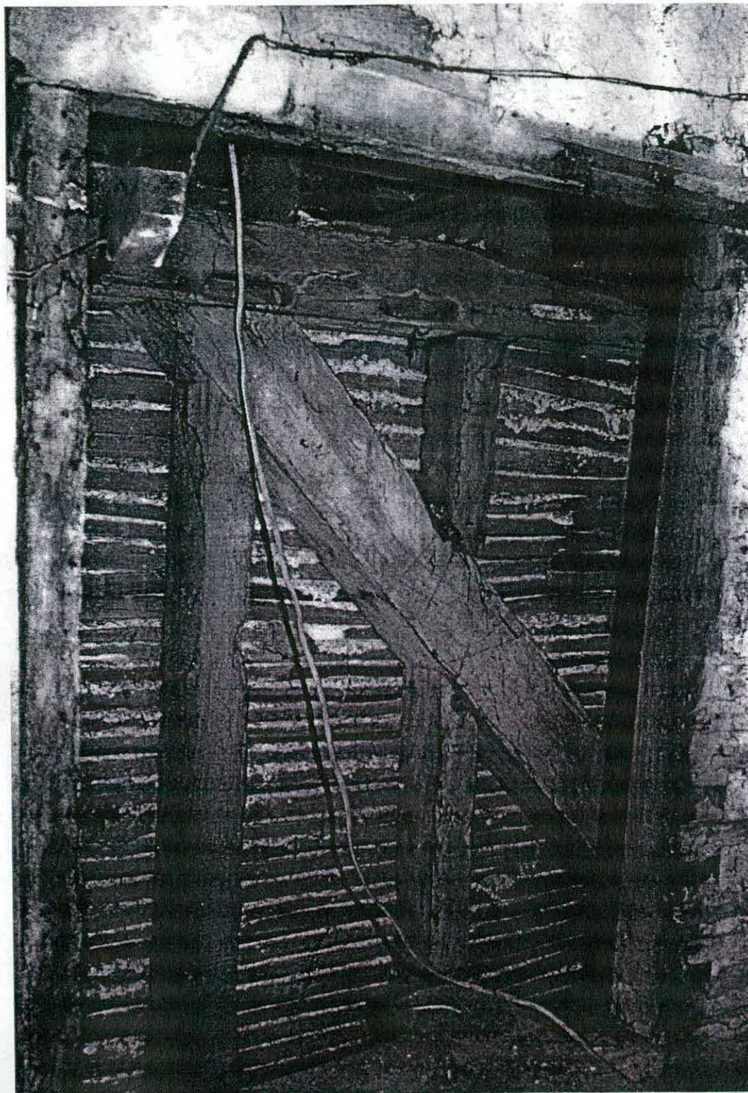
Constructional void between main front range and earlier 17C range showing braced framing and re-used timbers.
