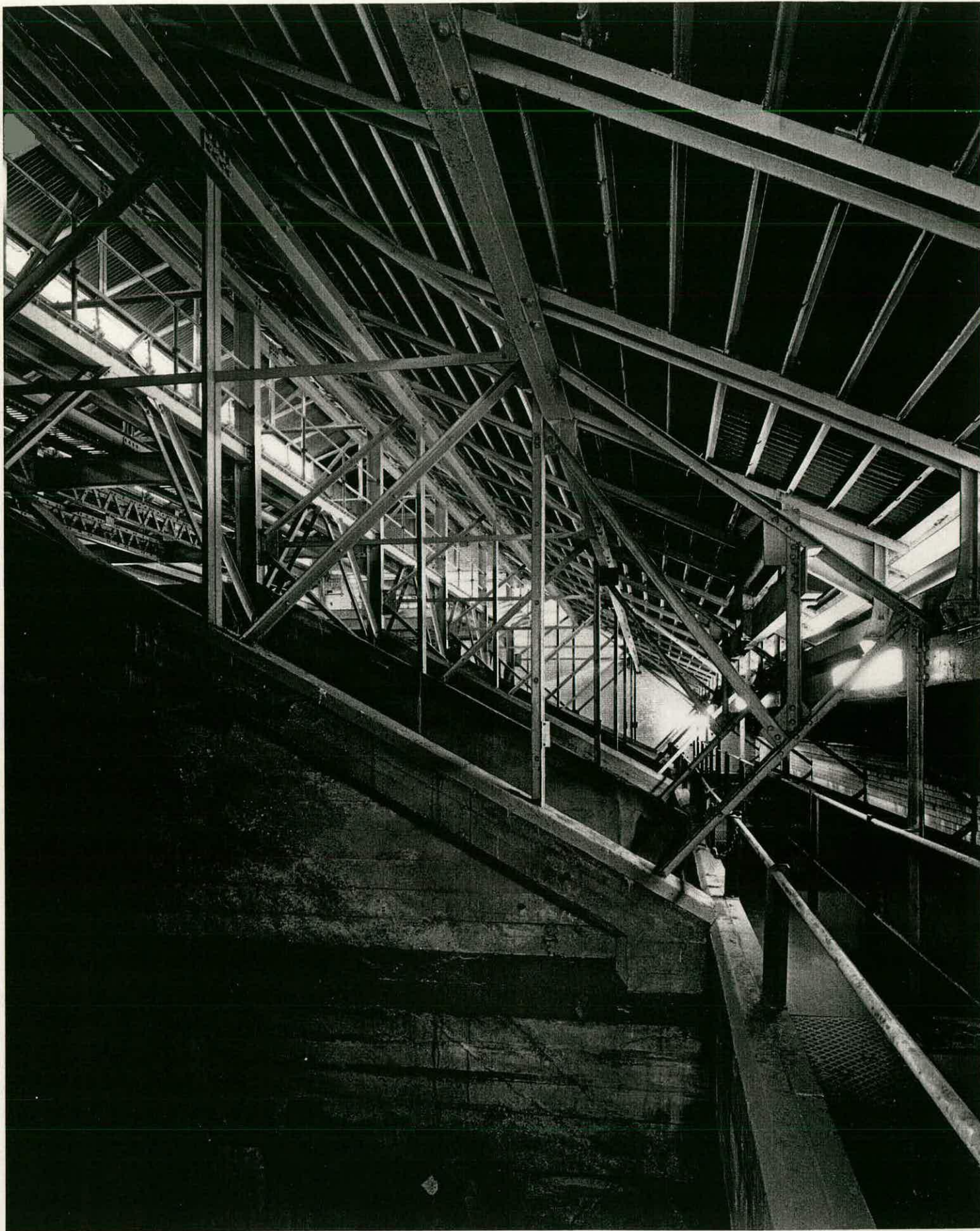
Greenwich Generating Station, view from within the former boiler house at roof level showing heads of coal bunkers (BB94/11451).
