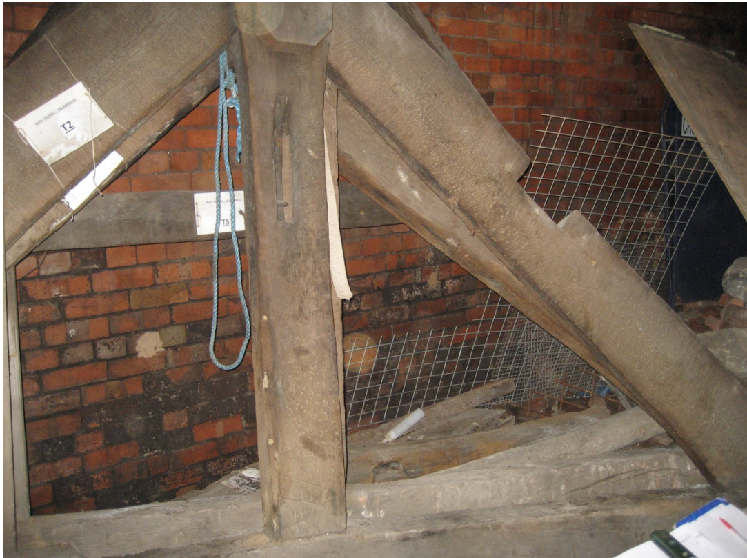
Figure 8: Trusses 2, 3, and 5 in storage with truss number labels still attached, truss 2 at the front, truss 5 against the wall at the back (photograph Cathy Tyers, Historic England)
