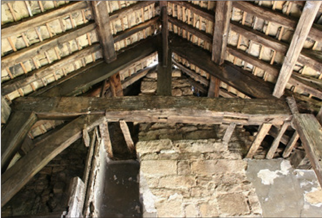
Fig 9: truss III, showing brace from post f, king-post truss and tie beam with mortices in soffit for brace to right and, centrally, for strut formerly down to bressumer (© Diane Charlton)
