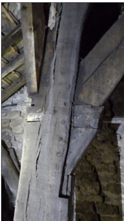
Fig 6: post f, west face, showing pegged joint for brace to tie beam and door lintel (©Historic England. Colum Giles)
