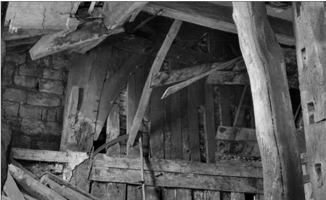
Fig 12: remains of the dais canopy, c.1956-7, photographed by Christopher Stell. Much of the plank boarding had been removed, but the head beam and some ribs remained, the latter pegged to the studs of truss IIII (©John Stell: Historic England Archive, STE01/01/005/04 (RB Card: 6672/35))
