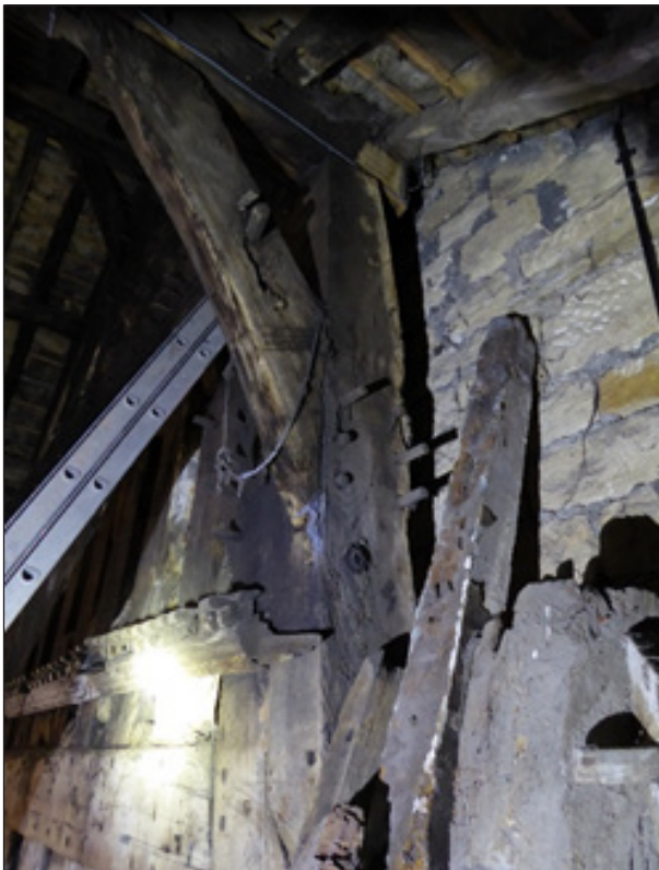
Fig 17: truss IIII, post h from north, showing brace up to arcade plate to east and pegged joint for similar brace (no longer in place) to west (©Historic England. Colum Giles)
