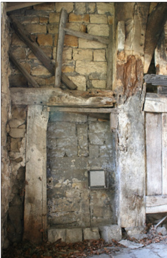
Fig 16: truss IIII, south aisle, showing aisle tie and doorpost for door to west: above the aisle tie are parts of the timber window recorded by Stell (© Diane Charlton)
