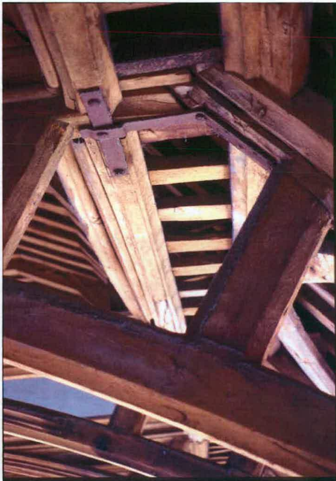
Fig. 23, a detail of the truss between the first and second bays at the west end of the Great Hall, viewed from the west. The iron strap repair may be contemporary with the insertion of the tie-beams in 1748. Photograph: March 1990.
