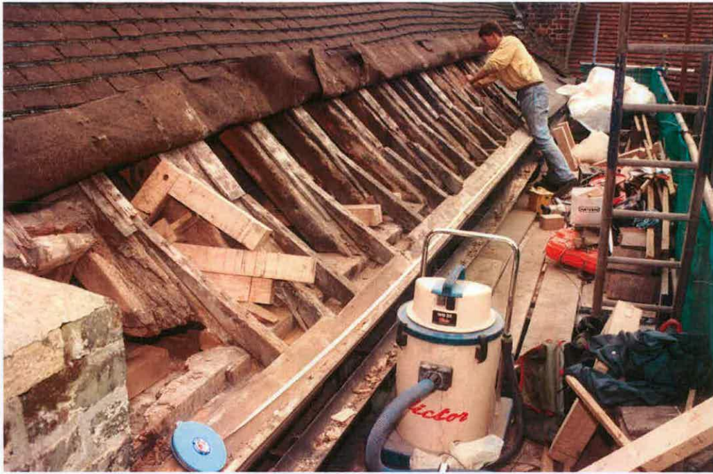
Fig. 39, the rafter ends above the north wall of the Guard Room. Photograph: October 1995
