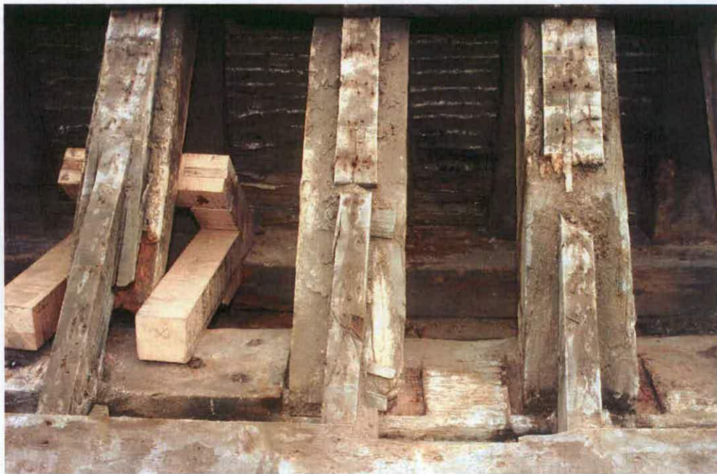
Fig. 40, rafter ends above the north wall of the Guard Room with one of the timber frames installed in 1995 to triangulate the rafters with the wall plates. Photograph: October 1995
