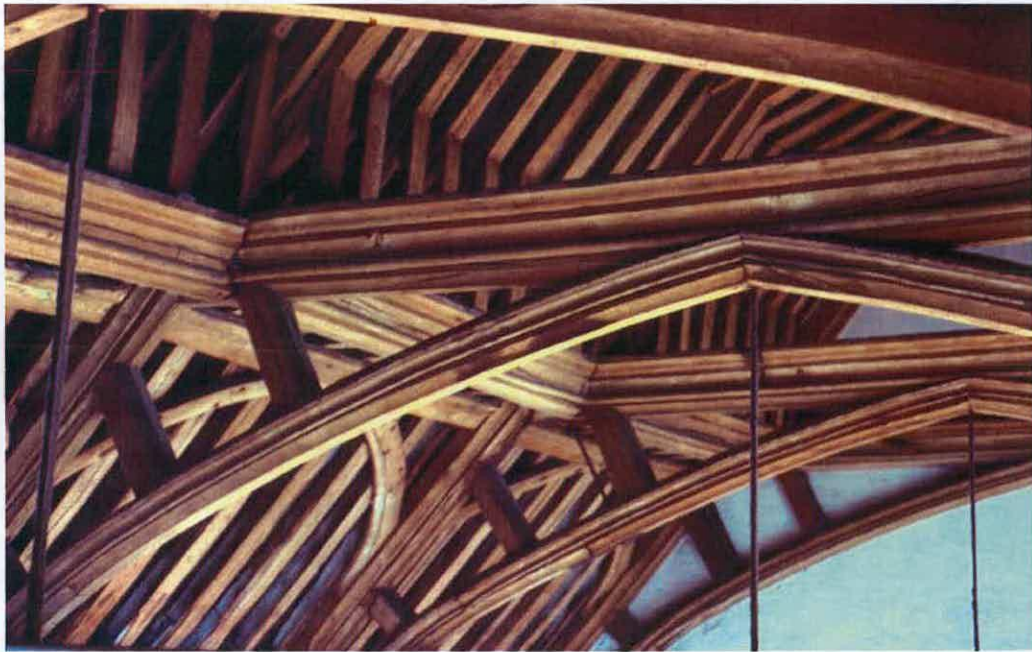
Fig. 22, a general view of the roof above the Great Hall from scaffolding erected against the west wall. Photograph: March 1990.
