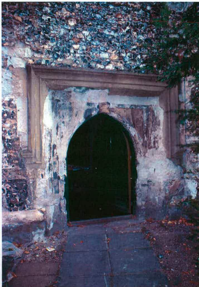
Fig. 34, the door at the east end of the south wall of the Great Hall. Photograph: August 1993.
