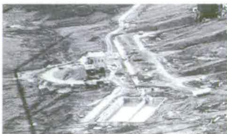
Figure 137 Aerial photograph taken in 1959 during the construction phase showing the position of the aggregate grader, looking west © Rolls-Royce plc
