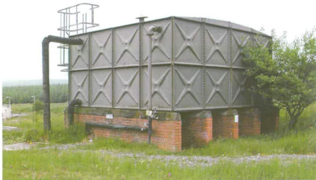
Figure 305 Braithwaite Water Tank containing the domestic supply for the Meteorological Station © English Heritage (AF00134/metstation water)
