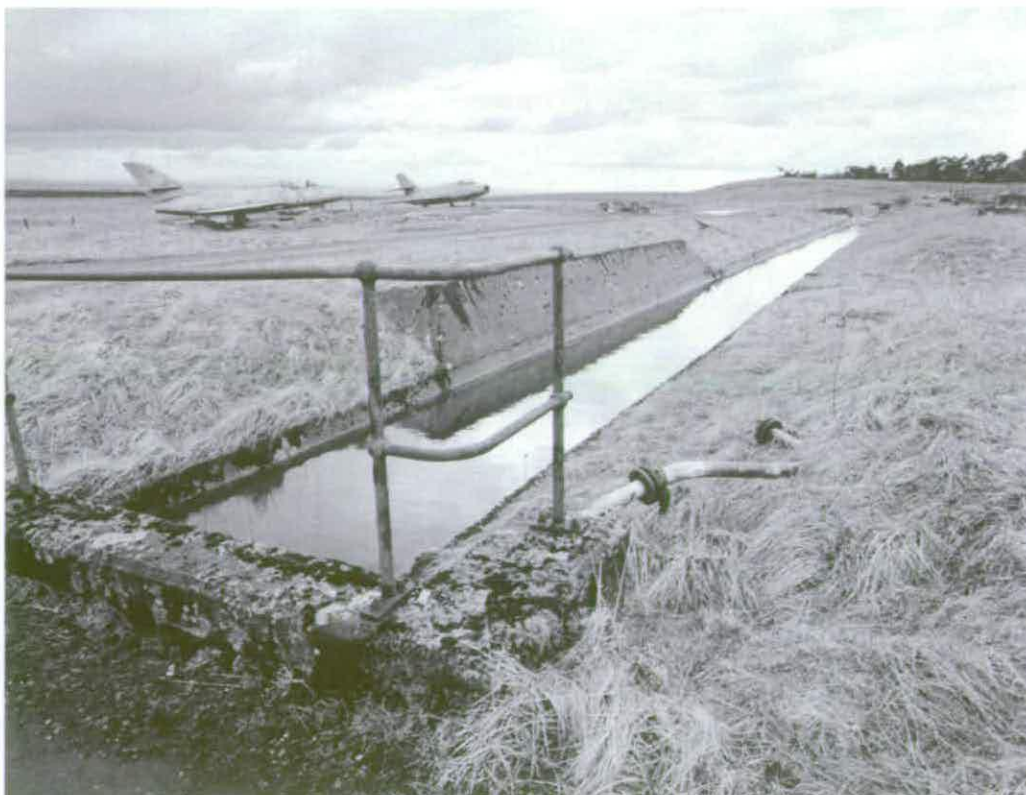
Figure 200 A concrete lined drain that flanks the south side of the test stands carried cooling water and unspent fuel to an Effluent Lagoon A14 © Crown copyright NMR (AA94/1968)
