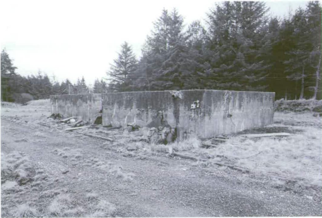
Figure 84 Cooling Tanks D7.1 and D7.2 now derelict, stand to the south of the main BOC Compound building © Crown copyright NMR (AA94/2910)
