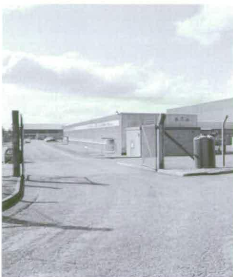
Figure 40 To the north of the Main Office Building F1.1 is a Sub-station F42.3 © Crown copyright NMR (AA94/1924)
