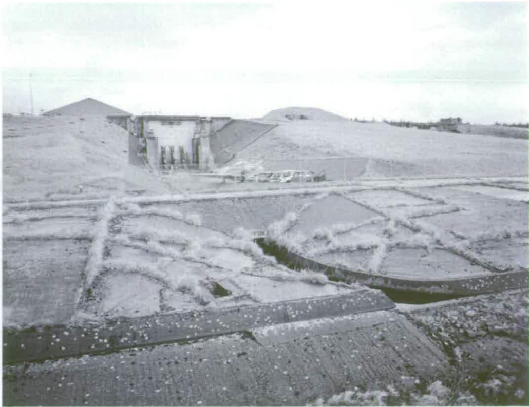
Figure 158 The concrete spillway of Engine Test Stand A2 drained into a conduit to the south © Crown copyright NMR (AA94/1961)
