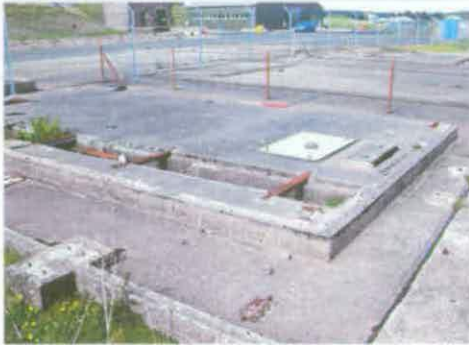
Figure 165 Concrete floor slab of the former Electrical Control Station A17.3 © English Heritage (AF00134/A17.3)
