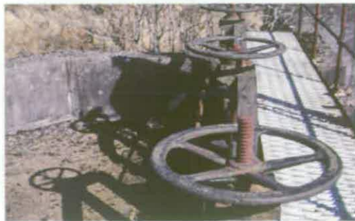
Figure 122 A series of four metal sluice gates controlled the flow of effluent from the main channel into the Settling Tank B6 © English Heritage (AF00134/B6 sluice)
