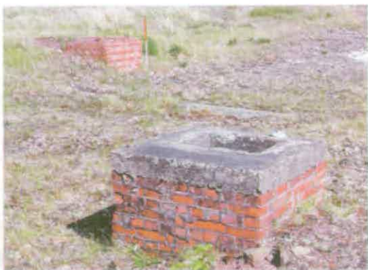
Figure 25 A series of brick drains survive on the site of the former labourers' huts © English Heritage (AF00134/paddy2)
