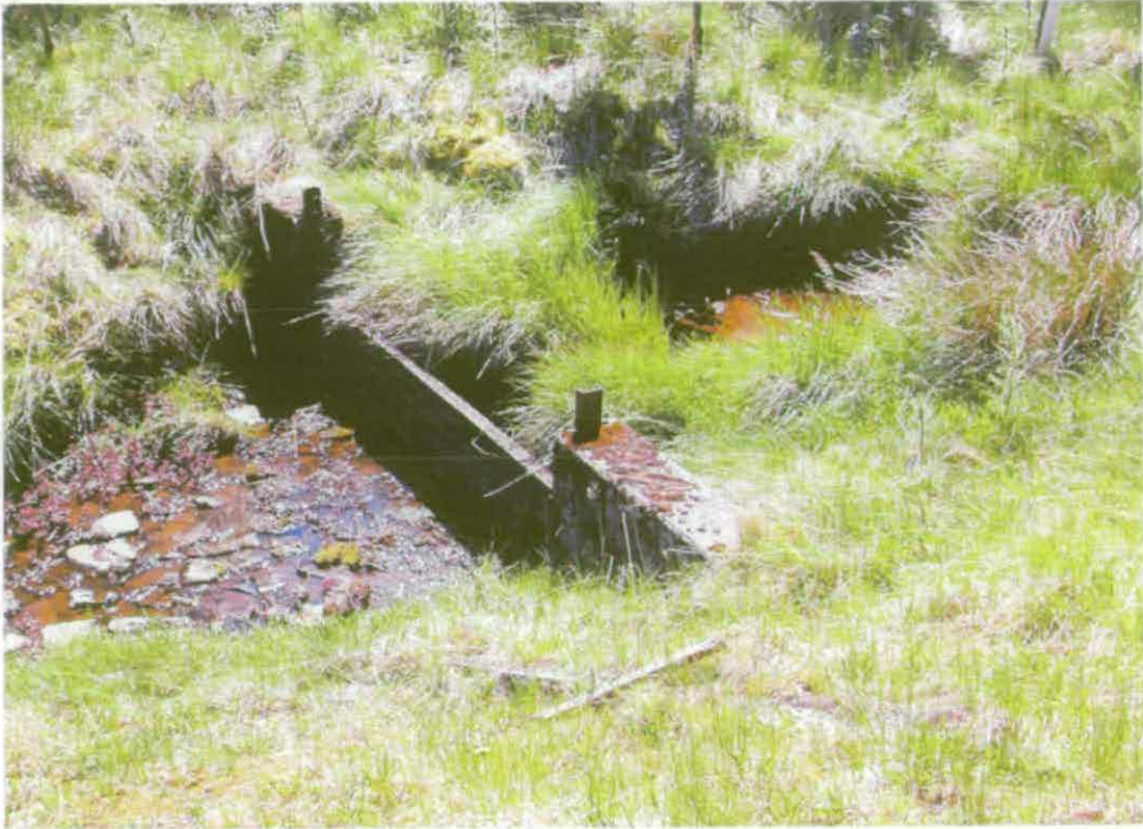
Figure 279 A sluice gate controlled the flow of stream water into the silo hole © English Heritage (AF00134/launcher silo2)
