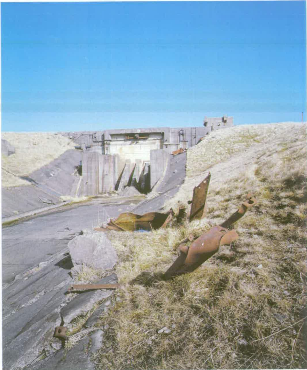
Figure 21 Test Stand A1 at Priorlancy Rigg was used in the late 1970s for destructive pipeline testing by the British Gas Council © Crown copyright NMR (AA94/2954)
