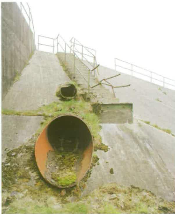
Figure 154 Large bore steel pipes on the east side of Engine Test Stand A2 poured vast quantities of cooling water onto the hot steel deflector bucket to prevent it from melting during test firings © English Heritage NMR (DP003884)
