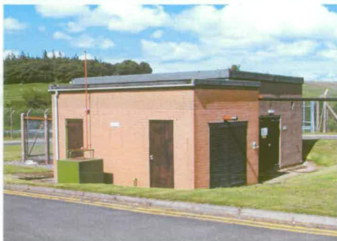
Figure 56 Midshield Sub-station F42.1 © English Heritage (AF00134/F42.1)
