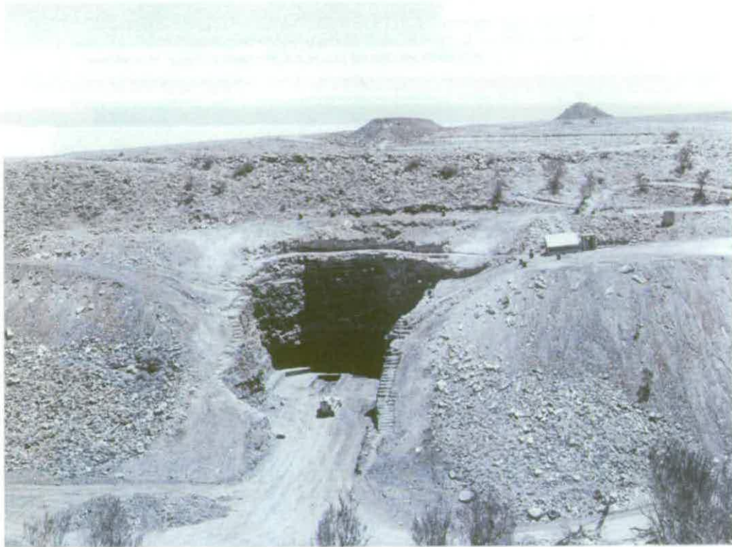
Figure 281 Excavations at Woomera, Australia for an Underground Launcher Facility © Weapons Research Establishment, Salisbury, Australia
