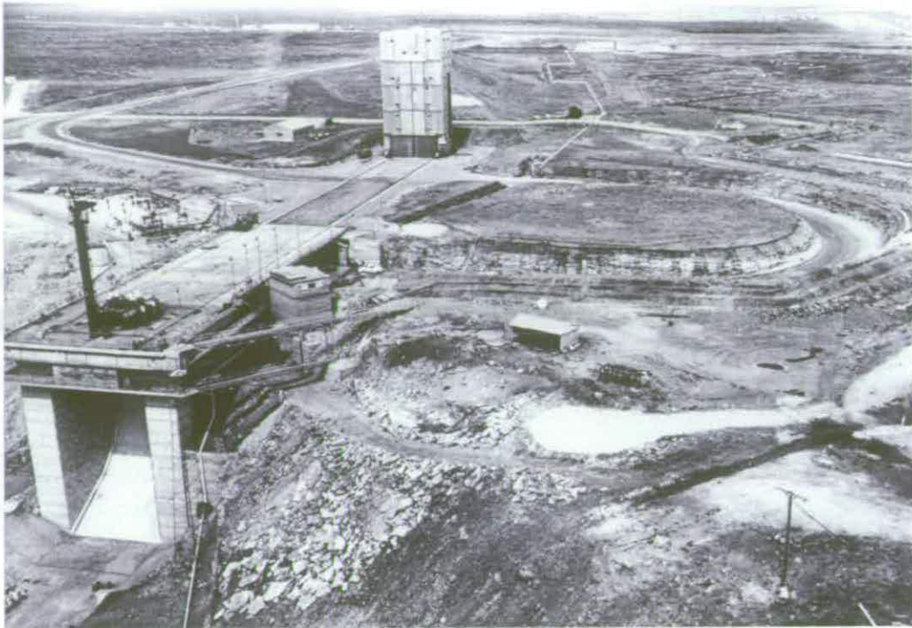
Figure 9 Construction of the test stand at Woomera, Australia © Weapons Research Establishment, Salisbury, Australia
