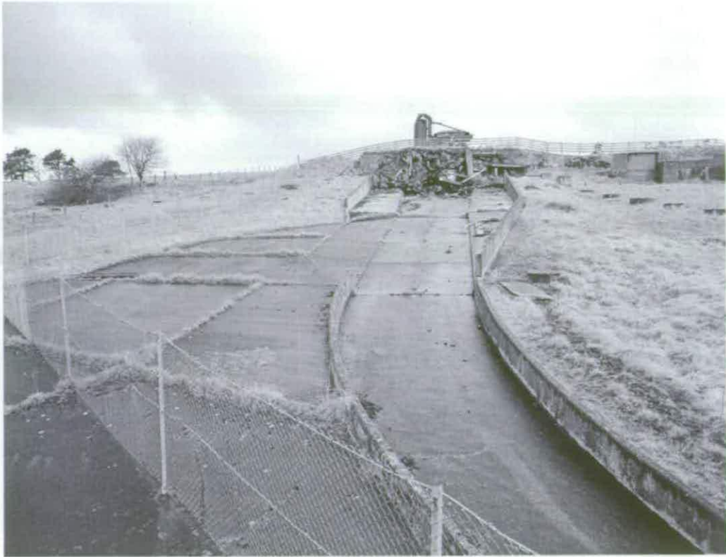
Figure 171 Derelict concrete spillway of Engine Test Stand A42 © Crown copyright NMR (AA94/2925)
