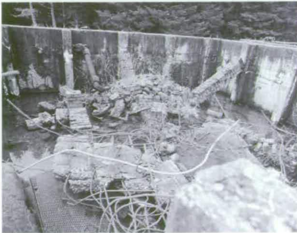
Figure 85 Interior of derelict Cooling Tanks D7.1 and D7.2 © Crown copyright NMR (AA94/2911)
