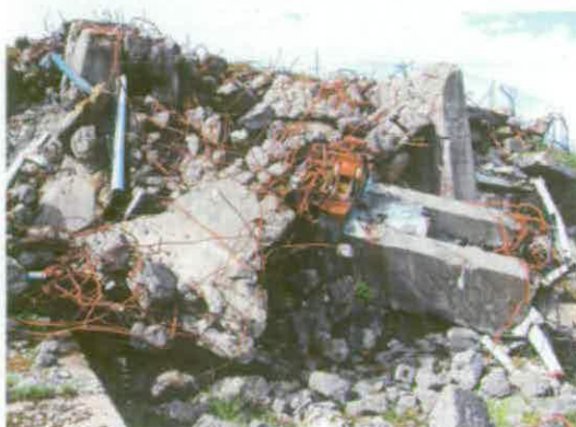
Figure 174 Engine Test Stand A42 was demolished with explosives after being decommissioned © English Heritage (AF00134/A42)
