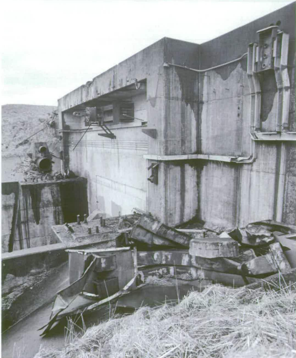
Figure 139 Rear wall of Engine Test Stand A1 with a gimballed mounting for the efflux deflector still in place © Crown copyright NMR (AA94/1957)
