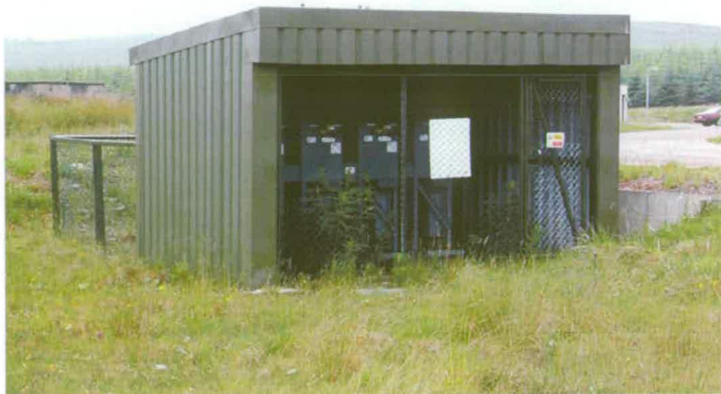
Figure 304 Transformer Station L4 at the Meteorological Station © English Heritage (AF00134/L4)
