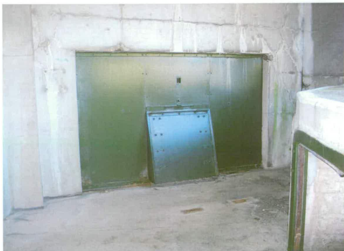
Figure 30 Photo of the self-closing door at the top of the ammunition hoist for no 2 twin 6-pdr QF gun. The ammunition handling area is in the foreground, the gun floor loading platform to the right (Paul Pattison)
