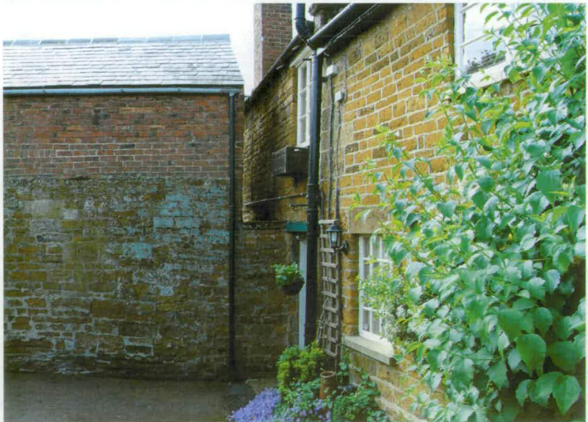
Figure 8 – The awkward junction between 53 Main Street (left) and the earlier houses (right)
