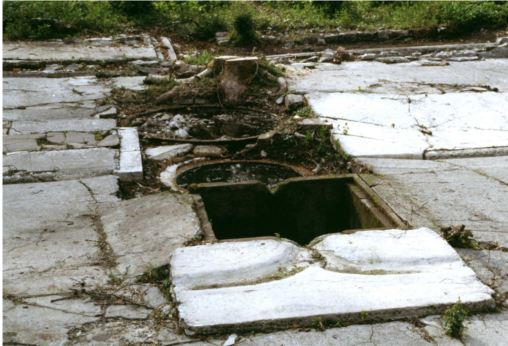
Figure 15. The tank and cast - iron basins in the floor of the saltpetre refinery, from the south east. (NMR: DP001578, reproduced by permission of Christopher Dunn)
