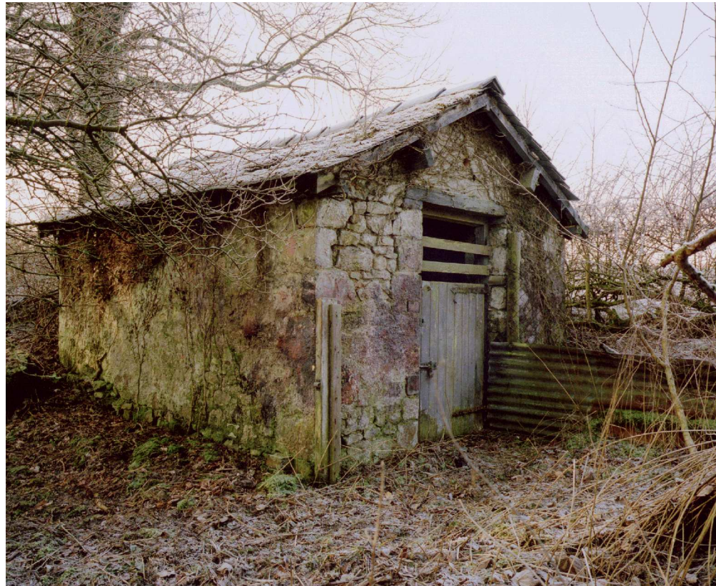
Figure 48. The small stable to the west of the cooperage, from the north east. (NMR:AA012847)
