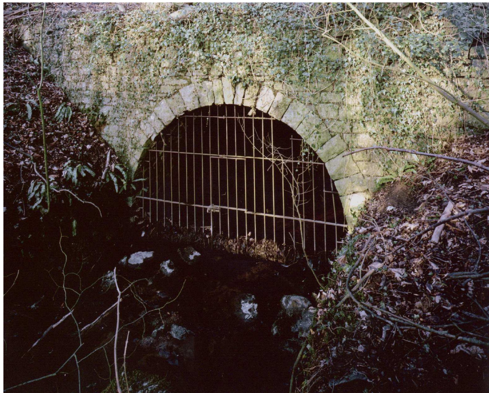
Figure 13. The arched exit of the main tailrace from the south east. (NMR: AA012903)
