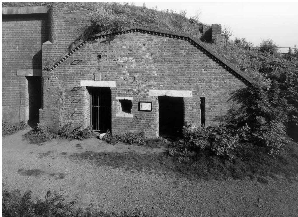
Figure 11 St Martin's Battery: doors to lamp store (at right) and shell store A, with lamp recess between (NMR: AA 99 09711 © Crown Copyright 1998)
