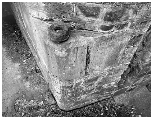
Figure 10 St Martin's Battery: lower davit socket in emplacement no II (extract from NMR: AA 99 09719 © Crown Copyright 1998)
