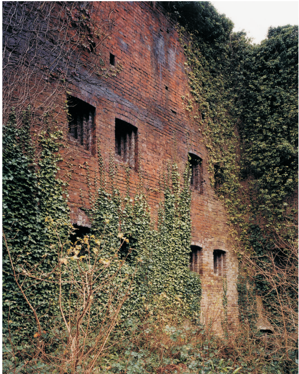
Figure 35 Detached Bastion; musket loopholes of the north musketry gallery, seen from the north ditch of the bastion (NMR: BB 029678 © English Heritage 2001)
