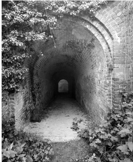
Figure 25 Detached Bastion; photo of the southern entrance to the west musketry gallery from the terreplein, showing the typical entrance arch and, centre right, a pintle hinge for the door, in its stone anchor block (NMR: AA008628 © Crown Copyright 1998)
