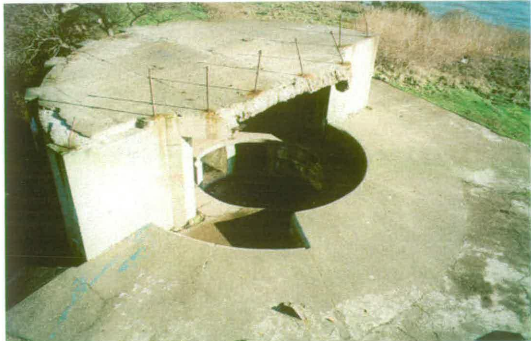
Figure 13 Photograph showing the southern 6-inch Mark VII gun emplacement with Second World War casemate over
