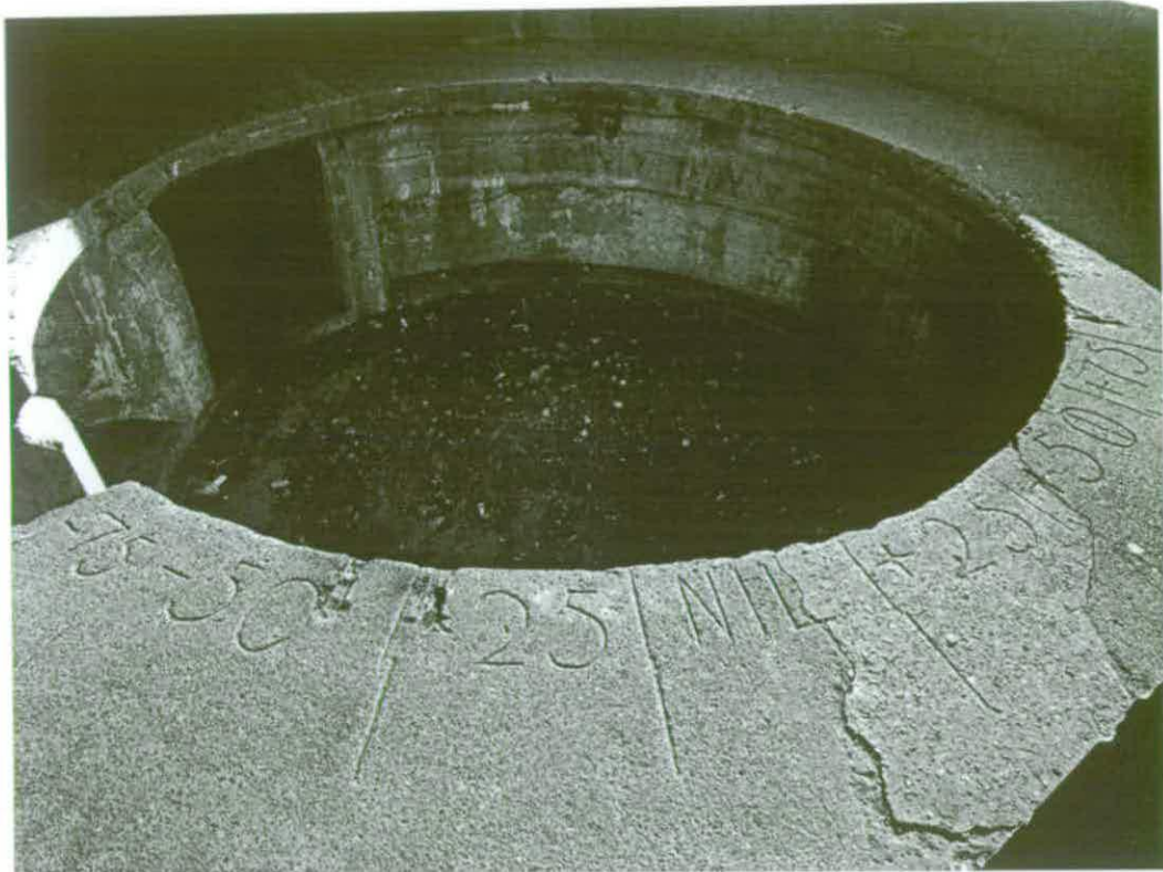
Figure 15 Photograph showing detail of the gun quadrant arcs for the southern 6-inch Mark VII gun (NMR: BB97/5388)
