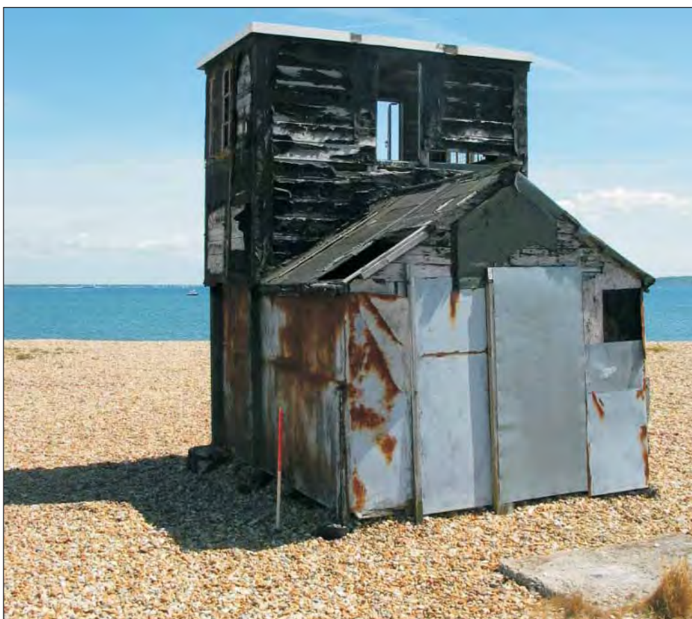
Plate B12: WA2059 . Former coastguard hut, possibly reused as a store shed
