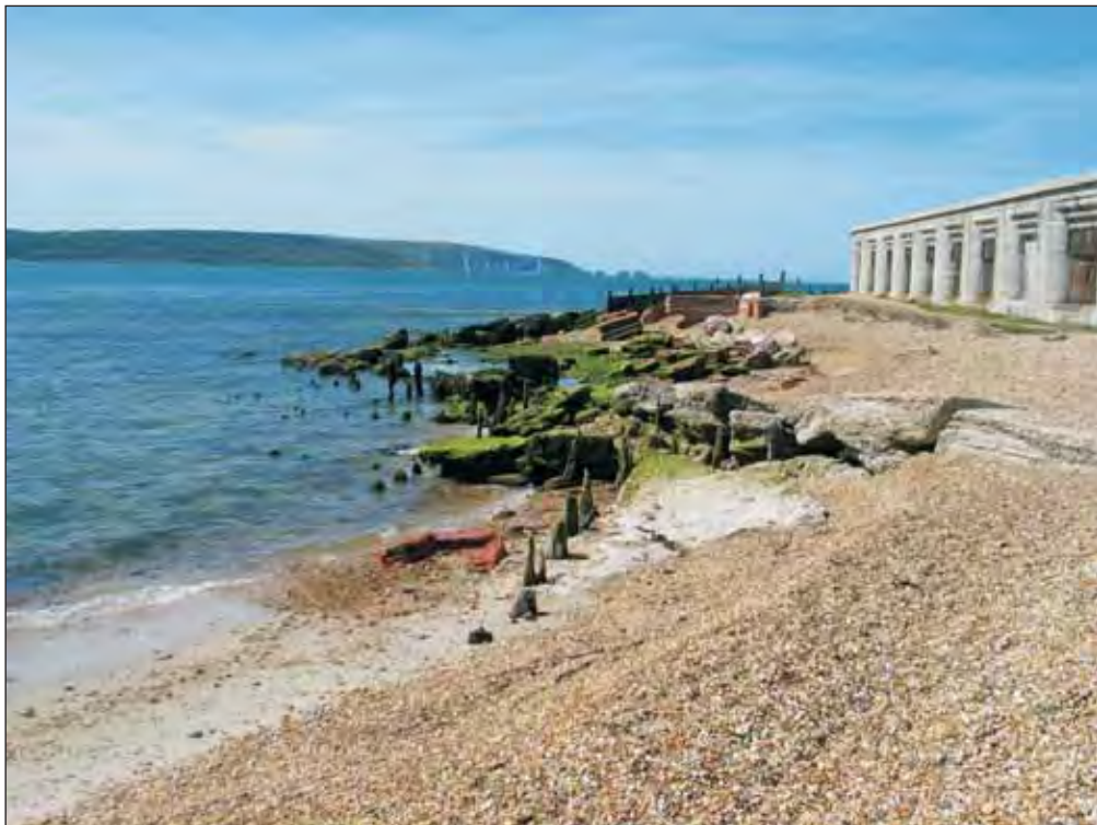
Plate B8: WA2051 . An array of wooden and concrete former sea defences, to the seaward of Hurst Castle
