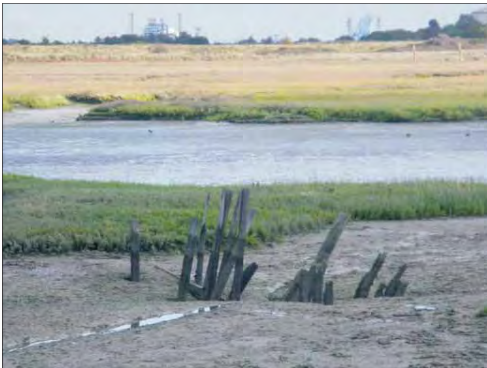
Plate E9: WA5033 . Remains of a timber revetment or sluice at Cadland Creek, besides a large outflow pipe from the adjacent refinery. The structure contains approximately 20 sunken posts
