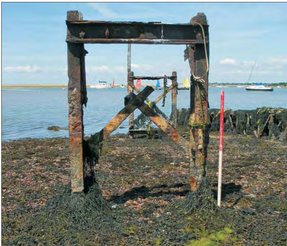
Plate B10: WA2056 . Wooden and metallic remains of large former jetty or landing pontoon, the north of the castle on Hurst Spit
