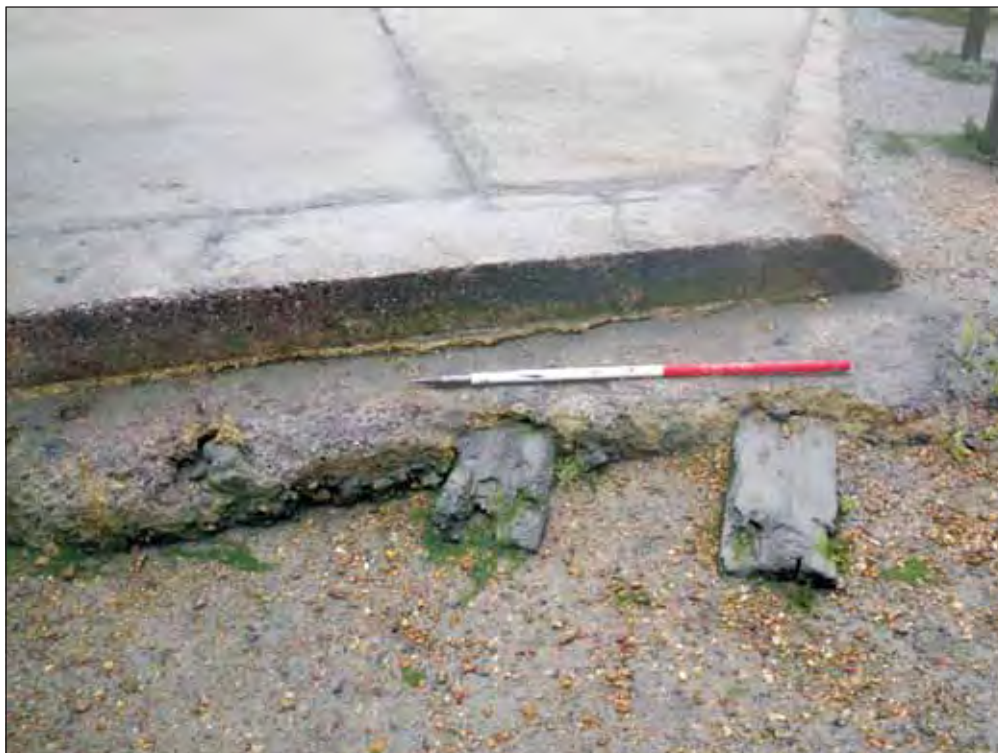
Plate E12: WA5031 . Three wooden beams protruding from underneath two phases of modern concrete, possibly part of Victoria Quay at Ashlett
