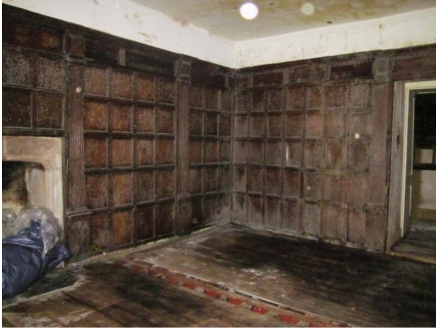
Figure 5a: View of the panelling to the Queen's Bedroom before removal for conservation (photograph Alan Lamb)
