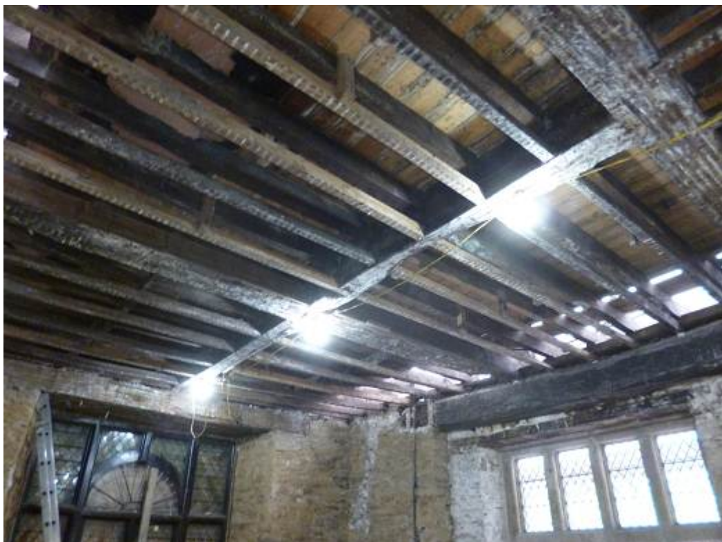
Figure 2c/d: Views showing the extent of the fire to the lower floors (photographs Robert Howard)
