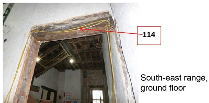
Figure 10o-r: Annotated photographs to help locate the sampled timbers (photographs Robert Howard)
