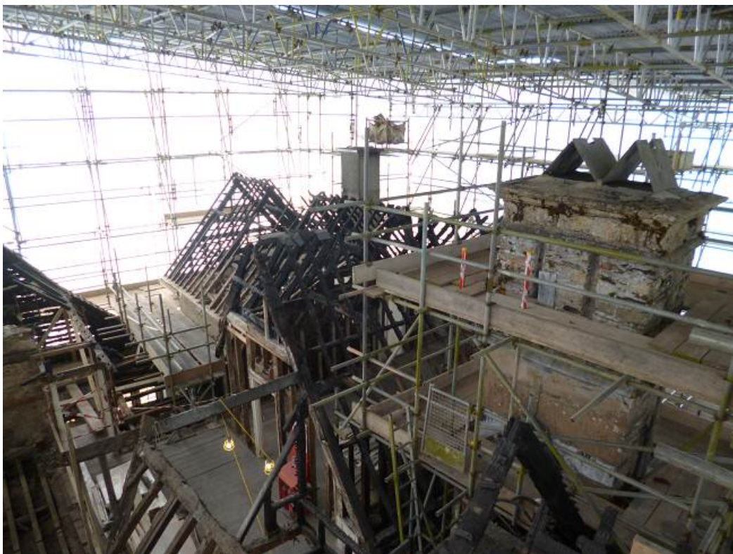
Figure 2a/b: Views showing the extent of the fire to the roofs (photographs Robert Howard)
